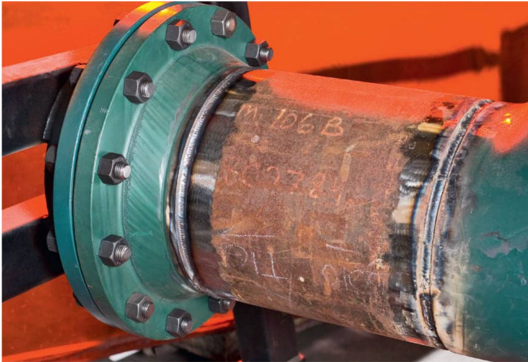
The first welds, called root passes, were made on this pipe using two different processes: TIG on the right and stick on the left.
