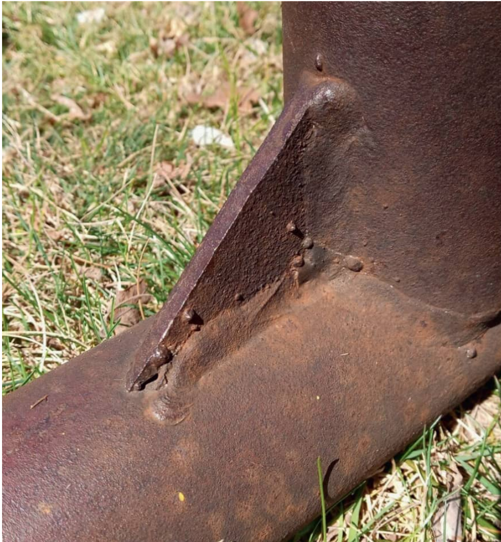
Weld is missing from the end of this triangular gusset. Wrap welds around corners to reduce the chances of cracking or tearing.
