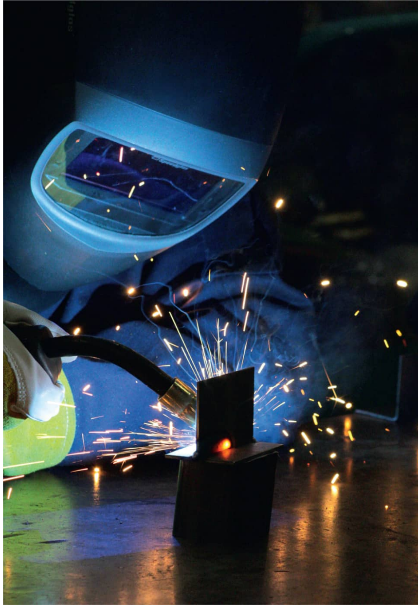
Seeing sheet metal glow orange on the back side of a weld is a good indication that you are using enough heat.
