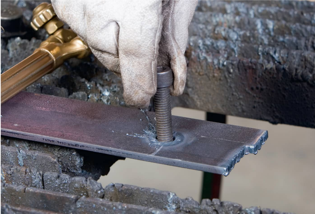
Torch cutting this hole for a bolt took much less time than drilling would have.
