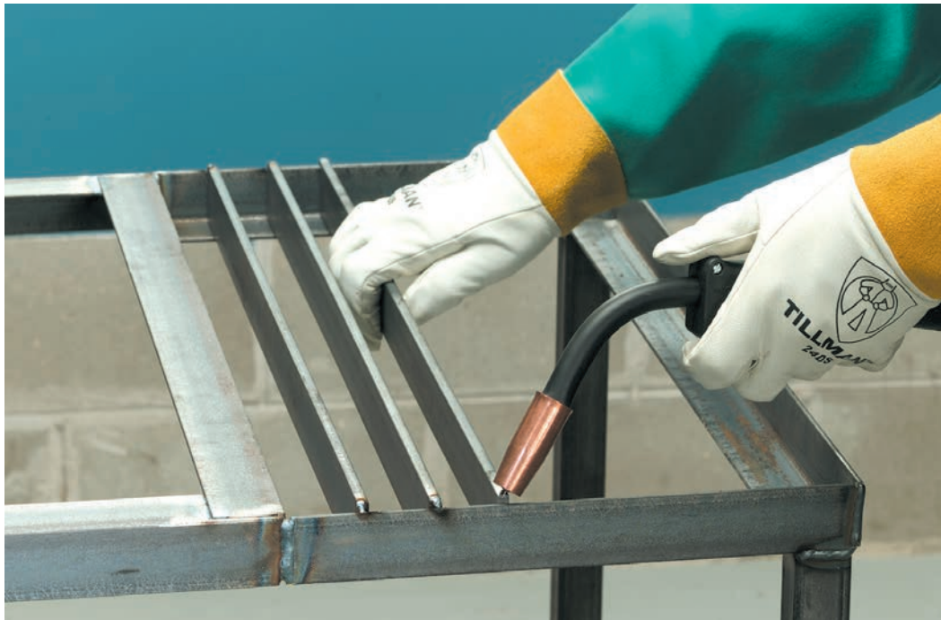
Tack weld cutting table slats to the angle iron every 1½" to form the cutting tabletop.
