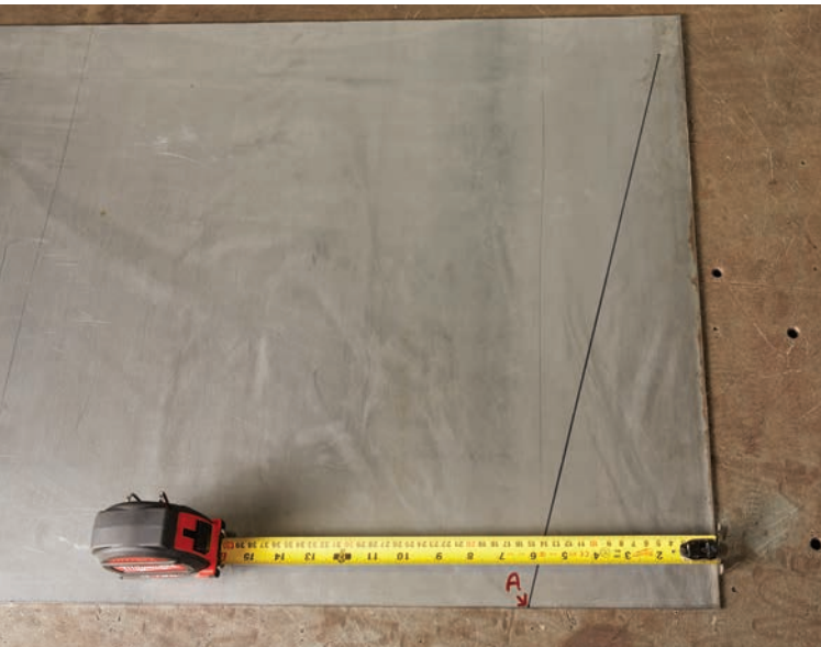
From point A, scribe a line at 75^\circ up toward the top outside corner.
