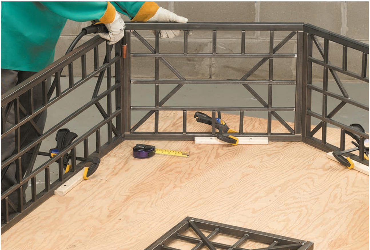
Place tack welds along the joint between the roof and side panels.
