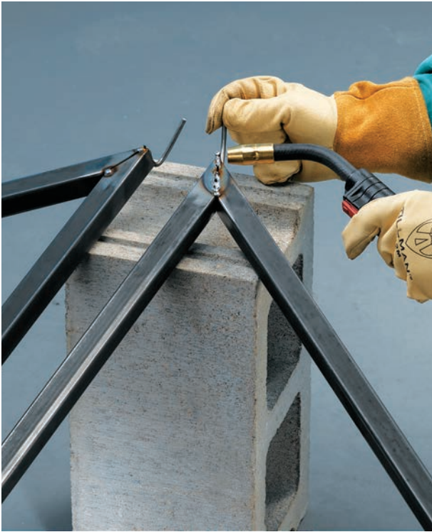
Support roof sections on a cinder block. Weld the finial pegs to the points of the panels.
