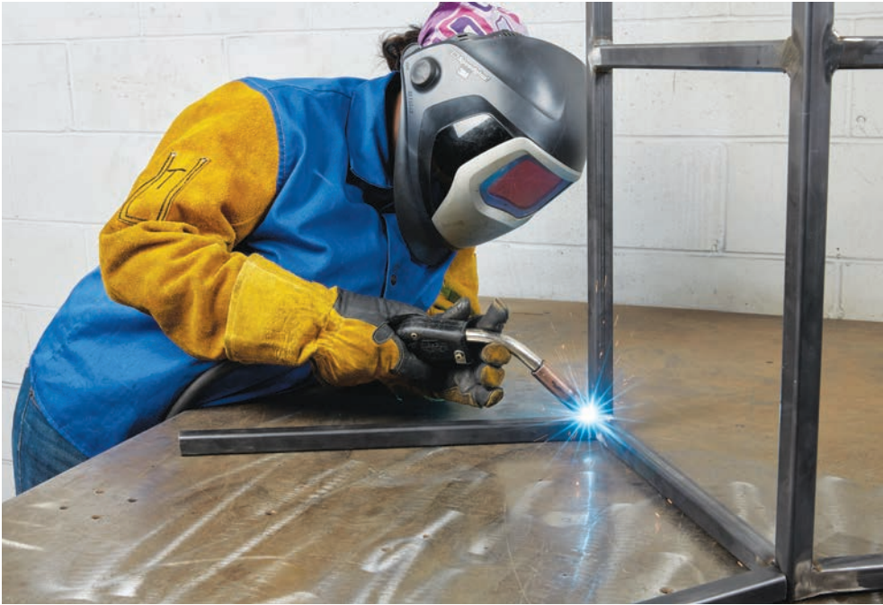
Align and tack weld one leg to each corner of the frame.
