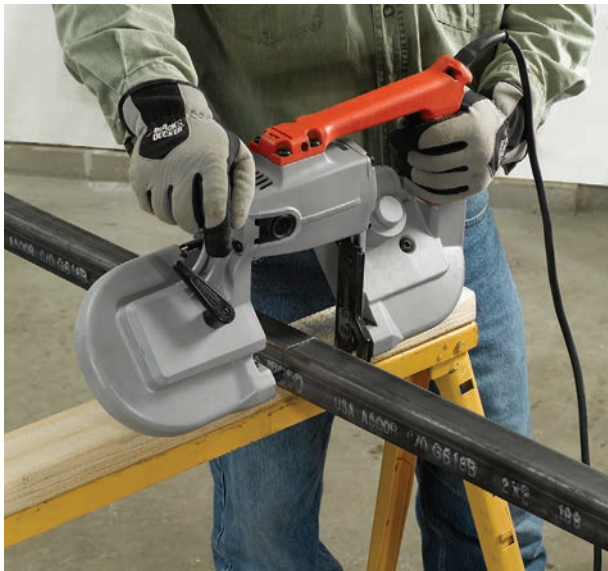
Cut the square tube using a metal-cutting bandsaw (shown) or cut-off saw with a hardened carbide blade.
