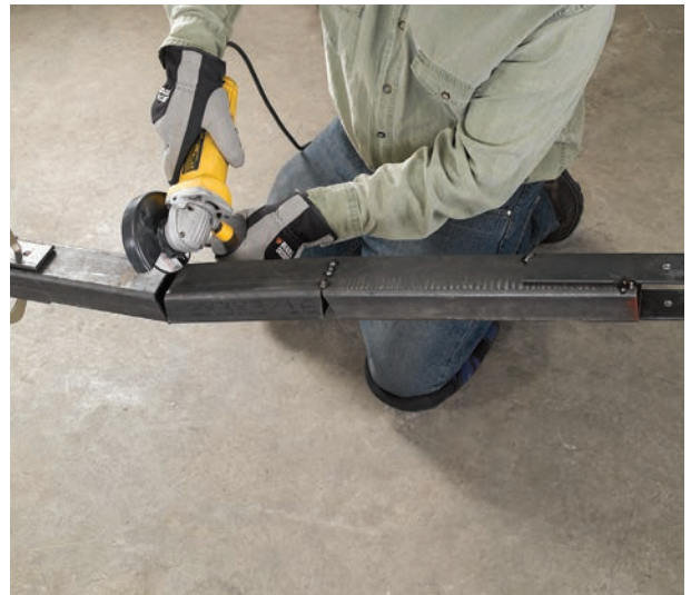
Score notches along the tongue to achieve the desired angle using a handheld grinder. Tack the bends and then hook up the trailer to your towing vehicle—the trailer should be level. If necessary, break tacks and re-bend tongue. Make final welds along each bend.
