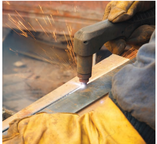
Making detail cuts is easy with a plasma cutter. Here the welder is cutting scrap metal for recycling.
