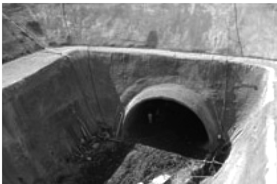
Figure 3.3 Portal with Wing walls in soft ground- Pir Panjal Tunnel North Portal.
