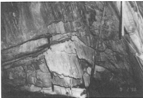
Figure 2: Stress induced fracturing and dilated joints above the backs of a recent ore drive, 410 Level.
