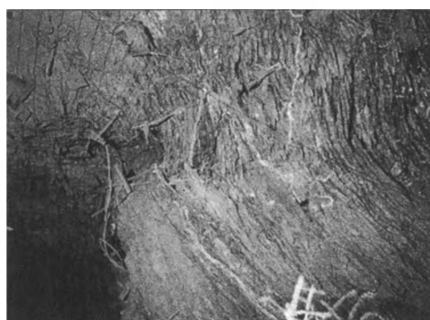
Figure 2. Buckling of rock mass after rehabilitation.
