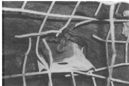
Figure 4: Severe damage caused to cable bolt surface fixtures by large deformations.
