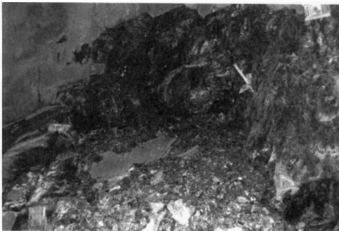
Figure 1. Unravelling in sheared ultramafic. Unreinforced shotcrete has been ineffective in controlling the failure.
