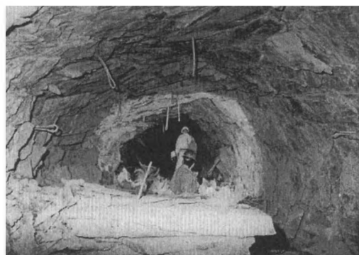
Photograph 6. Rock mass unravelling between rock bolts (background) and rock bolt failure (foreground).
