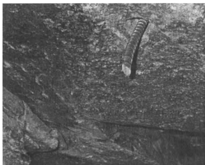
Photograph 4. Guillotining of hangingwall rock bolt.
