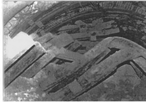
Figure 10. Floor heave of the main air roadway in soft rocks in Xieqiao Colliery, Anhui Province.
