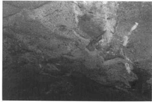
Figure 4. Detachment of unreinforced shotcrete, due to ongoing deformation.
