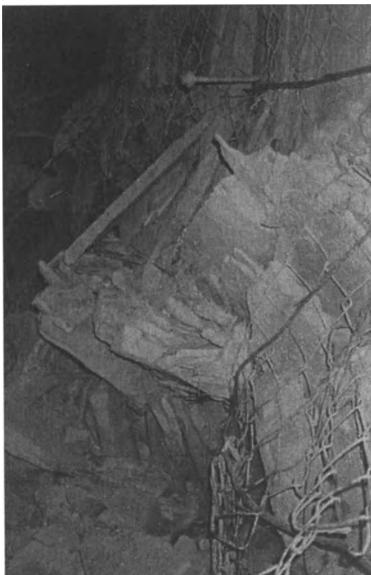
Photograph 1. Failure of mesh panel.
