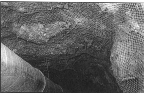
Figure 6 b. Wire mesh containing large volumes of unravelled rock at Hartebeestfontein site.
