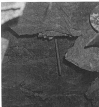
Photograph 5. Tensile failure of hangingwall rock bolt.
