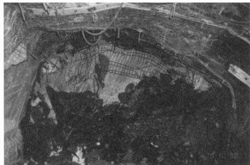
Figure 7: Multiple support phases at Site 1, cable bolts, gewi bolts and straps
