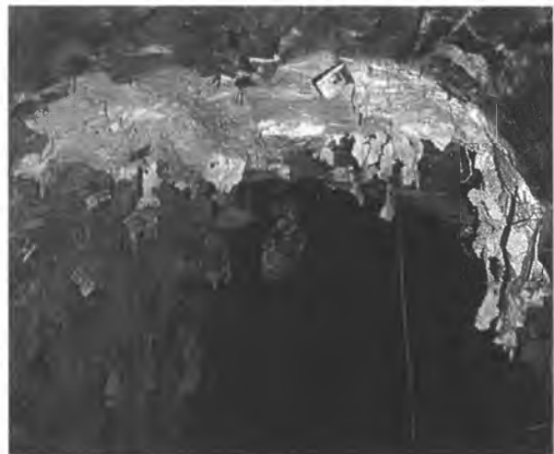
Figure 3. Damage to the Mineguard membrane along the brow following a stope firing.
