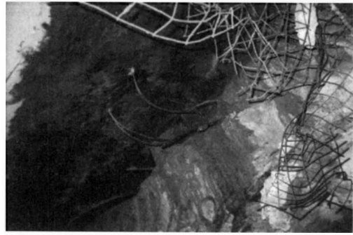
Figure 8. Cables installed through the footwall contact shear that have undergone more than a metre of shear (view looking up dip).
