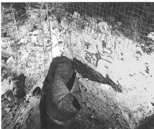
Figure 2. Peeling of the Mineguard membrane along the hangingwall and in the backs.
