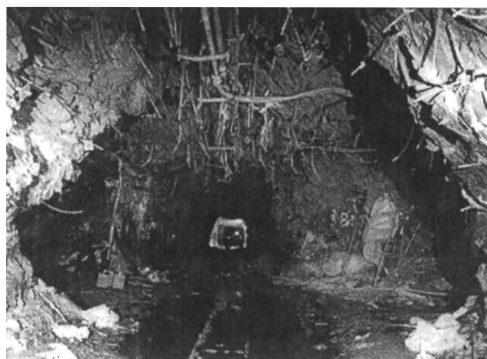
Figure 1. The unravelled walls and backs after re-bolting at 18B FWDR.
