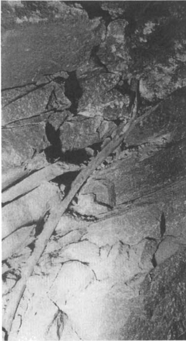
Photograph 7. Shear deformation of smooth bar rock bolt.
