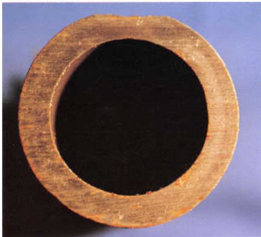
Figure 10.5 Transverse profile of tube showing metal loss.
