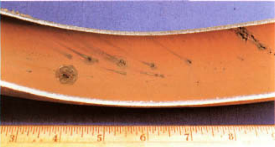
Figure 8.5 Oxygen pits on internal surface.
