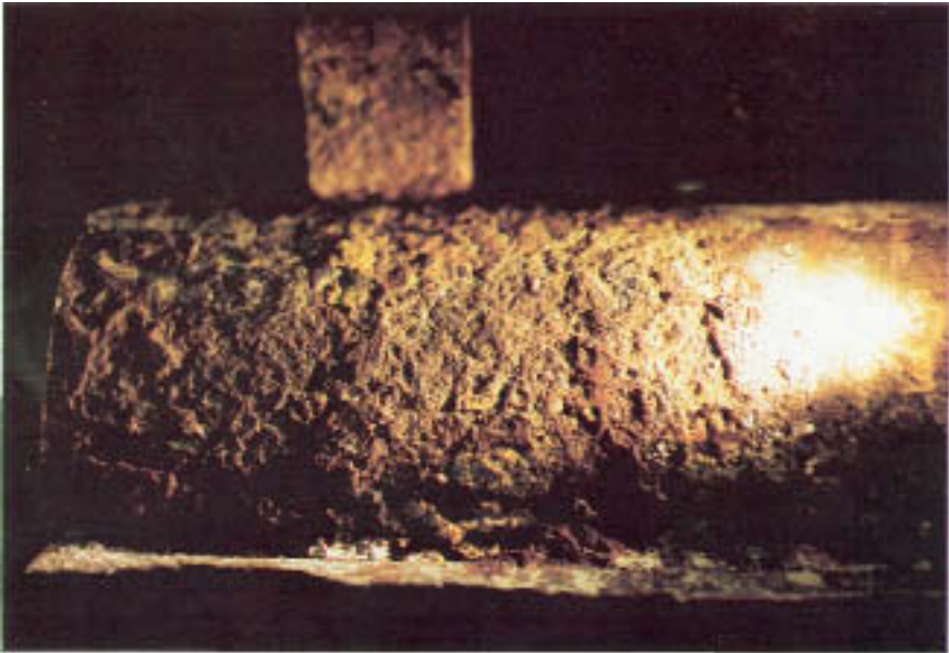
Figure 13.5 Idle-time corrosion occurring beneath refractory.
