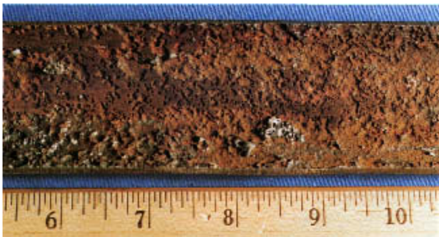
Figure 5.6 Internal surface of downcomer tube.
