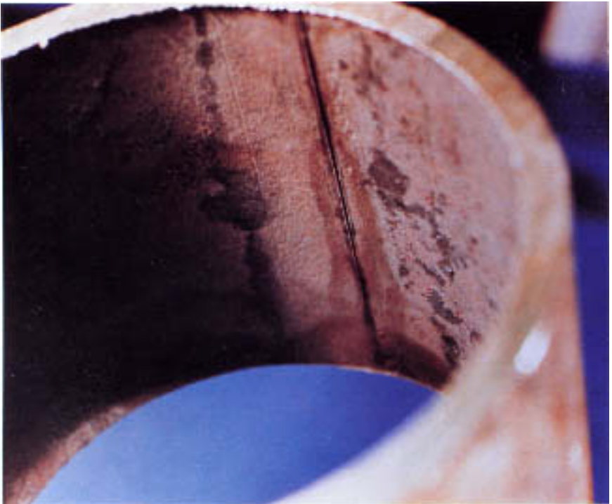
Figure 19.8 Seam defect in steam line.
