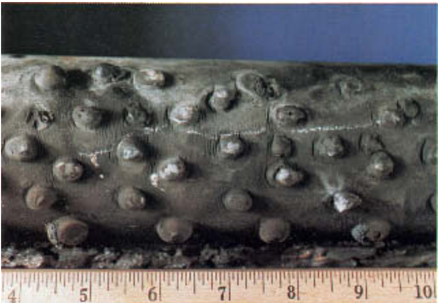
Figure 15.8 Transverse fissures at and near stud bases.
