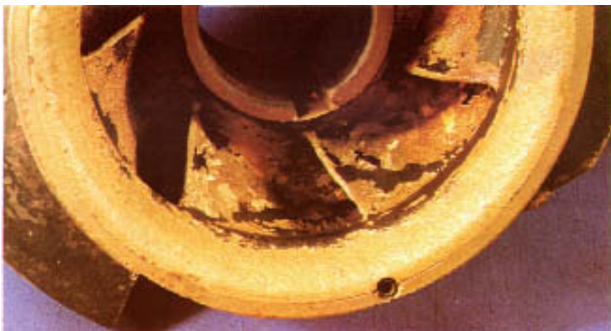
Figure 5.5 Chelant corrosion on feedwater pump.
