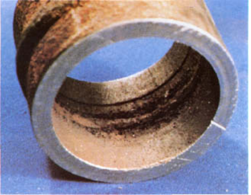
Figure 7.9 Acid corrosion at weld.
