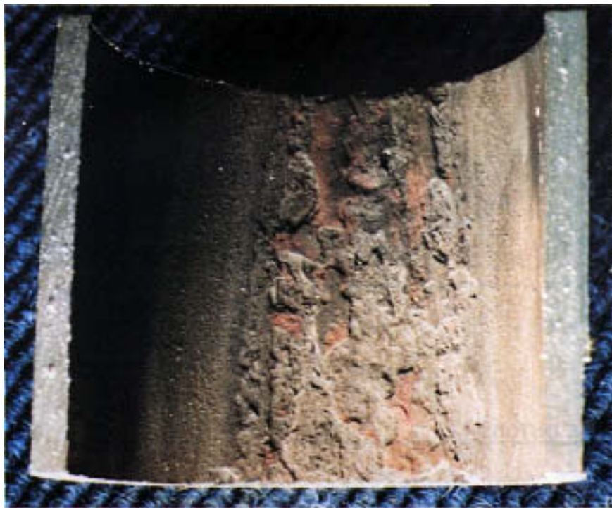
Figure 4.14 Internal surface showing wasted metal.
