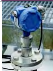
Rosemount 3300 Guided Wave Radar Installed
