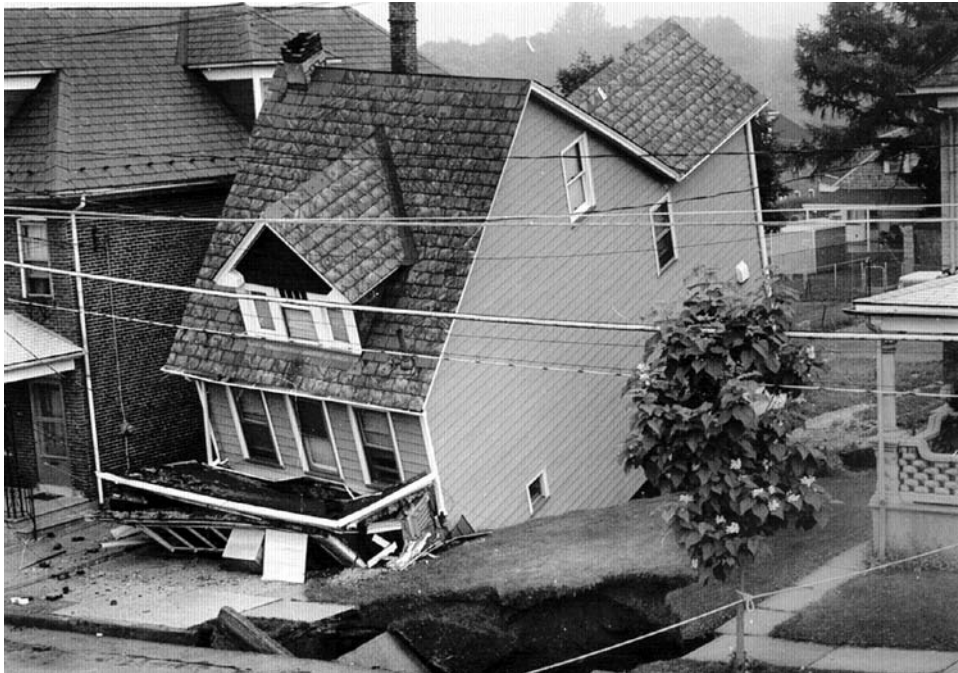
Figure 8.3. Terminal damage to a timber-frame house in Phillipsburg, New Jersey, caused when sinkholes developed underneath it and under the sidewalk after a water main burst beneath the street.
