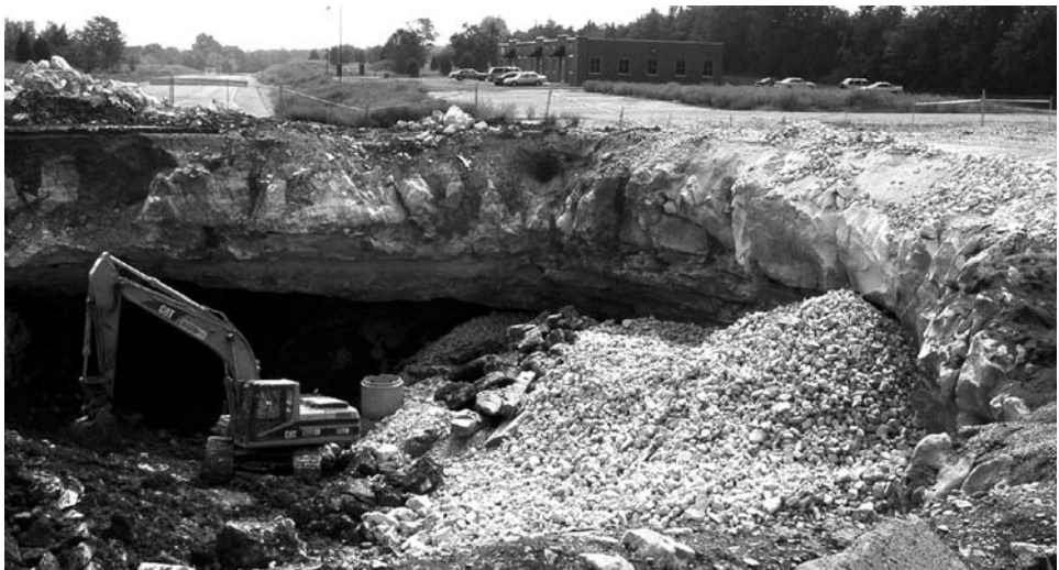
Figure 13.2.4. The edge of the collapse zone under Dishman Lane, showing the deeply fissured limestone rockhead beneath the red clay soil cover.
