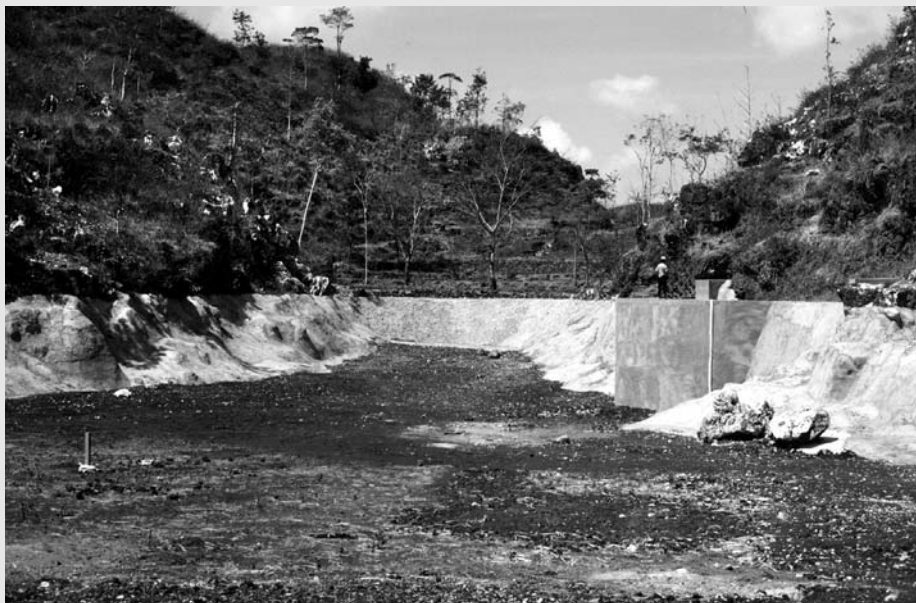
Figure 2.1.2. The Puleirang doline as modified in 1982, with its mortar-sealed slopes, graded clay floor and the concrete dam around the open sink. TW.
