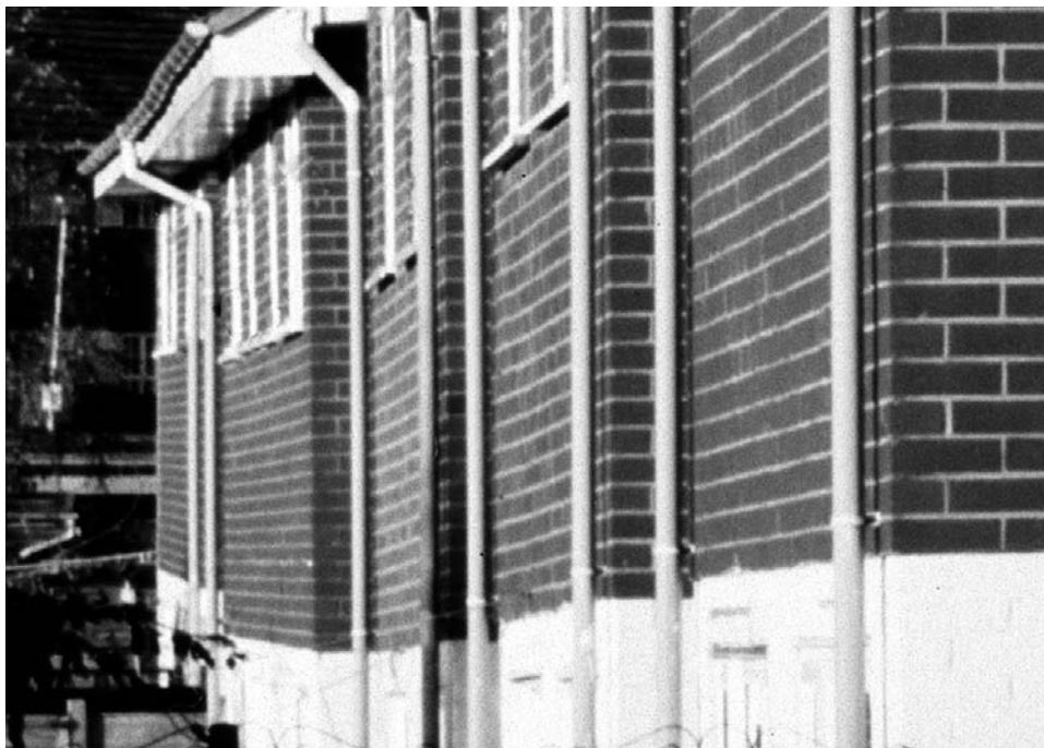
Figure 2.8. Houses in Sandbach subsided and tilted due to dissolution and removal of salt from the rockhead zone beneath 20 m of drift cover, in the Cheshire Plain, U.K. TW.
