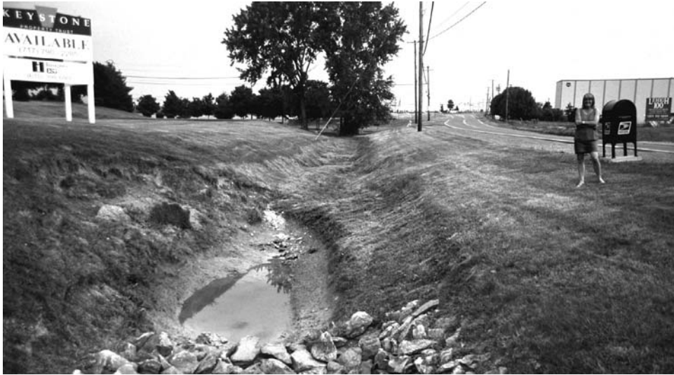
Figure 8.1. Early stages of a sinkhole developing in the untreated soil floor of a ditch beside a Pennsylvanian highway; it is temporarily choked with clay, while the riprap in the foreground was placed to prevent erosion at a culvert outlet.
