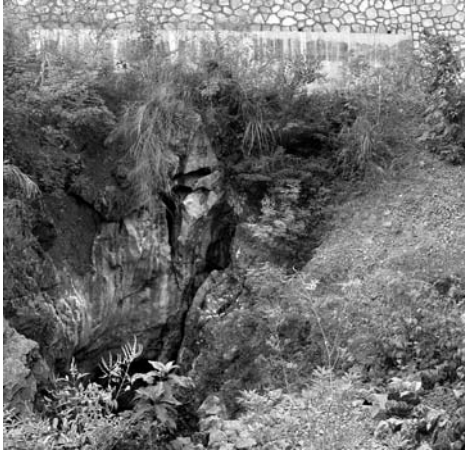
Figure 13.5.6. A concrete slab spanning wide and deep fissures in exposed limestone, with hand-placed stone facing on the road embankment above.
