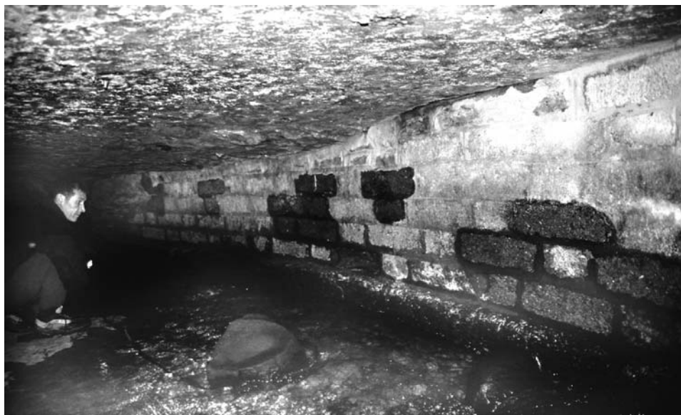
Figure 12.13. A masonry wall built beside the underground stream inside the St. Augustine's Cave in Ireland in order to reduce the unsupported span beneath a main road that stands on a concrete slab.
