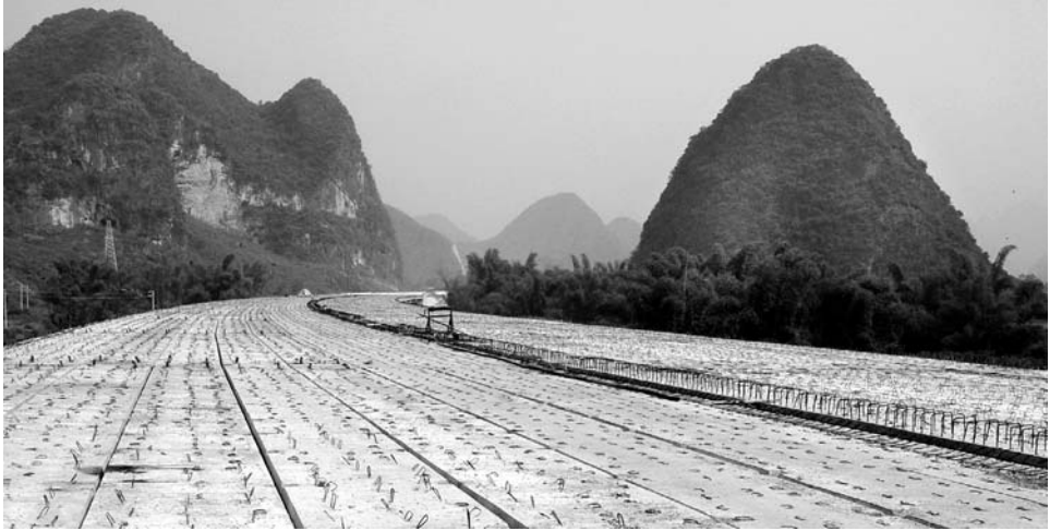
Figure 13.5.1. The deck of a long viaduct with piled piers carrying the Shui-Nan Highway over difficult karst ground between steep conical hills in the fengcong karst. Photo: Mingtang Lei.
