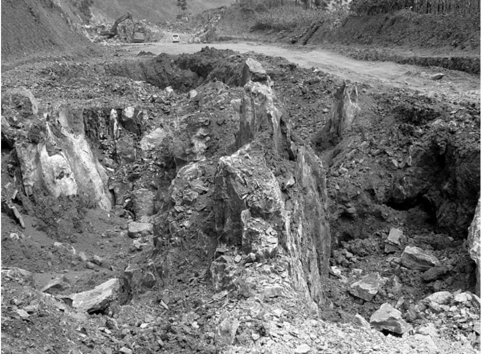
Figure 13.5.5. Excavating the soil fill from fissures and hollows between elongate, bladed pinnacles in the karst rockhead, before building the Shui-Nan Highway.
