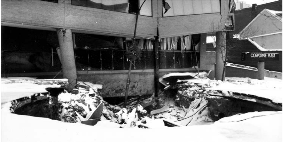
Figure 13.7.3. The Seventh Street facade of Corporate Plaza damaged by the collapsing sinkhole. The column on the left is damaged over its subsided column base, exposed except for a thin cover of snow and debris. The column in the centre has its steel stanchion hanging from the building's frame after all its footing has dropped into the sinkhole and its brick cladding has fallen away. The corner column, on the right is almost undisturbed. Photo: Percy Dougherty.
