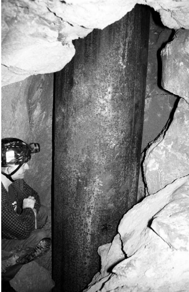
Figure 13.6.4. A caisson that supports the Courthouse in Huntsville, passing through the major zone of karstic breakdown along the northern side of Big Spring Cave. TW.
