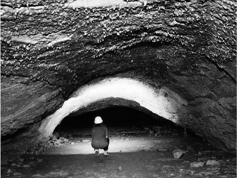
Figure 13.4.4. The stable arch roof in sound basalt where the Sung Gul lava tube lies directly beneath the main road. TW.
