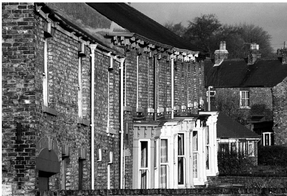
Figure 2.9. A terrace of houses in Ripon, U.K., subsided due to a combination of rockhead dissolution of gypsum and compaction of soft sediments filling an old buried solution doline. TW.
