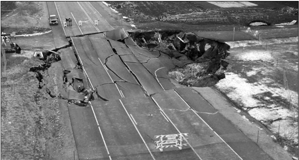
Figure 13.2.1. Aerial view of the collapse sinkhole in Dishman Lane, Bowling Green, seen looking towards the south-east
