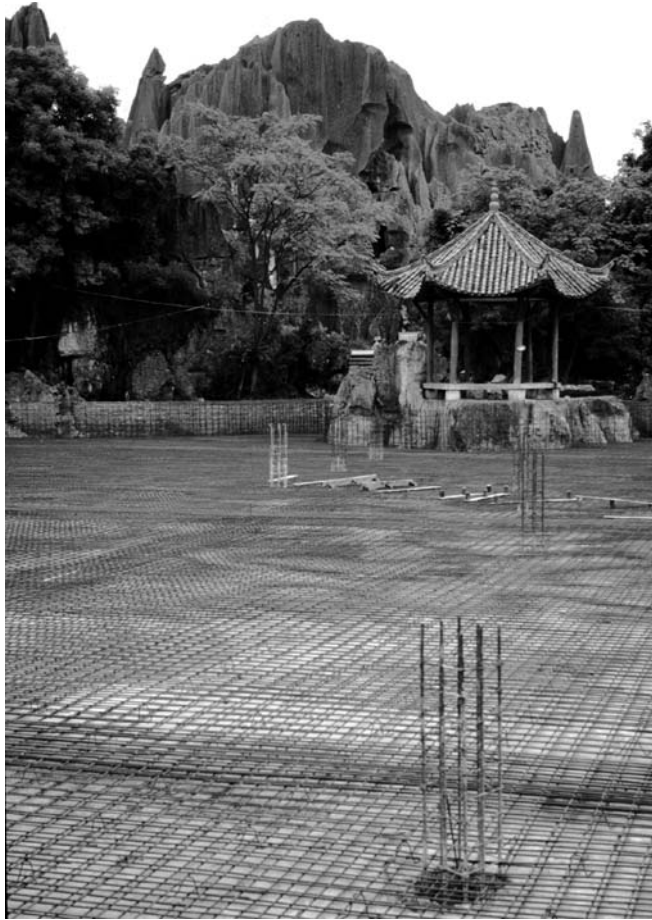
Figure 12.2. Double weldmesh reinforcement for a concrete slab, cast as foundations for an ornamental lake with a bridge and pagoda, on deep soils over pinnacle karst at Shilin, southern China.
