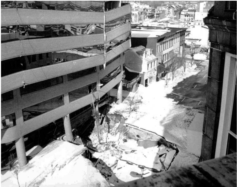
Figure 13.7.1. The newly collapsed sinkhole in Seventh Street, with the conspicuous sag in the Corporate Plaza building above it.
