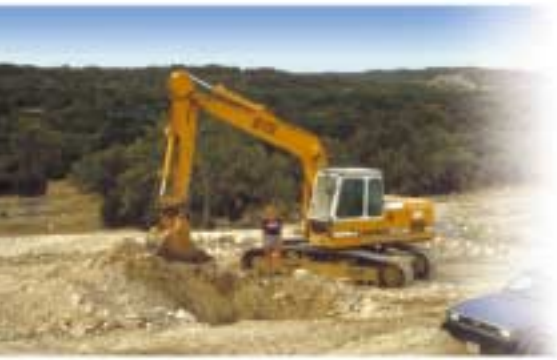
Fig. 49. A road being built over and sealing a cave runs the risk of collapse and problems with water quality and quantity.
