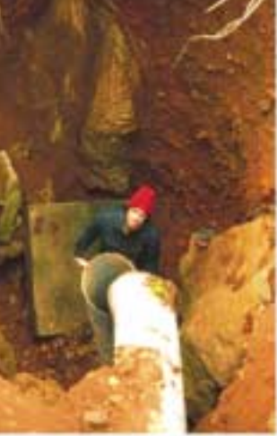
Fig. 37. (Above) A large sinkhole collapse around a poorly installed drainage well.
