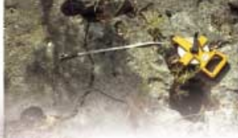
Fig. 11. The fractures and pits in this limestone have become larger as the surrounding rock dissolved by solution.
