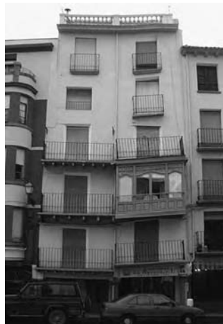
Figure 12.12 (Upper) Subsidence of buildings in Calatayud, Spain. Damage is mapped on a four-part scale, from None to Very Severe. Reproduced from Gutierrez, F. and Cooper, A.H. (2002) Evaporite dissolution subsidence in the historical city of Calatayud, Spain: Damage Appraisal and Prevention. Natural Hazards , 25, 259–88. (Lower) Moderate damage in the main square of the town.
