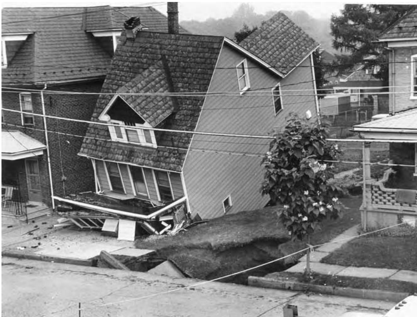
Figure 12.8 Subsidence of a timber-frame house into a collapse sink-hole, Phillipsburg, New Jersey. The sink-hole was created when a water main leaked, surcharging soil-mantled epikarst. (Photograph by Rick Rader, with permission.)
