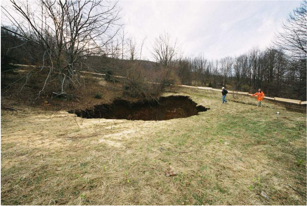
Fig. 7.47 Brinje Tunnel collapsed all the way to the surface of the terrain
