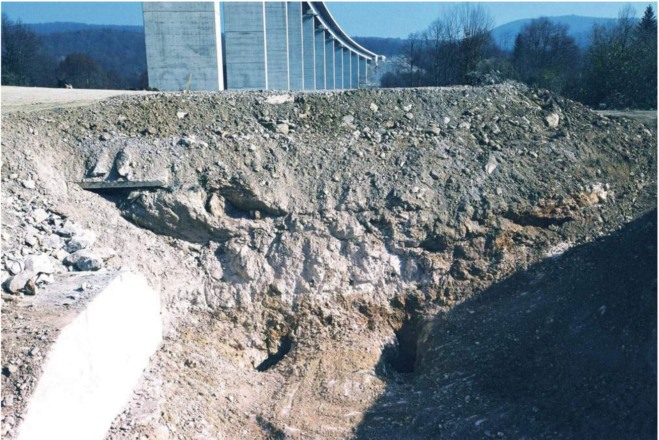
Fig. 8.3 Entrance to cavern at km 70 + 510 under pillar S-7 of Zečeve Drage Viaduct
