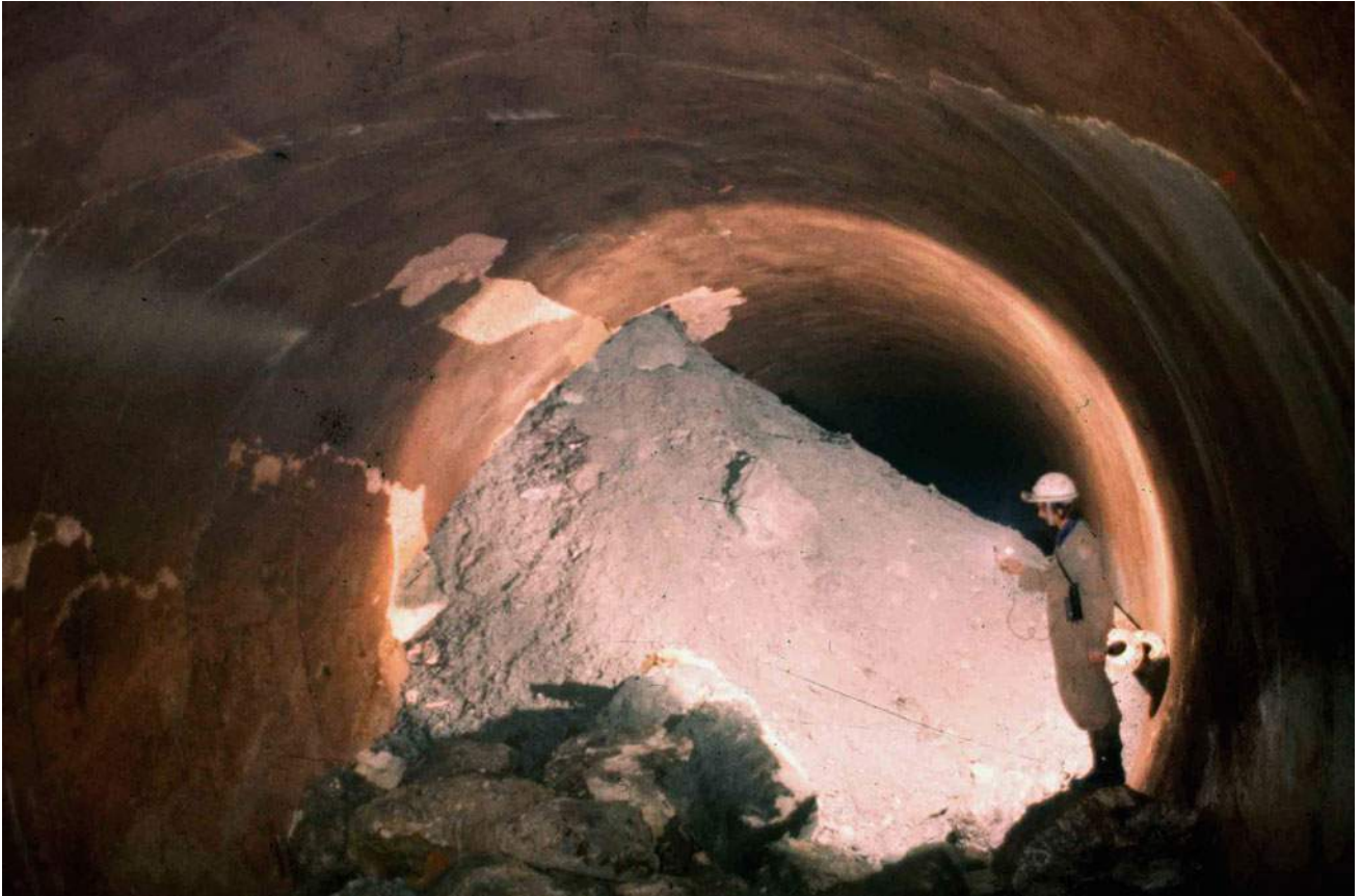
Fig. 5.20 Numerous caverns were found in Zakučac hydrotechnical tunnel
