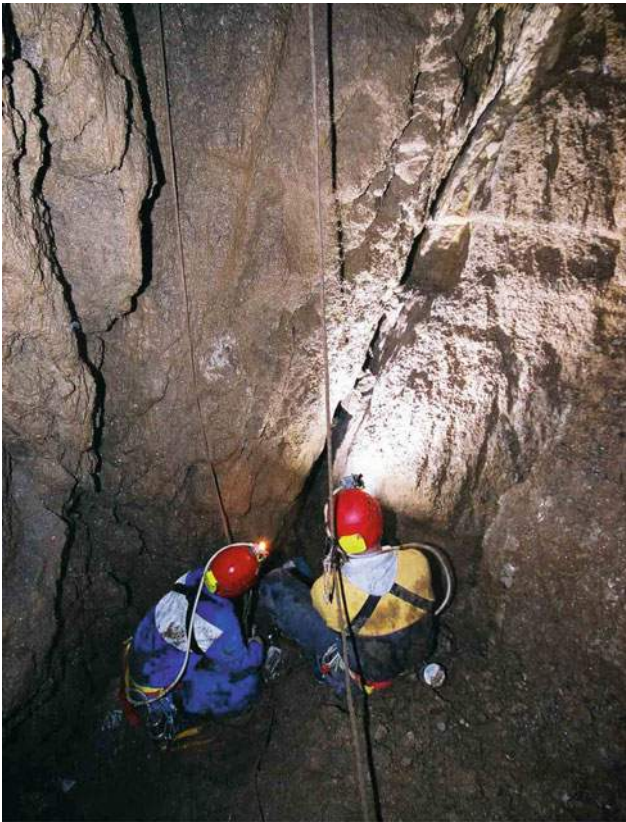
Fig. 8.39 Cavern in the embankment at km 22 + 950
