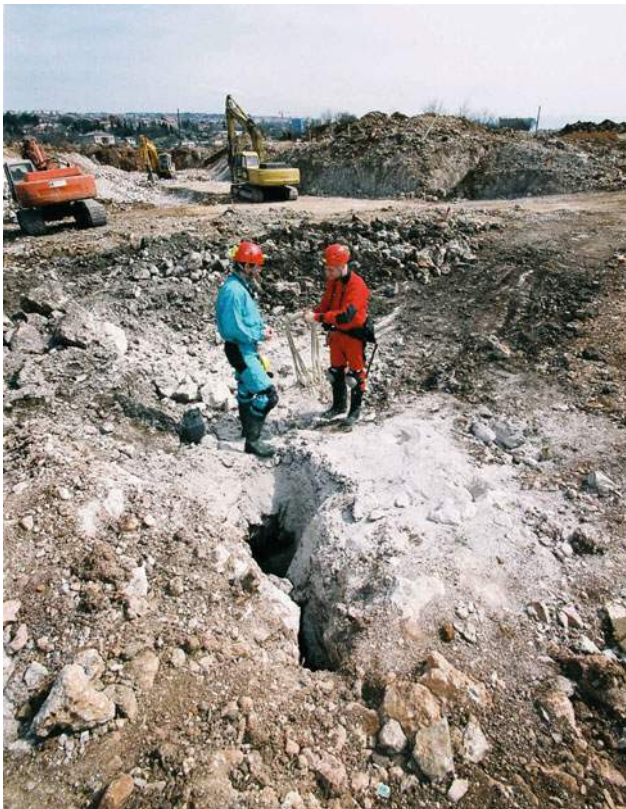
Fig. 8.46 Cavern at km 0 + 160 on Rujevica road junction, ramp 5, in Rijeka
