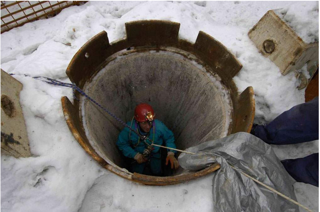
Fig. 8.41 Entrance in cavern under pillar S-9 (right) in the "Zečeve Drage" viaduct
