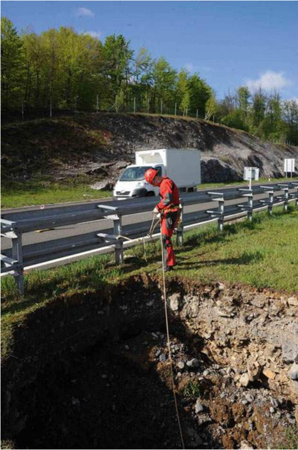
Fig. 8.42 Cavern at km 9 + 000 in the green grass area between two lanes,
