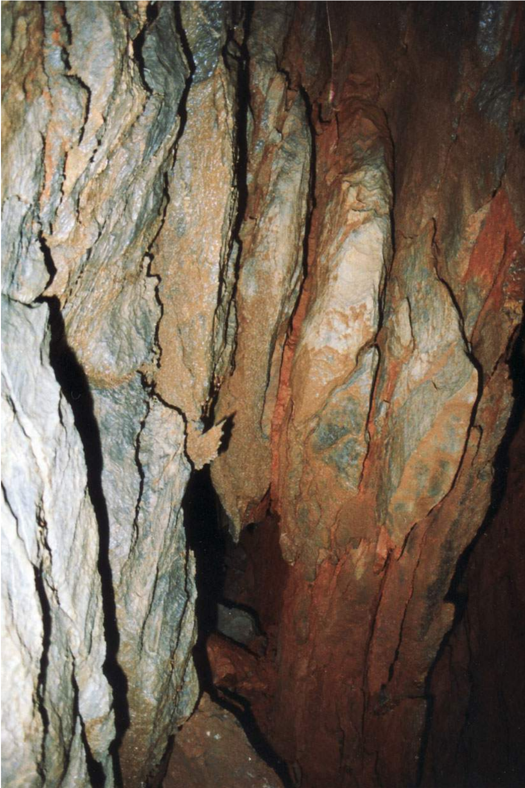
Fig. 6.14 Vertical fissures in cavern km 24 + 433 in Tuhobić Tunnel
