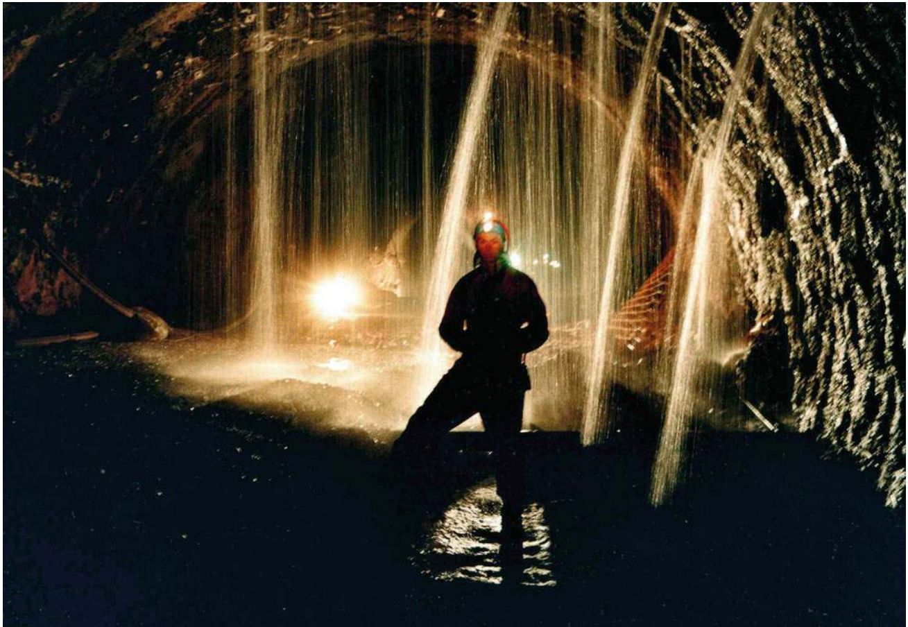
Fig. 7.12 Cavern at km 198 + 645 in Sveti Rok Tunnel—high groundwater level during rainy periods
