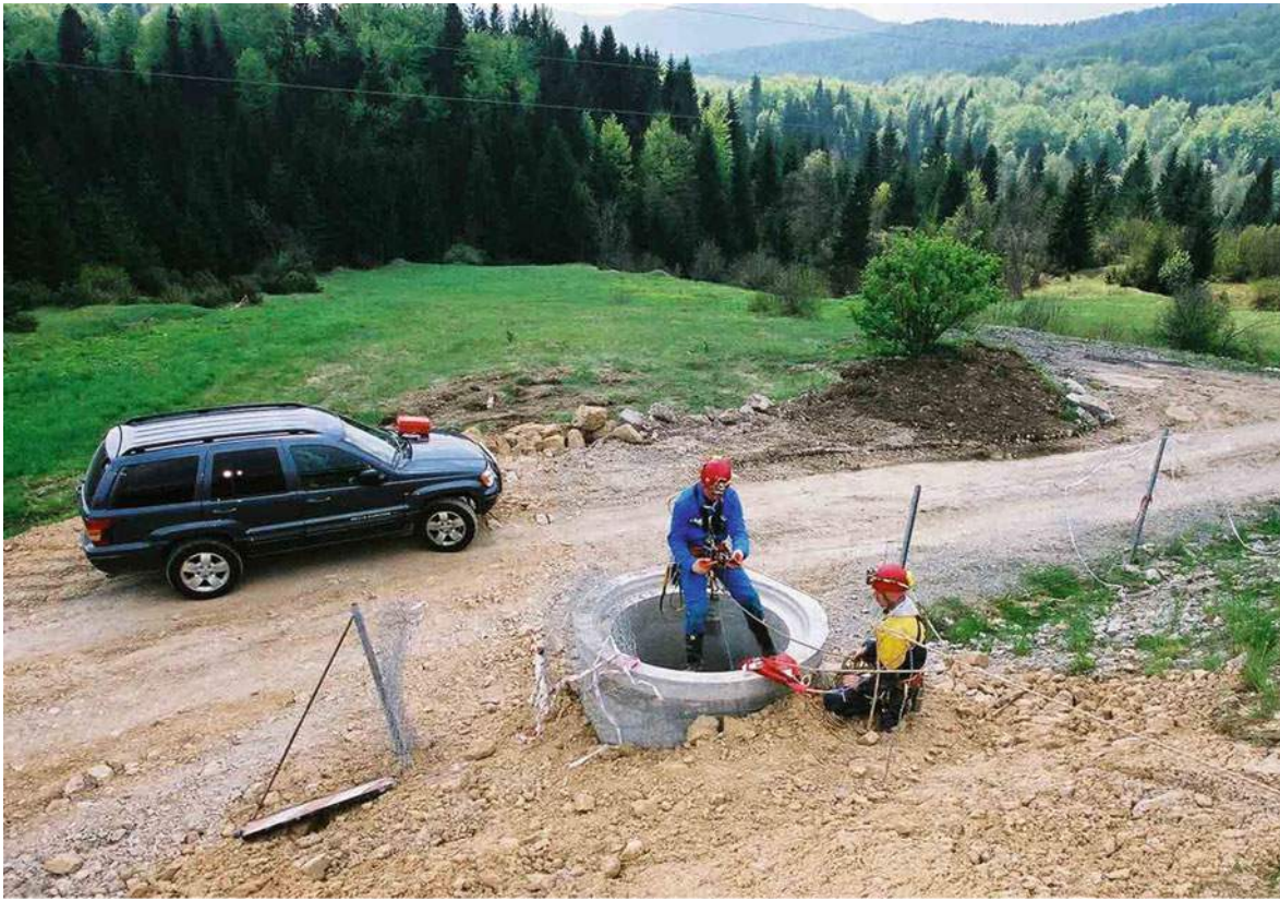
Fig. 8.38 Entrance to cavern in the embankment at km 22 + 950
