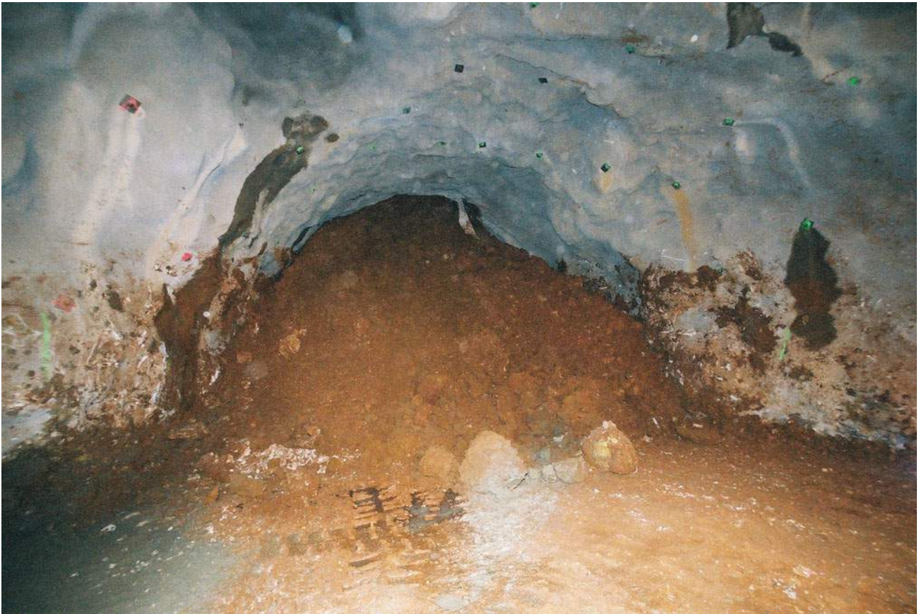
Fig. 7.49 Inside the Brinje Tunnel in time of collapsing
