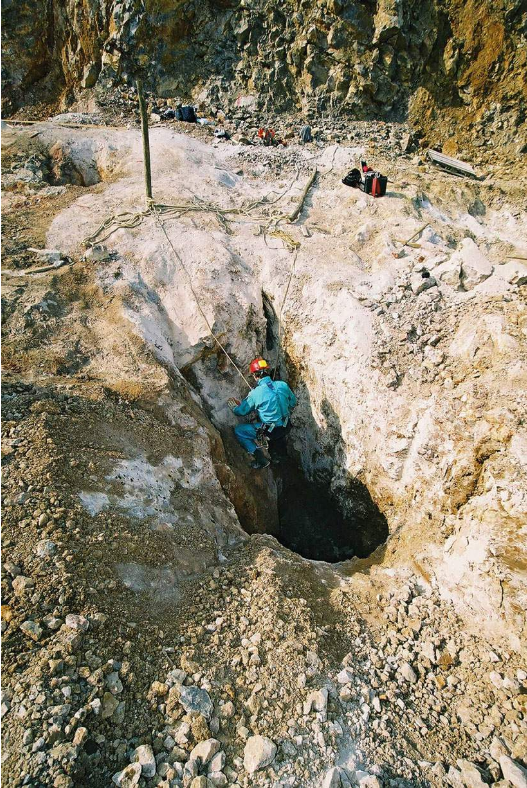
Fig. 8.10 Cavern at km 2 + 020 under pillar S-3 (left) Jezerane Viaduct
