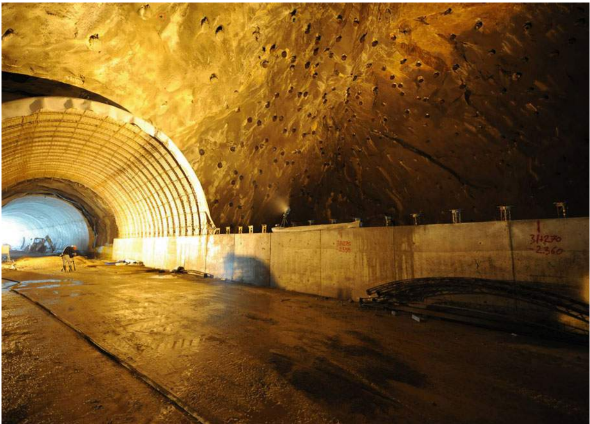
Fig. 6.68 A 58-m-long bridge was built across the cavern at km 31 + 292 in Vrata Tunnel
