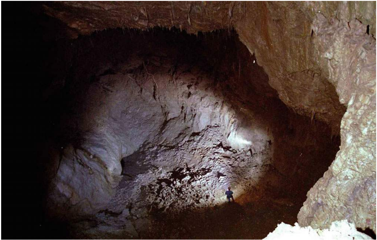
Fig. 8.8 Big cavern at km 1 + 281 under pillar S-4 of Kačjak 2 Viaduct
