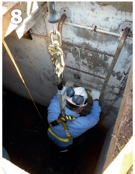
8 View of worker descending into a confined space attached to shock absorbing lanyard connected to a personnel-rated hoist mounted on a tripod.
