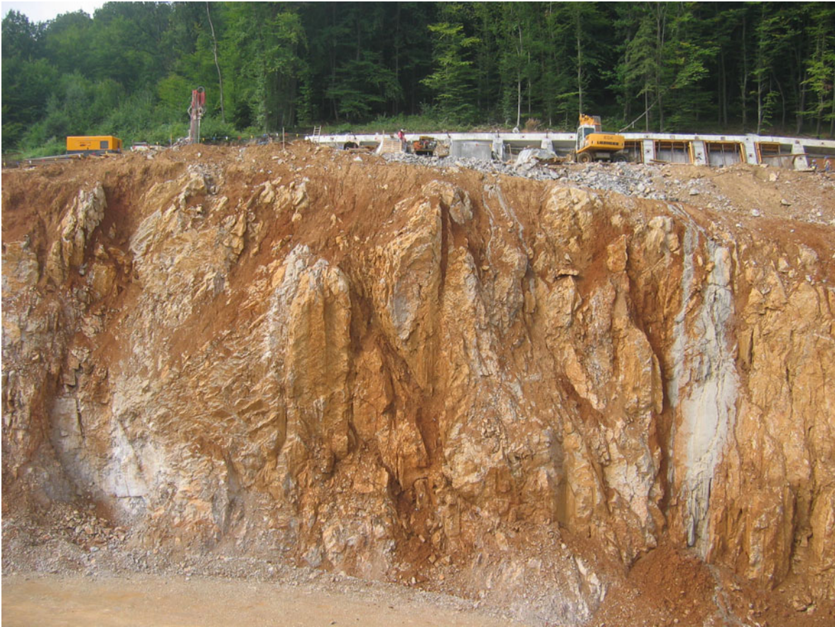
Fig. 21.3 Vertical subsoil channels on the walls of stone columns and of the shaft
