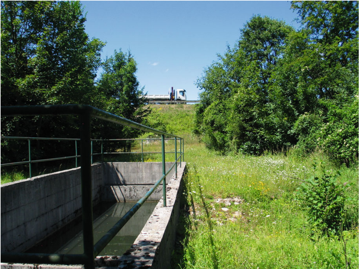
Fig. 27.1 Oil separator is a treatment facility for mechanical treatment of road drainage: sedimentation of suspended material and oil separation. It can be used for trapping spillages caused by traffic accidents
