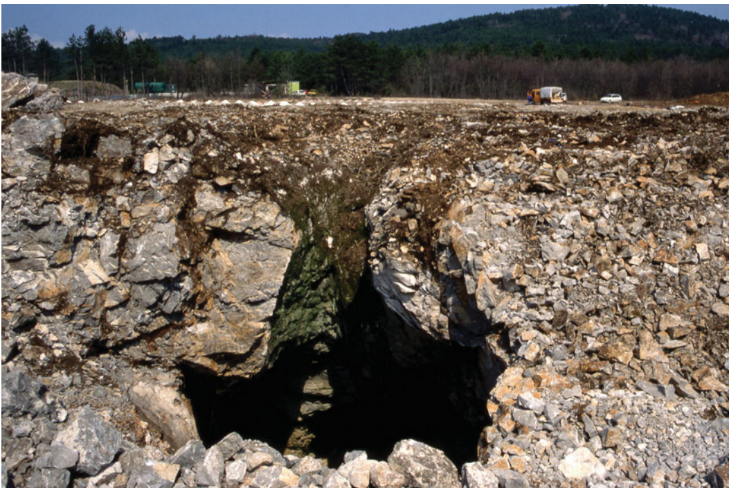
Fig. 1.12 Roof of a cave which collapsed during construction
