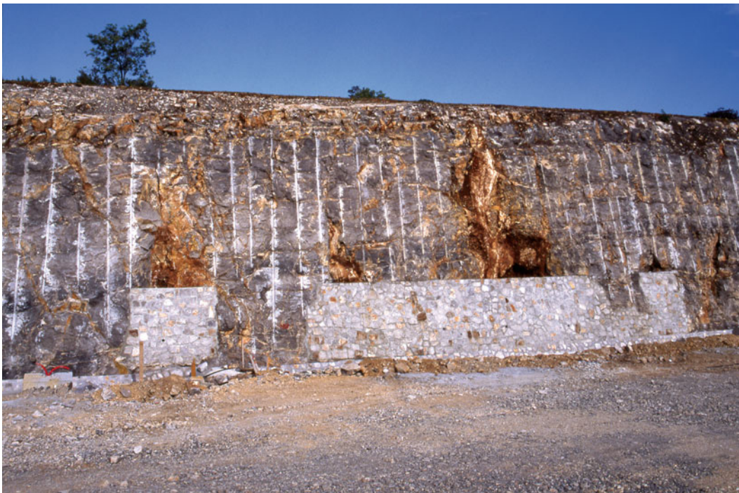
Fig. 5.6 Caves in the embankment of a motorway roadcut that were closed with rock walls
