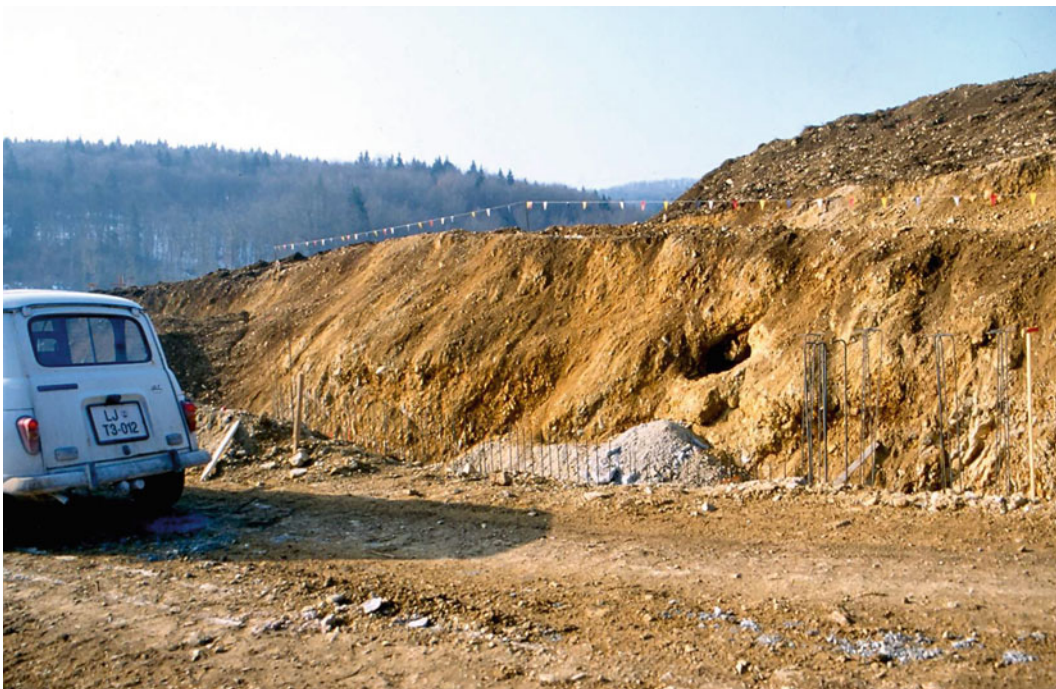
Fig. 15.9 Entrance to the shaft in the cutting of the Mali Medvedjek hill
