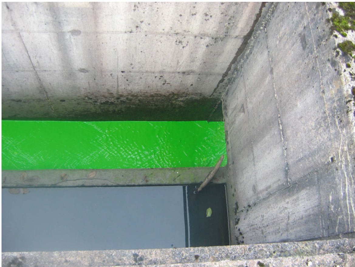
Fig. 28.9 Outflow of uranium from the sinking stream of the oil separator B at Postojna
