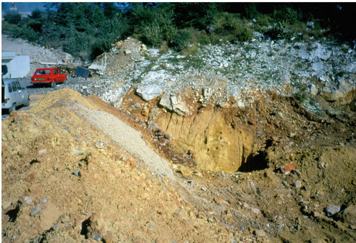
Fig. 11.1 A filled cave south of Divača in a doline on the eastern edge of the construction site of the motorway section Divača–Kozina
