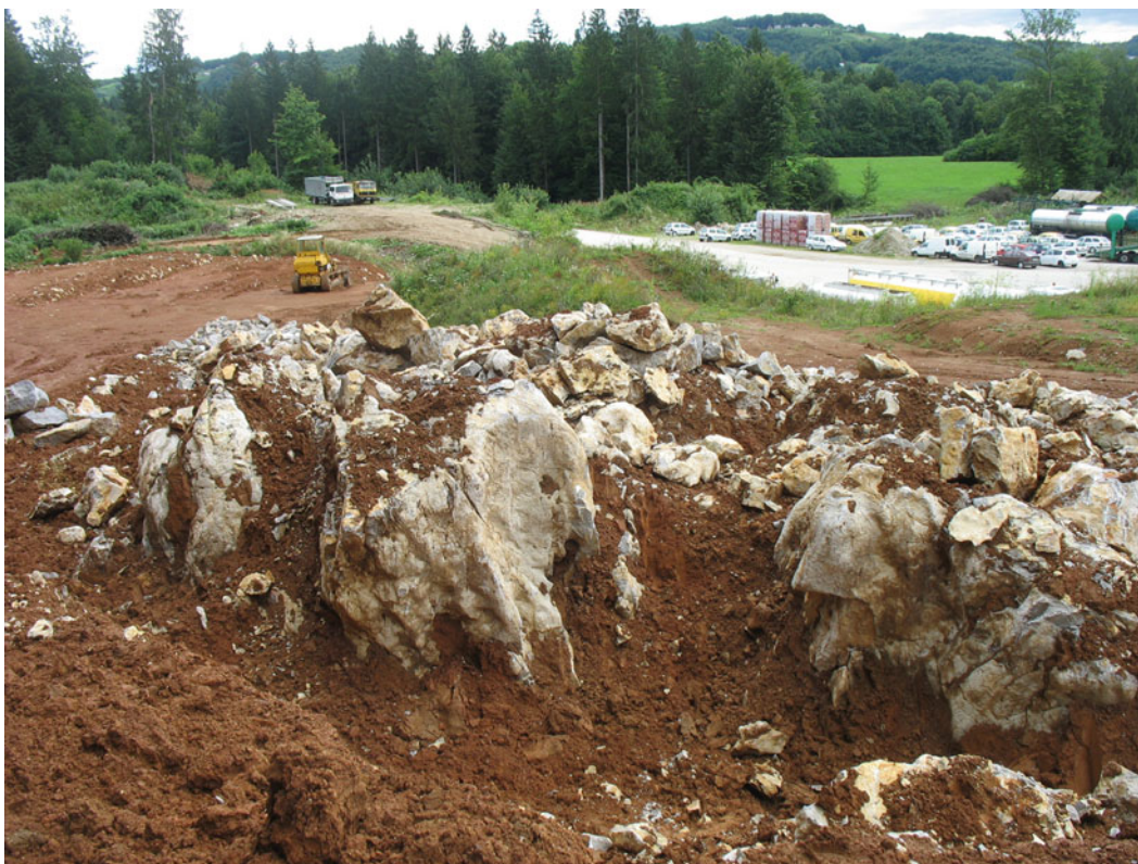
Fig. 16.1 Subsoil stone forest on the Pluska–Ponikve motorway section
