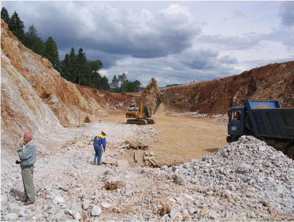
Fig. 20.2 Construction of the highway north of Novo mesto has an exposed profile of laminated grey sediments, which were covered by red soil. The profile lies behind the drilling machine in the middle of the photo
