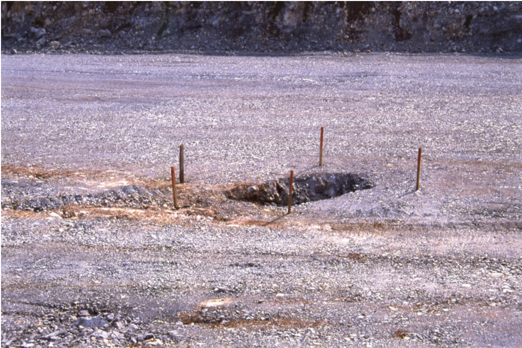
Fig. 5.7 A subsidence in the motorway
