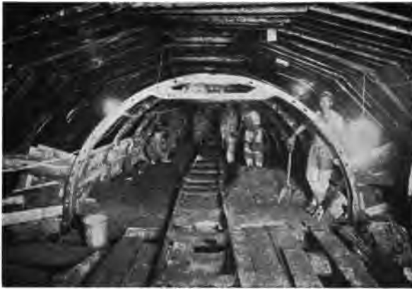
FIG. 132.—Ogier's Run Intercepting Storm-Water Drain, Baltimore, Maryland.
