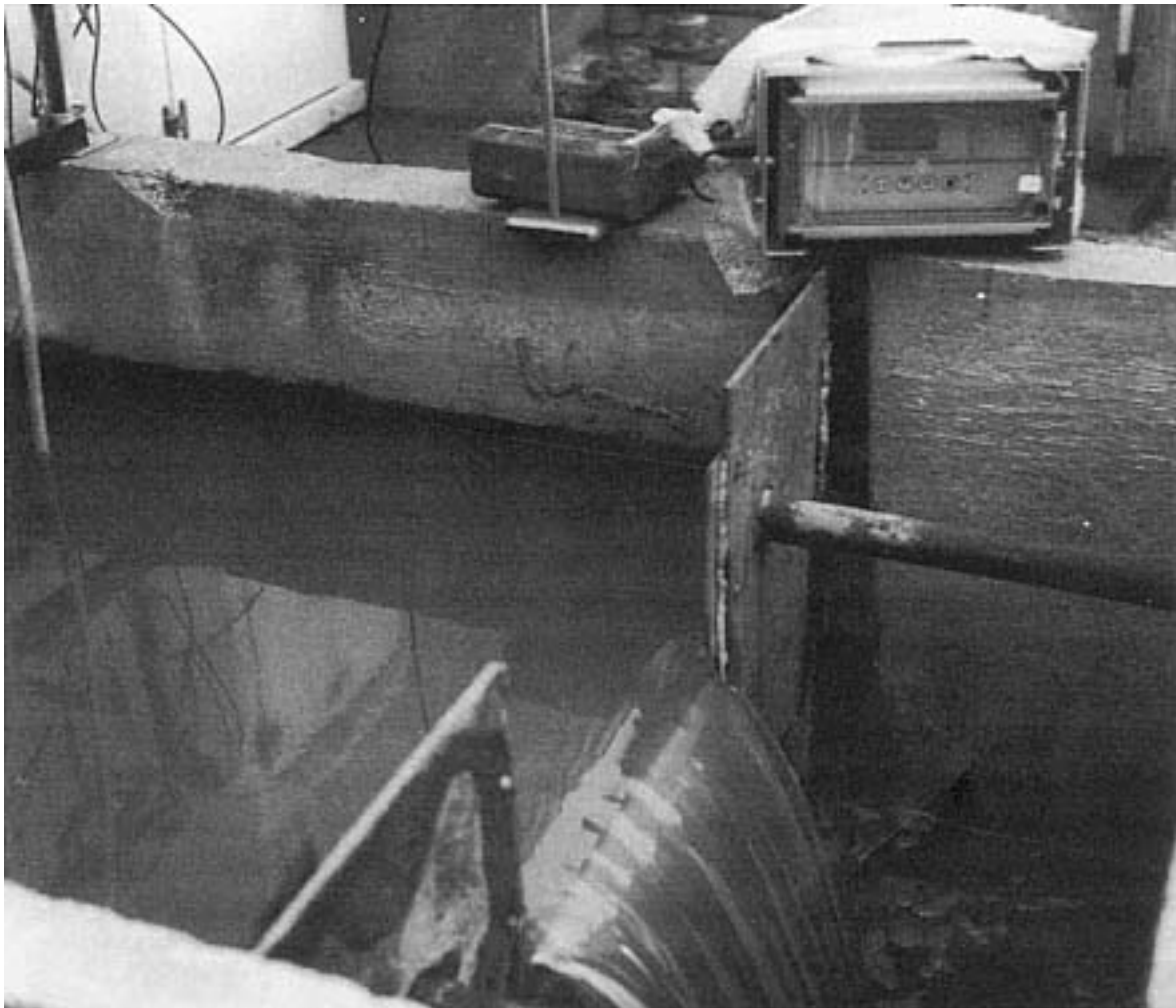
Figure 8.3 Portable flow recorder on site.
