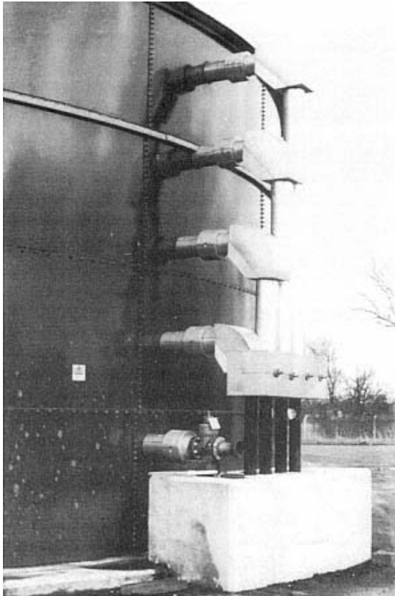
Figure 5.1 Grp-coated sludge dewatering tank and dewatering valves.
