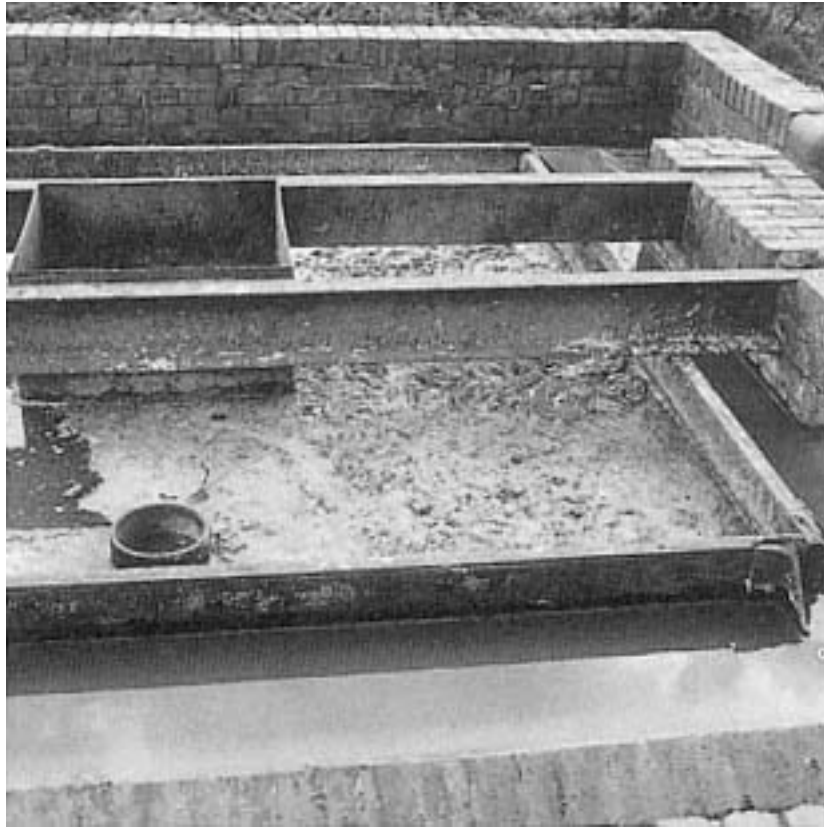
Figure 6.14 Primary settlement tank with floating scum.
