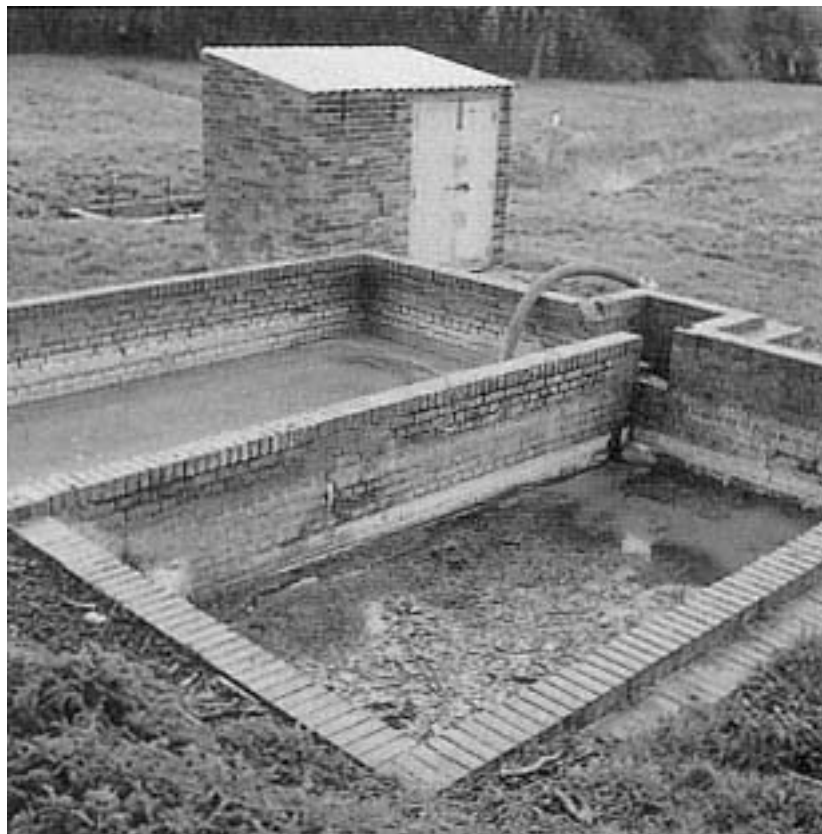
Figure 6.13 Sludge storage bays.
