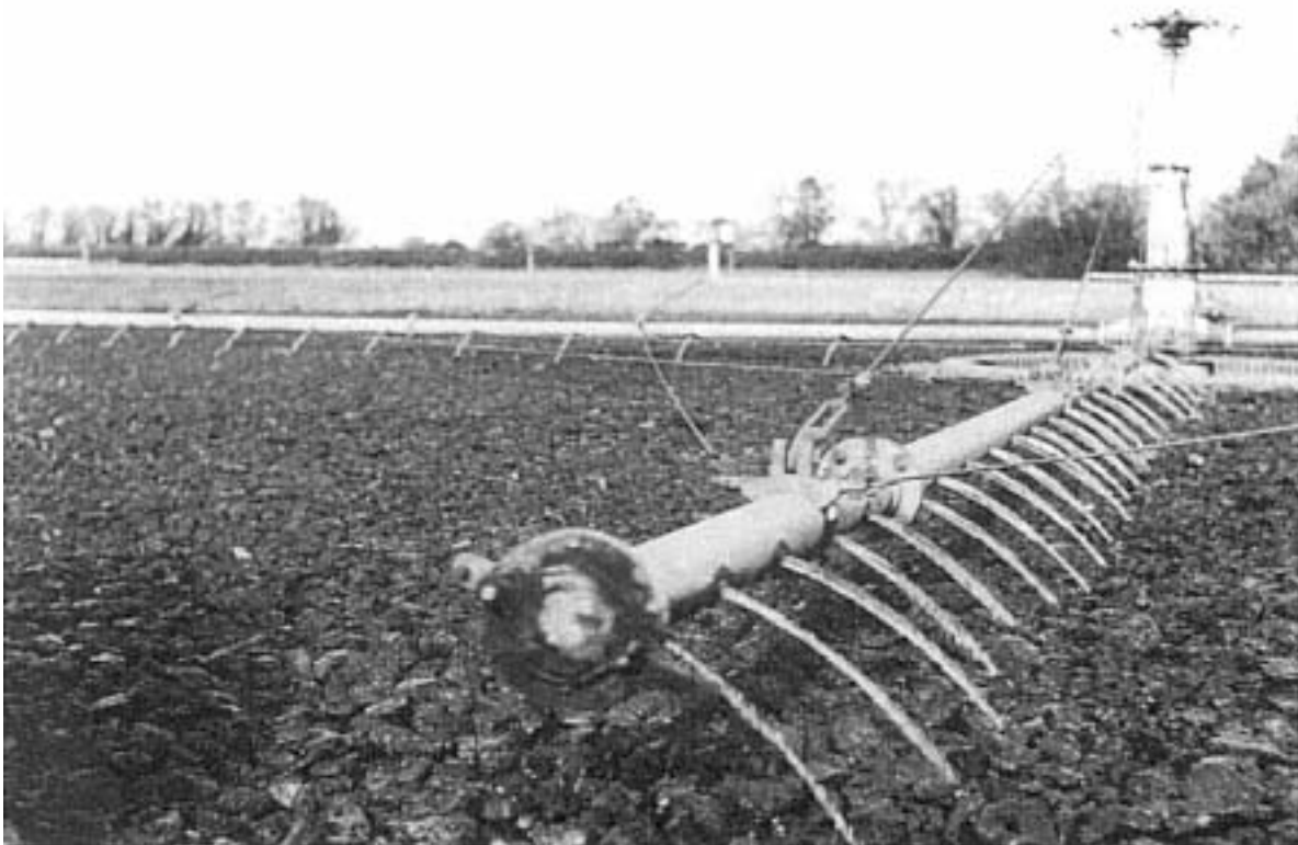
Figure 4.1 Close-up of the distributor arm of a circular percolating filter.
