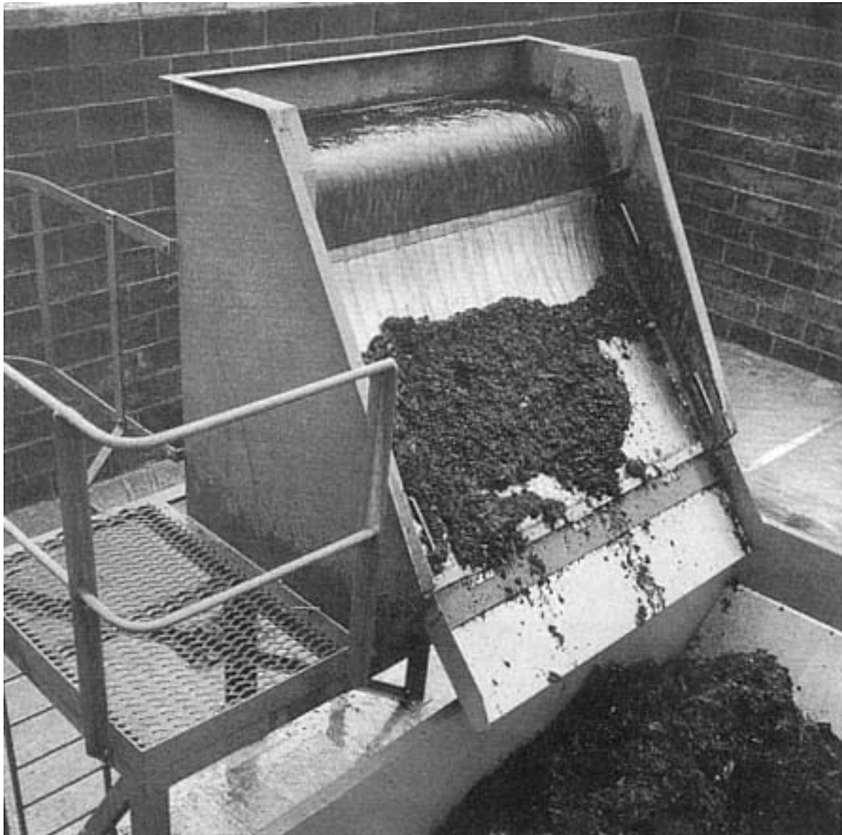
Figure 1.3 Rundown screen. (Courtesy: Environmental Engineering Ltd.)
