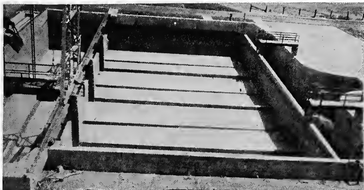
FIG. 75.—View of storm-water stand-by tank at North Toronto sewage-treatment plant, Toronto, Ont.
