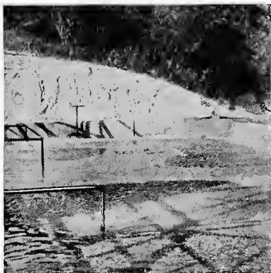
FIG. 73.—Skimming nozzles in preliminary-sedimentation tanks at North Toronto sewage treatment plant, Toronto, Ont.
