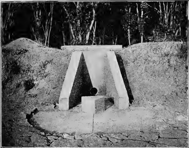
FIG. 112.—Outlet at sand-filter bed, Marlborough, Mass.
