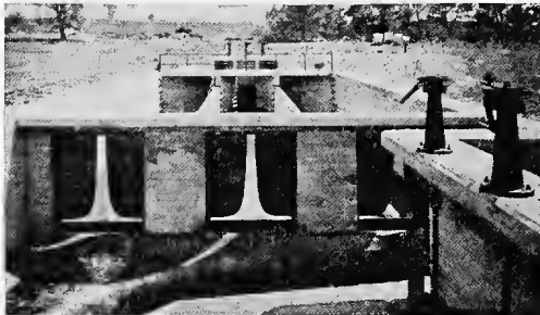
FIG. 67.—Outlet end of grit chambers at sewage-treatment plant, Springfield, Ill., showing proportional weirs.
