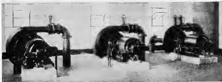
FIG. 193.—Centrifugal air compressors geared to induction motors at Irwin Creek sewage-disposal plant, Charlotte, N. C.
