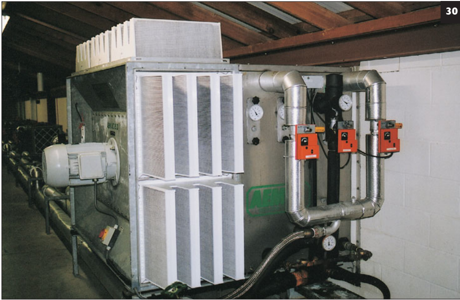
30 A large absolute-filter assembly with the filter units projecting. This assembly is in the roof space above the units requiring filtered air.
