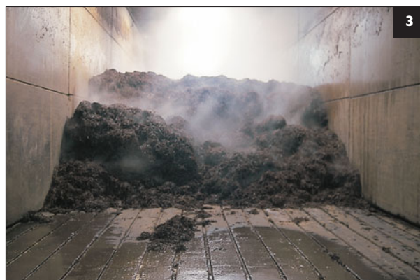
3 Phase I bunker with underfloor ventilation holes in the lines in the concrete.
