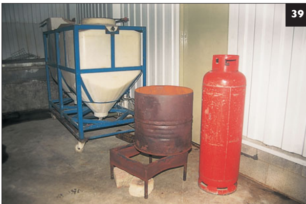
39 Equipment used for formalin fumigation. The large metal container holds the formalin and a bottle gas supply provides the fuel for the heat for vaporization.
