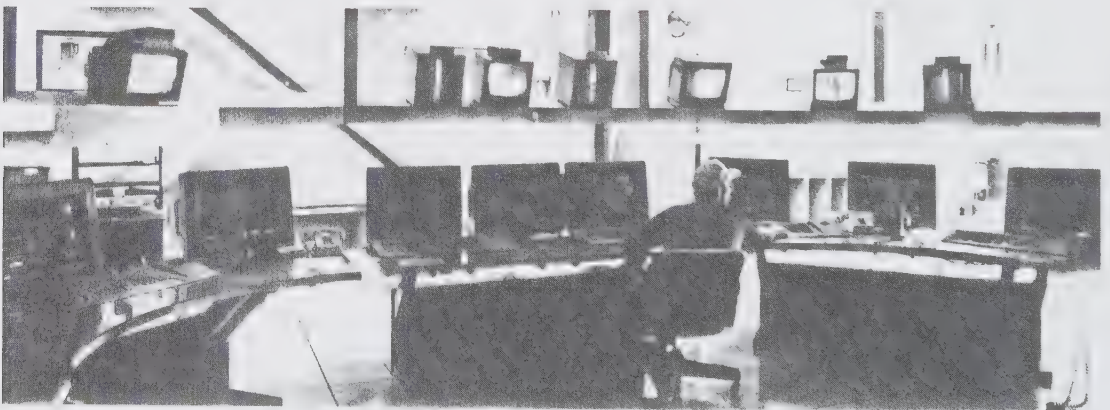
FIGURE 24-8. Video-based control room. (Photo courtesy of ABB).
