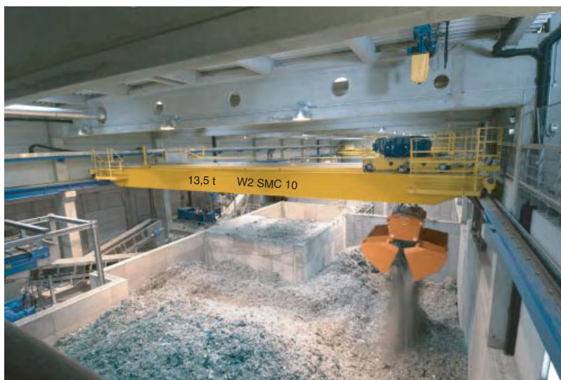
Figure 9.31 Typical storage system for high- and low-caloric residuals feeding incineration, using cranes, live bottoms, and special conveying equipment.
