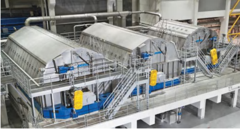
Figure 7.127 Mill installation of disk filters. (Source: Andritz.)
