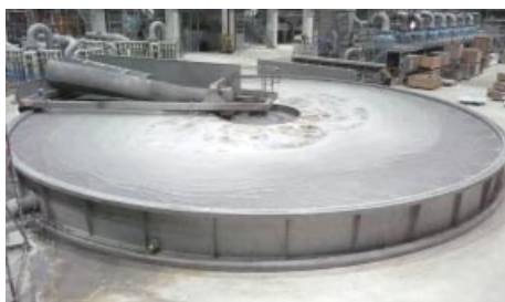
Figure 7.111 Photo of a tank for dissolved air flotation (DAF).
