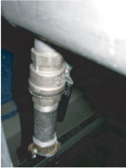
Figure 29.6 Sampling out of the pipes with the help of valves.
