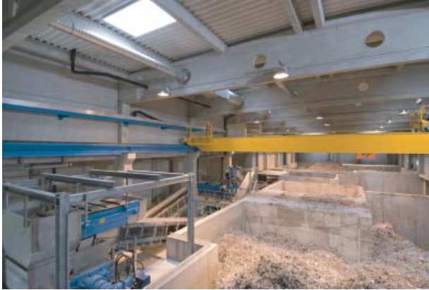
Figure 9.44 Typical storage bunkers with intelligent laser scanning crane, live bottoms, shredding, and metal separation.
