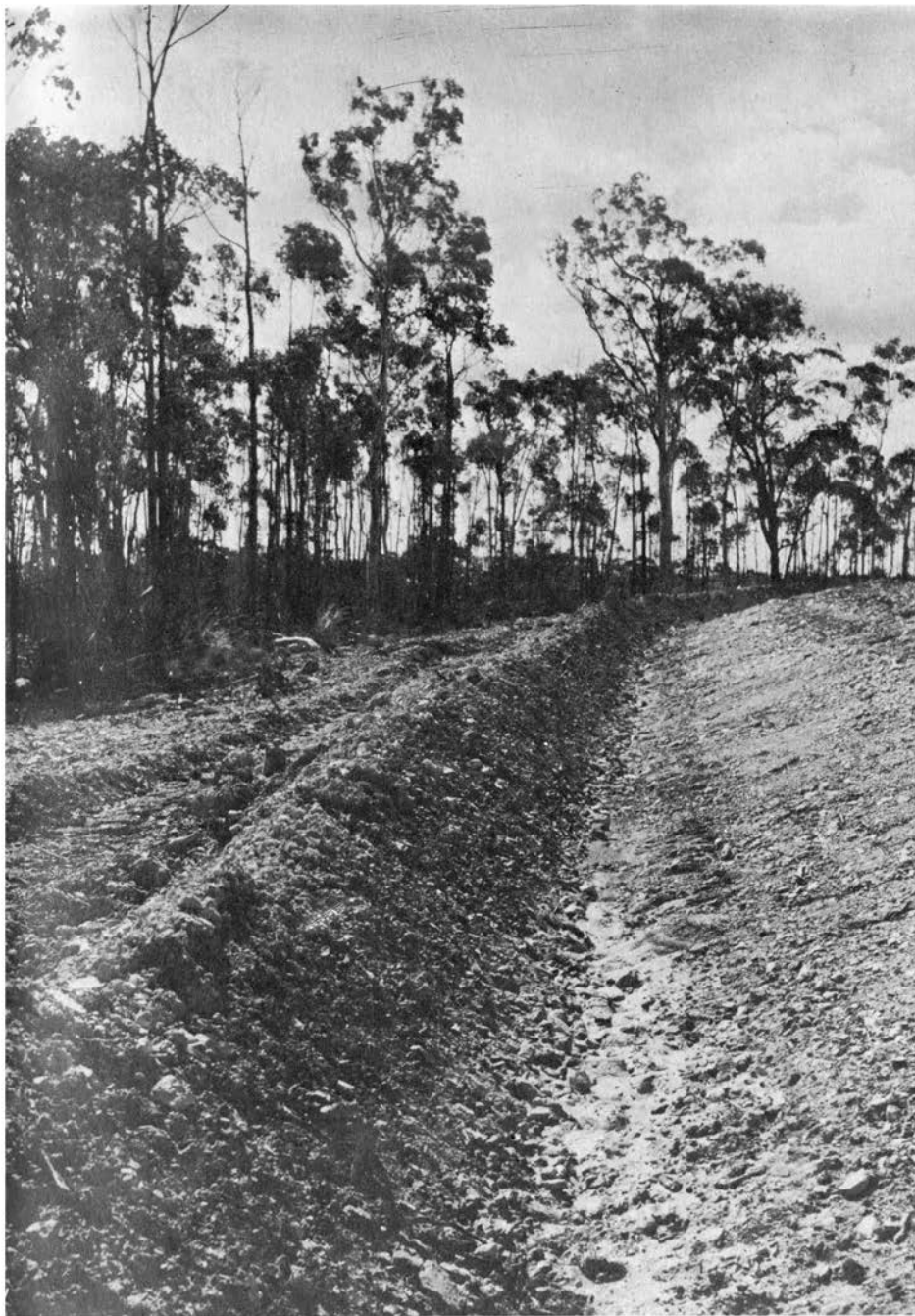
A Newly constructed diversion channel in medium undulating country. The channel has a fall of 1 in 300 and collects rainfall runoff from the hills above it to fill a farm dam for irrigation.
