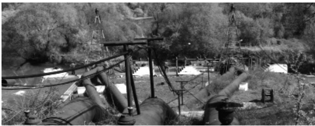
FIGURE 4 Floating pumping station on Mures River [3].
