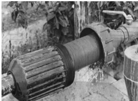
FIGURE 3 Disk filter: Flushing operation.
