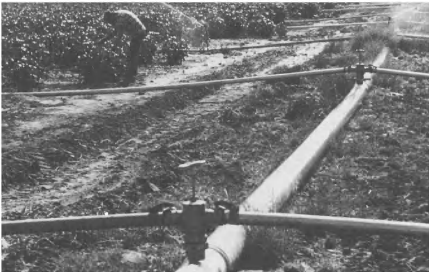
FIG. 4.6. Solid-set Sprinkler Laterals Connected to Portable Aluminum Mainline.
