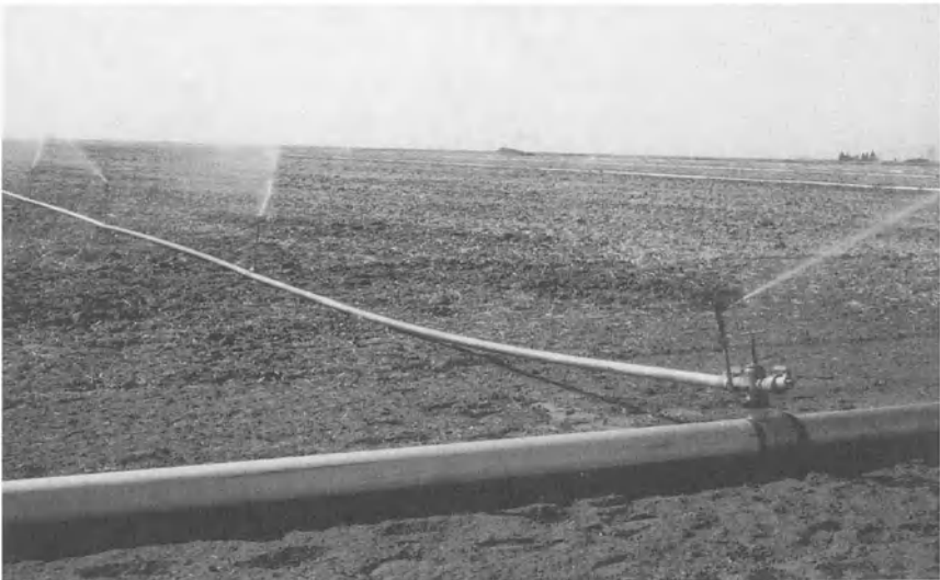
FIG. 5.3. Components of a Set Sprinkle Irrigation System Showing Booster Pump Supplying a Portable Main Line (Top) and Portable Main Line, Hydrant, and Sprinkler Lateral (Bottom).
