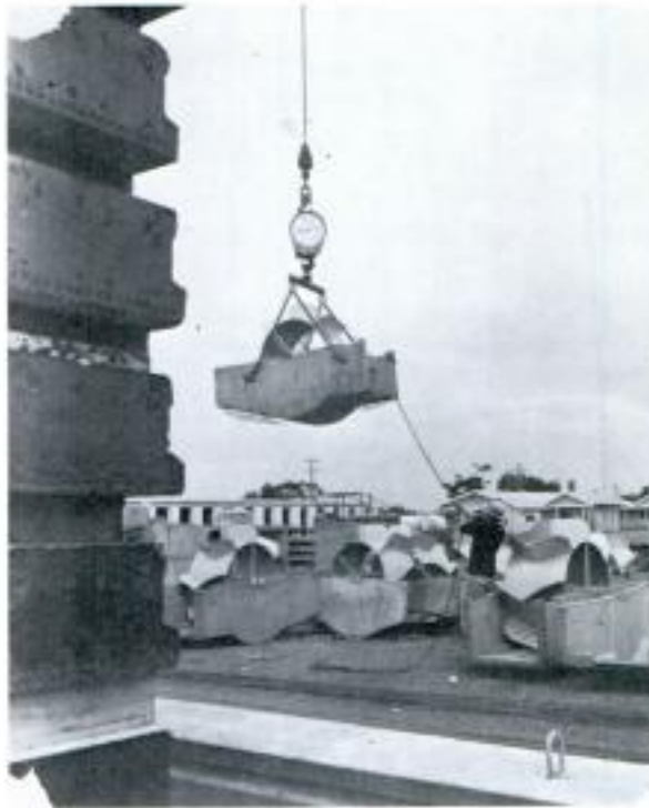
FIGURE 5-2. - Pre-cast large meter emplacement with wheels installed; note reinforcement to tie into cut-offs and pre-cast head wall.
