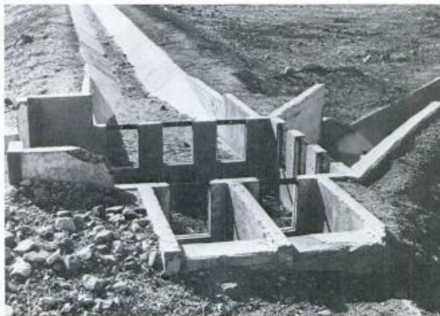
FIGURE 4-20 (a) and (b). - Distribution structure with proportional weirs constructed from prefabricated parts - East Ghor Extension Project, Jordan.
