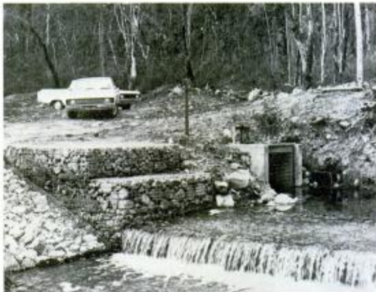
FIGURE 3-34. - Stone mesh basket construction, stone mesh apron, and location and general construction of inlet box with screen and screw-type gate. (About 3 \text{ ft}^3/\text{s} passing over the weir.)
