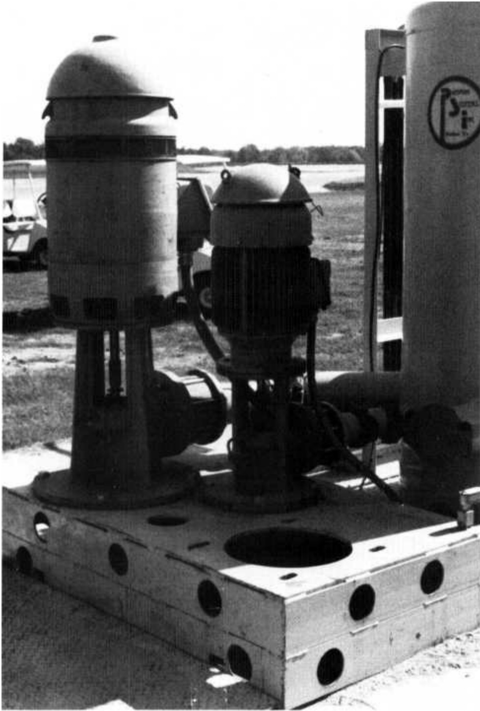
FIGURE 25. 11 Large pump, jockey pump, and pressure tank.
