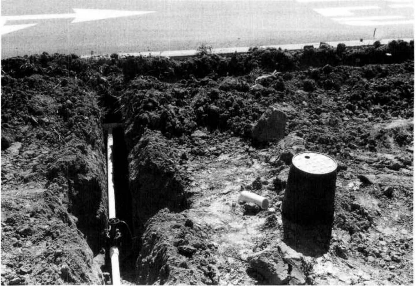
FIGURE 9.6 Mainline and automatic valve.
