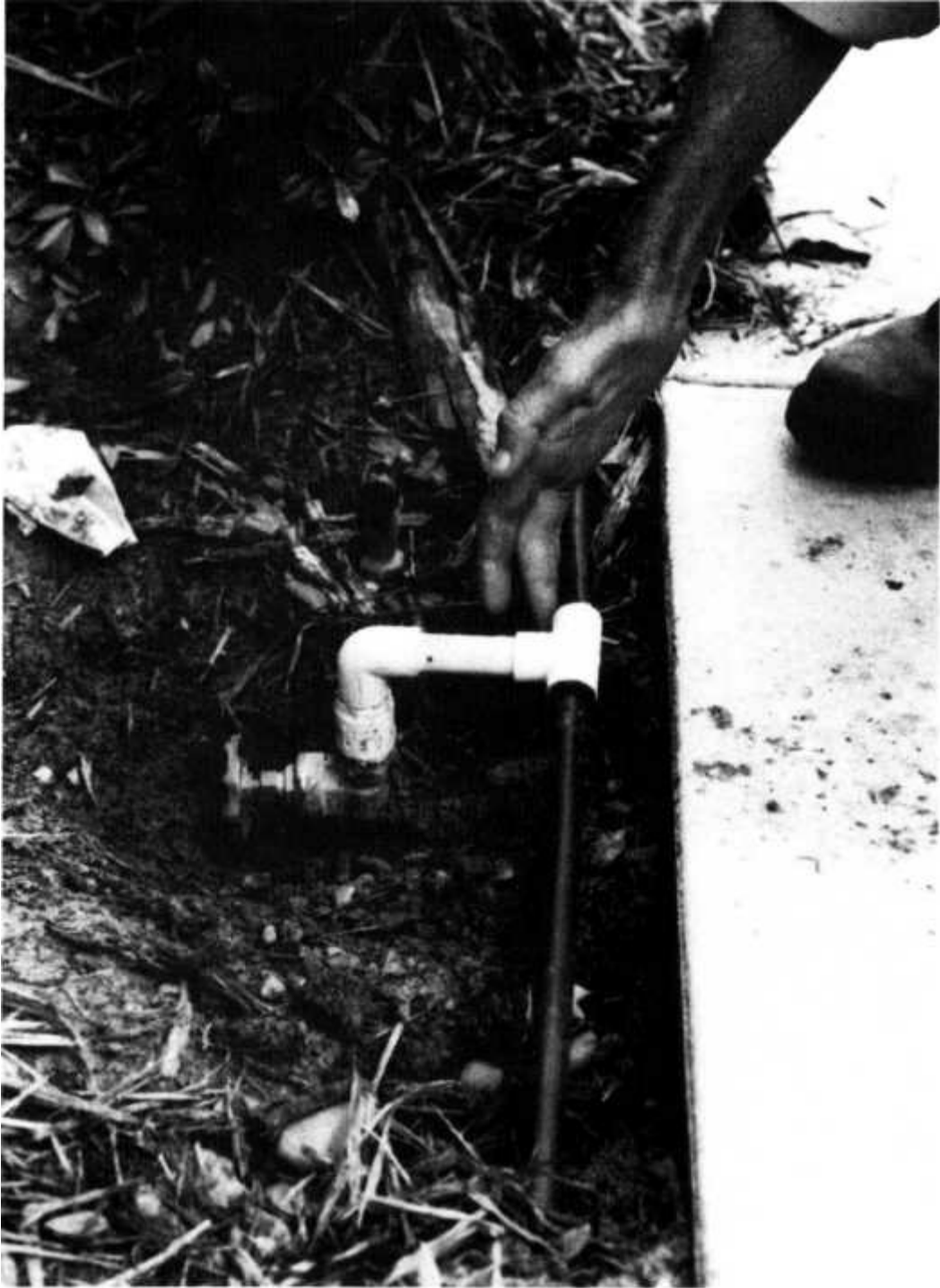
FIGURE 33. 1 Drip system connected to gate valve.
