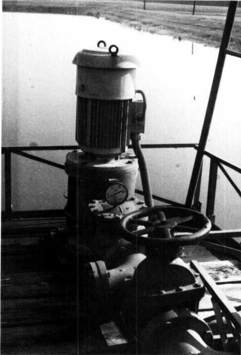
FIGURE 25.6 Vertical turbine pump at storage pond.
