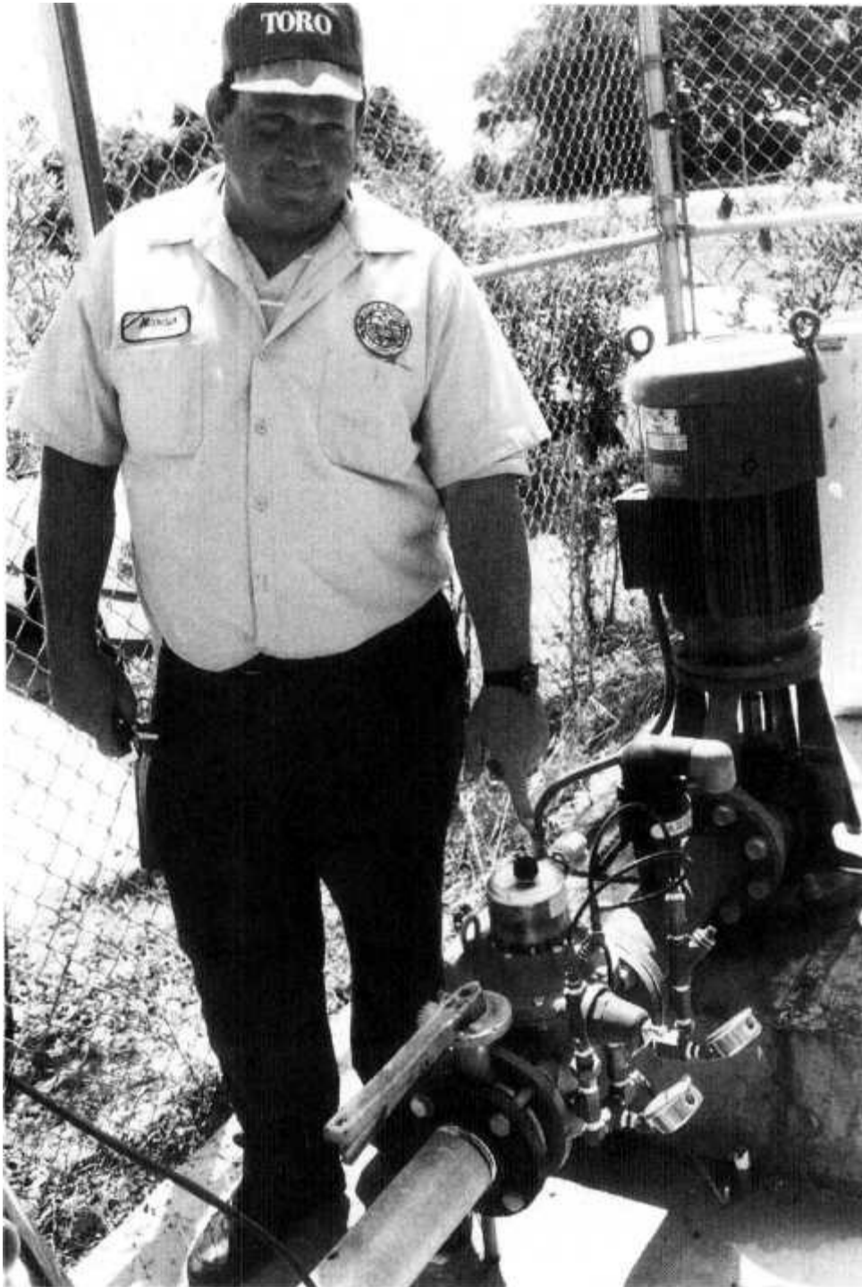
FIGURE 15. 10 Flow meter at wellwater source.
