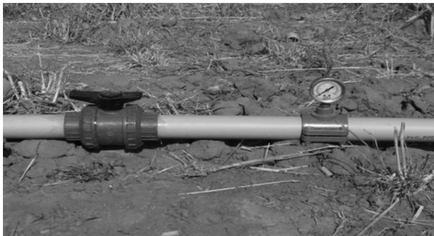
FIGURE 5.3 Control valve (Left).
