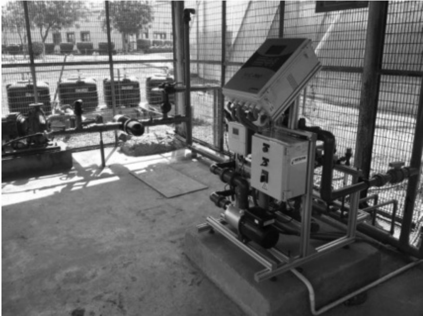
FIGURE 6.1 Drip fertigation control head.
