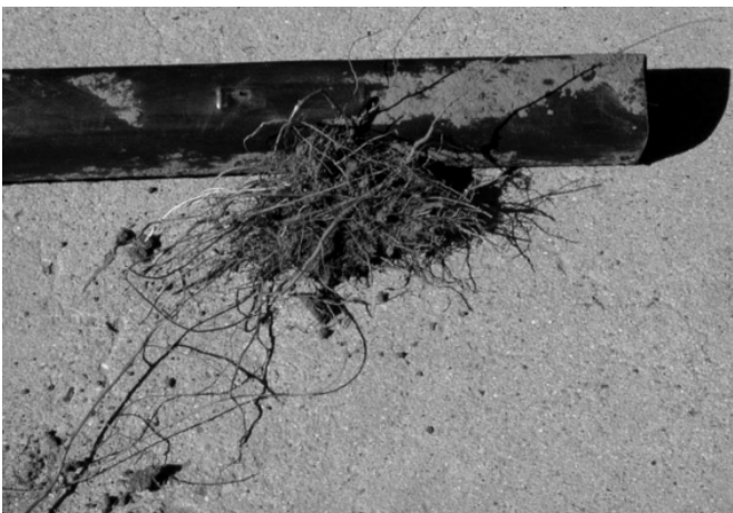
FIGURE 4 MRoots penetrating a drip emitter.
