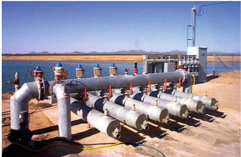
Fig. 12.30 Reservoir and pump station for center pivot farm. Cylindrical stainless steel ring filters and manifold in foreground. Motors on top of turbine pumps are seen behind manifold (Credit Paul Colaizzi, University of Arizona and USDA-ARS Bushland, Texas)
