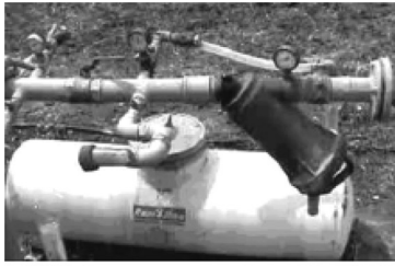
a. By-bass pressurized mixing tank.
