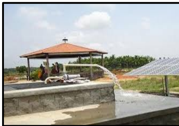
Figure 11.3 Pumping unit with solar system
