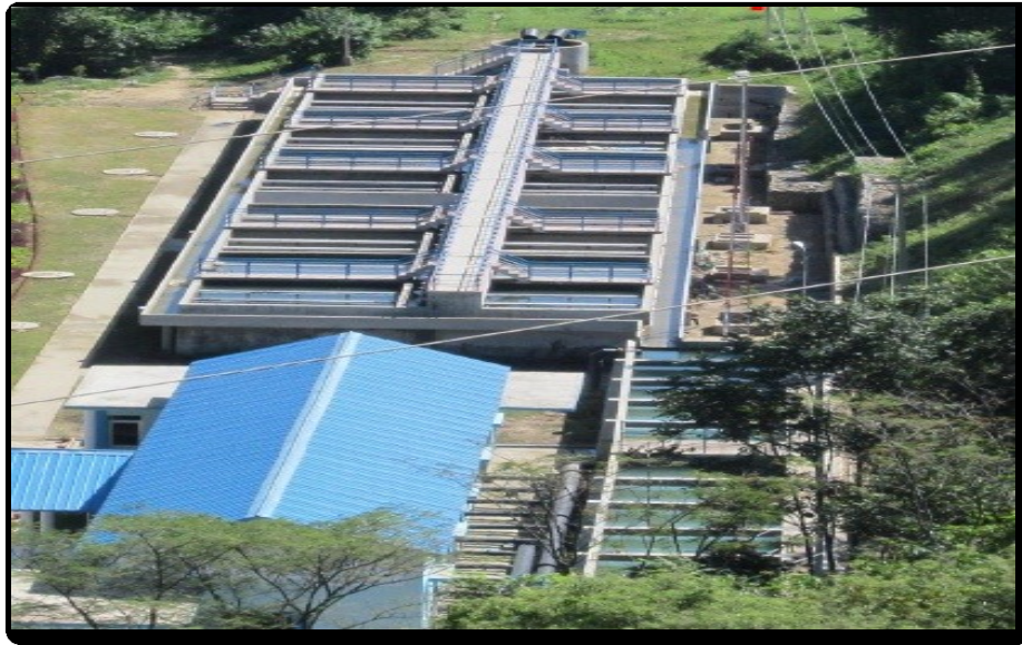
Figure 6.16 Aerial View of Tube settler type desilting arrangement provided in Balh Valley Medium Irrigation Project, HP
