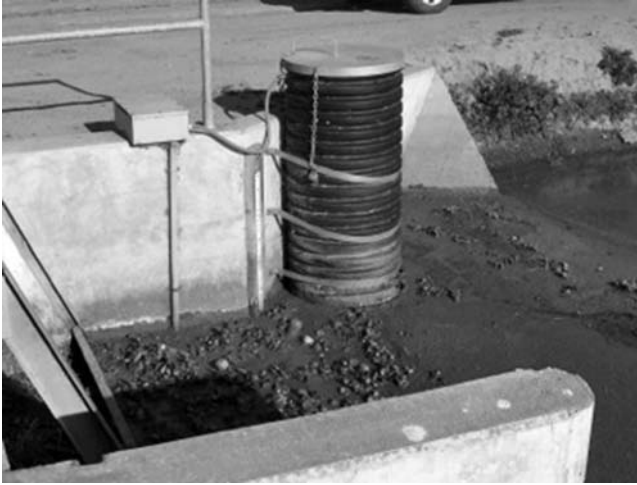
Fig. 2-35. Stilling well to the side of an automated canal structure at a point of low velocity, as seen with dry canal; no access tube is used, and a staff gauge to the side allows for easy confirmation of SCADA readings
