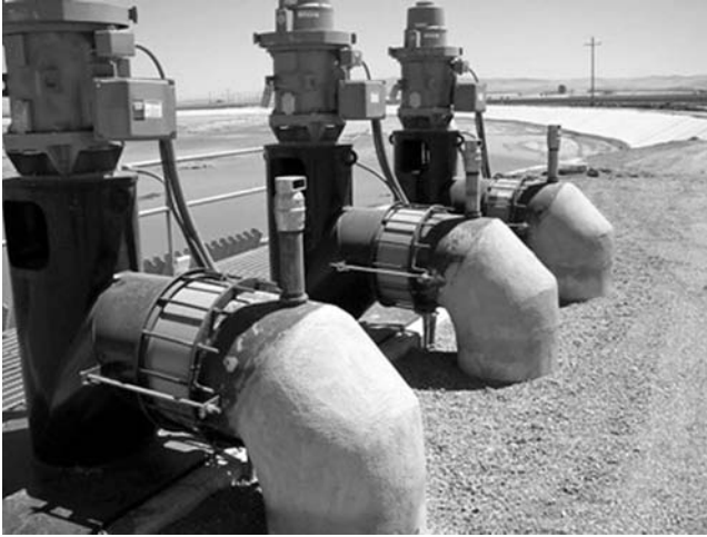
Fig. 2-51. Three identical pumps controlling the discharge from a regulating reservoir at Ingomar Reservoir, Central California Irrigation District, California, USA. The motor on one of the pumps is oversized; it is operated at a slightly higher Hz than the others at maximum speed and is controlled by a VFD controller (VFD not shown)
