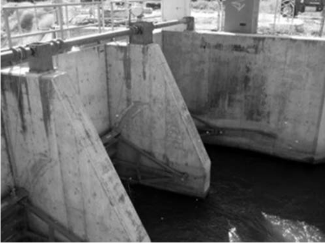
Fig. 2-14. Radial gates, downstream view with gate spools and shaft seen on the top of the structure at San Luis Canal Company, California, USA
