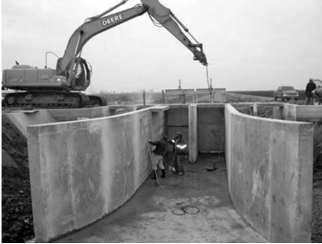
Fig. 2-46. Special entrance walls to ensure uniform velocity profiles at San Luis Canal Company, California, USA
