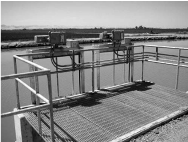
Fig. 2-26. Sluice gate actuators at the entrance to a regulating reservoir at Central California Irrigation District, California, USA
