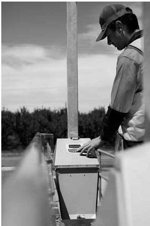
Fig. 8-15. Operators learn to set flow set points at a gate rather than to adjust the height of a gate leaf
