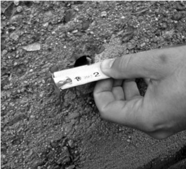
Fig. 2-34. Very small access tube entrance to a stilling well; although the hole entrance is flush with the wall (as it should be), the diameter is too small. This tube needed to be enlarged prior to automation
