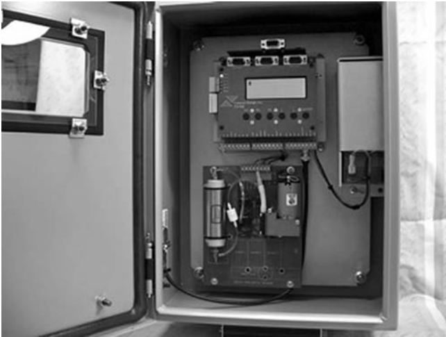
Fig. 2-31. Water level bubbler system inside an RTU panel
