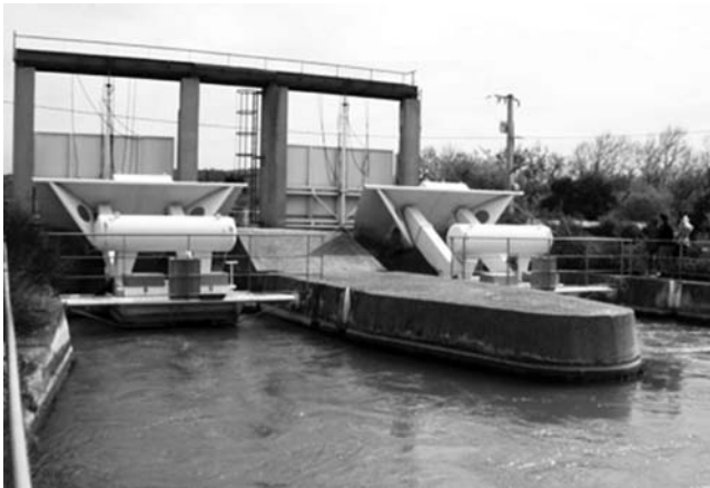
Fig. 2-21. AVIS gates at a canal in Boisgelin-Craponne, France Source: Photo courtesy of Gilles Belaud, International Center for Higher Education in Agricultural Sciences, Montpellier, France; reproduced with permission
