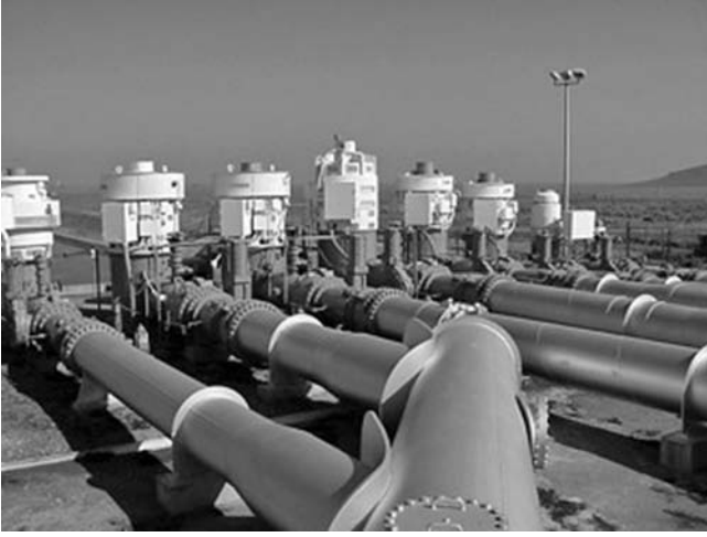
Fig. 2-49. Multiple pumps in parallel at Berrenda Mesa Water District, California, USA
