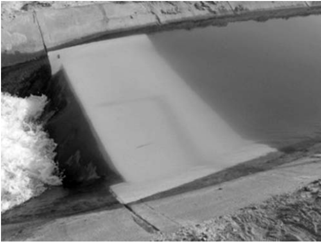
Fig. 2-41. Painted broad-crested flume to minimize algae growth; flow rate capacity is 3 CMS (100 CFS) at Imperial Irrigation District, California, USA
