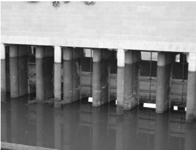
Fig. 2-10. Multiple parallel sluice gates of 1.3-m width each (canal is de-watering) at the Modesto Irrigation District, California, USA. The sluice gates control the vertical opening of a hole in the bottom of the concrete structure to minimize the height of the gate
