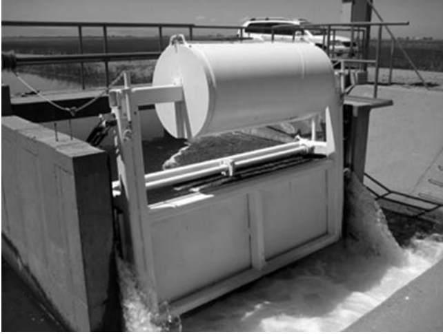
Fig. 2-25. ITRC flap gate at San Luis Canal Company, California, USA
