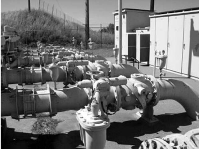
Fig. 2-48. Modulated valves (followed by check valves) on the discharge of each pump at Orland-Artois Water District, California, USA
