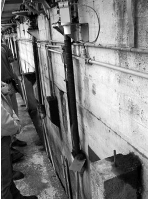
Fig. 2-37. Ultrasonic sensor (top center) pointed down to flat horizontal plate (bottom center) attached to sluice gate at Alta Irrigation District, California, USA
