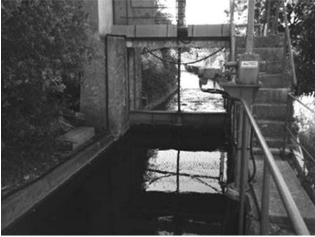
Fig. 2-6. Automated vertical sluice gates of Left Bank Gignac Canal, France Source: Photo courtesy of Gilles Belaud, International Center for Higher Education in Agricultural Sciences, Montpellier, France; reproduced with permission
