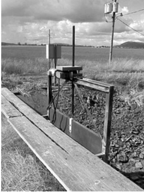
Fig. 2-11. Automated sluice gate in a small canal at Tulelake Irrigation District, California, USA
