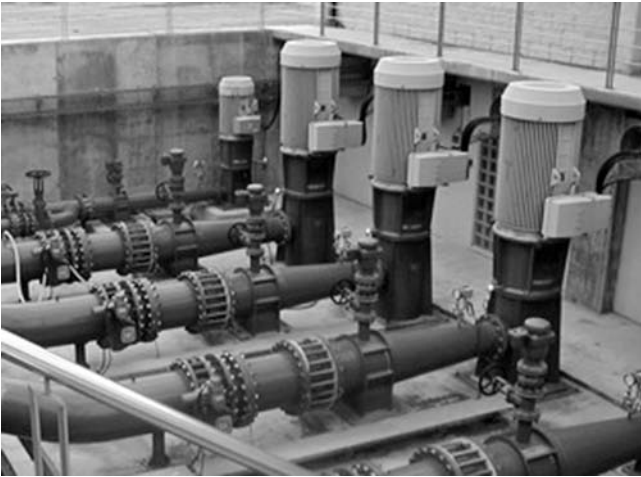
Fig. 2-50. Pumping station at Torres de Segre, Spain Source: Photo courtesy of Gilles Belaud, International Center for Higher Education in Agricultural Sciences, Montpellier, France; reproduced with permission
