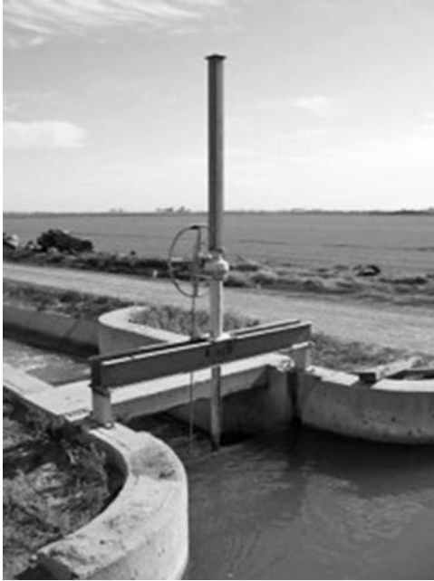
Fig. 2-9. Manual sluice gate with large hand wheel and gear box for a small canal at Imperial Irrigation District, California, USA. The stem is covered to avoid dust accumulation. The top boards can be removed so that the sluice gate can also have an overflow weir action
