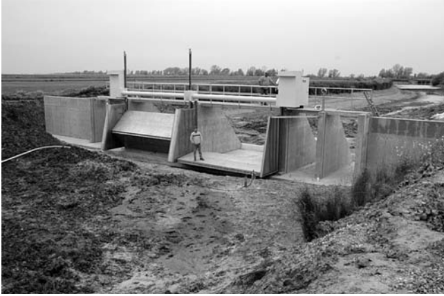
Fig. 2-5. Langemann gates by Aquasystems 2000, upstream view. This configuration hinges on the bottom and middle. All movement of the weir crest is vertical, rather than having an arc as in the previous three gate configurations shown
