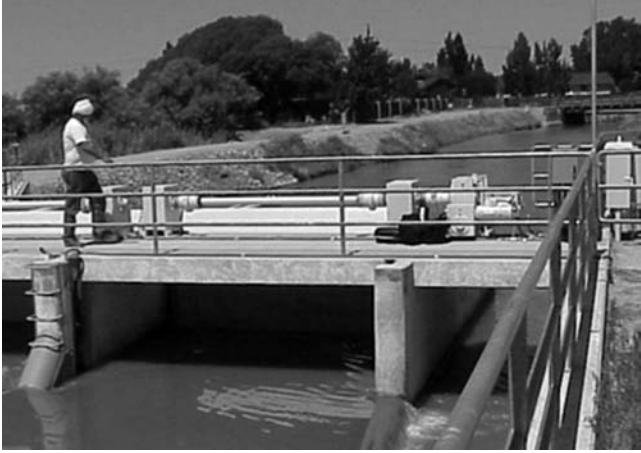
Fig. 2-27. Actuator (on right side) for a radial gate on the Government Highline Canal, Grand Junction, Colorado, USA. Note the high silt content of the water
