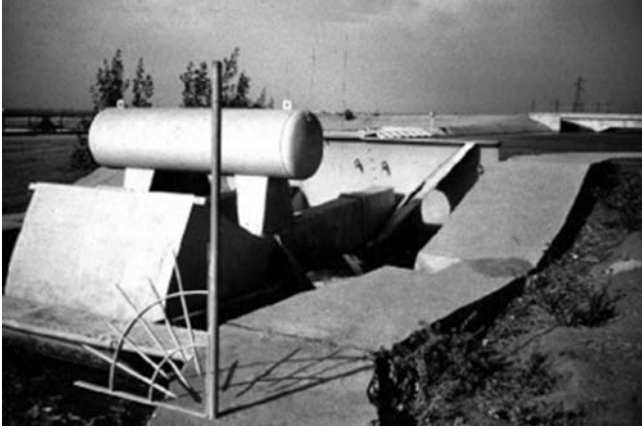
Fig. 2-19. AVIS gate at the Doukkala Project, Morocco
