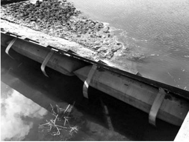
Fig. 2-3. View from downstream of an Obermeyer gate with no flow in late summer at Walker River Irrigation District, Nevada, USA. Air-inflated pillows control the angle of the rigid gate leaf opening. The gate leaf hinges at the bottom, on the floor. These gates are primarily used for coarse water level control in rivers or on dam spillways because no structure is required above them. However, monitoring and control of precise leaf positions has proven problematic in some projects
