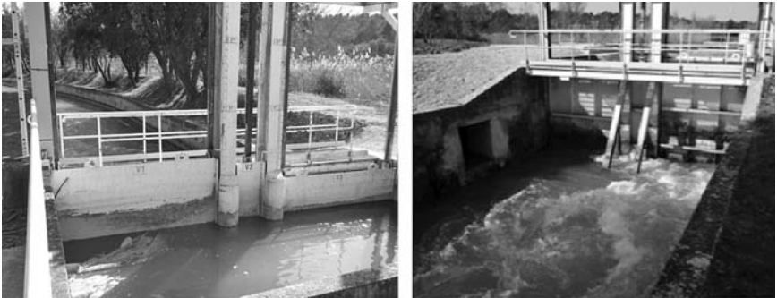
Fig. 2-7. Automated vertical sluice gates in parallel at the Canal de Marseille, France
