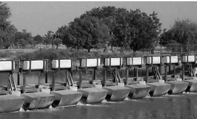
Fig. 2-24. Begemann gate with a special "Vlugter" back to allow submergence at Hadejia Valley Irrigation Project, Nigeria Source: Photo courtesy of Xavier Litrico, Centre R&D de Lyonnaise des Eaux à Bordeaux, France; reproduced with permission
