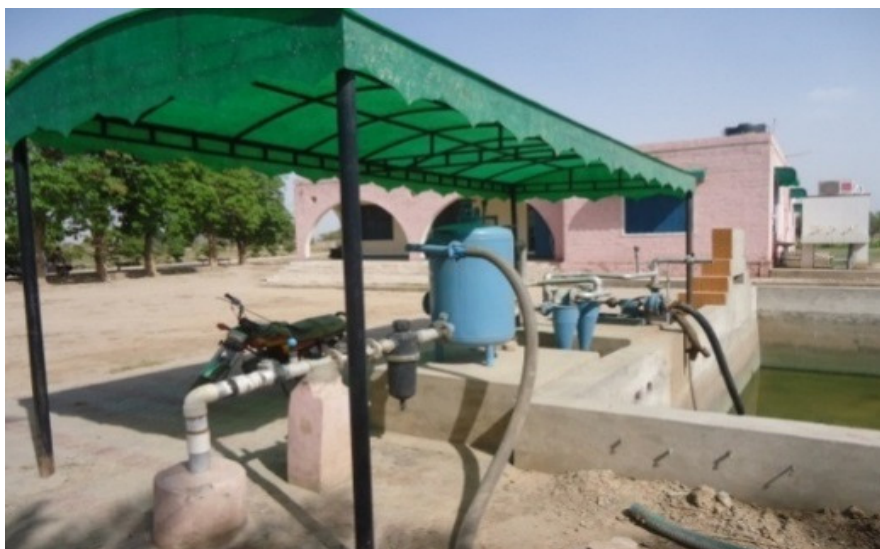
Fig. 15.5 Drip Irrigation System Power Unit installed at PARS
