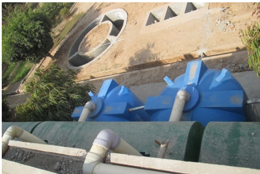
Fig. 15.10 Rainwater Collection Setup along with Storage Tank and Recharging Well
