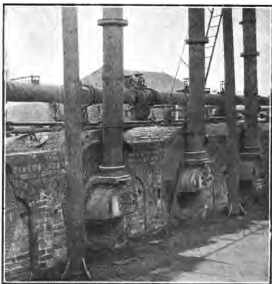
Fig. 94.—Front of Boilers Fired with Blast-furnace Gas.
