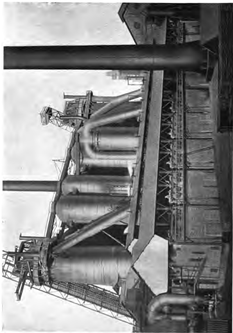
Eighteen Babcock & Wilcox Boilers, each of 3,140 square feet heating surface, arranged for firing with blast furnace gases and coal.
