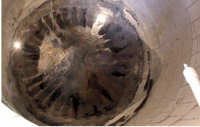
Figure 2.1b The raceway after a blowdown and nitrogen quench (courtesy John Ricketts)
