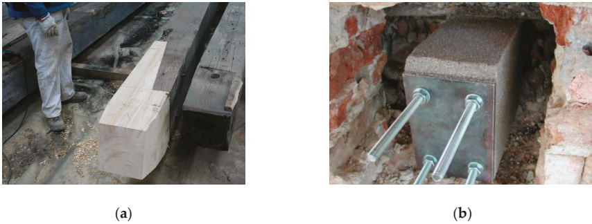
Figure 13. Re-construction of the beam ends: (a) stainless steel reinforced wooden prosthesis; (b) detail of the stainless steel reinforced epoxy prosthesis [48].
