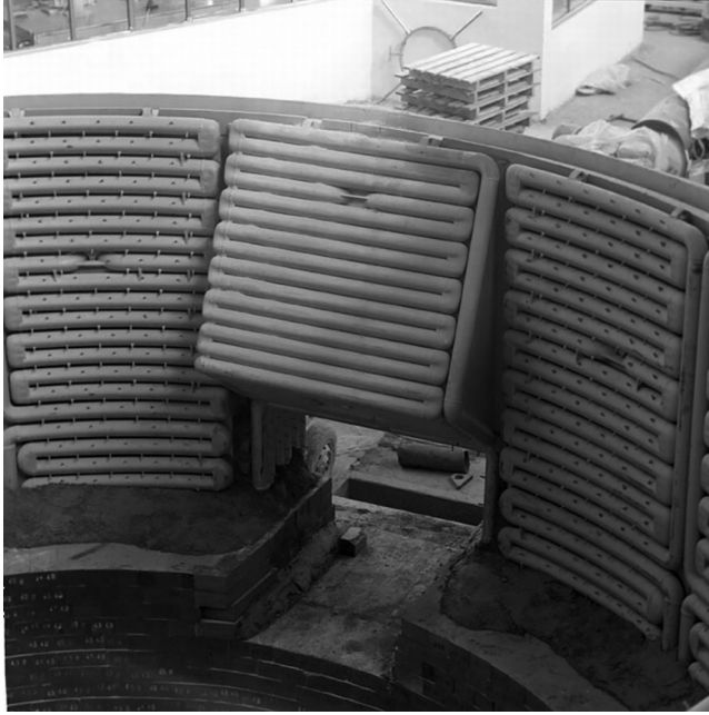
FIGURE 3.29 View of water-cooled panels in the furnace along with a panel above the main door [1]. (Advertising materials (corporate brochure) of the SMS group GmbH (formerly SMS Siemag AG) – with permission.)
