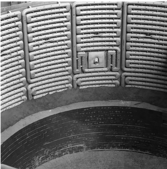
FIGURE 3.28 View of water-cooled panels in the furnace along with a burner-cooling panel [1]. (Advertising materials (corporate brochure) of the SMS group GmbH (formerly SMS Siemag AG) – with permission.)
