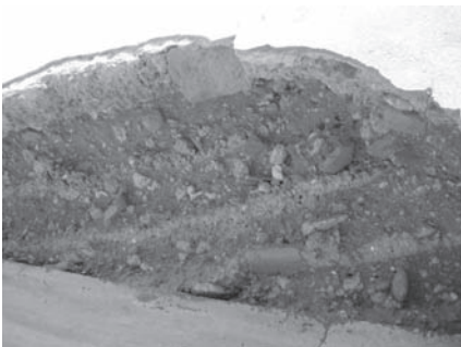
Figure 13. Interior of a rammed earth wall with facing made of bricks and lime mortar in Koléa. (Alliche. S., 2011).
