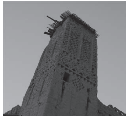
Figure 7. Detail of one adobe decorated tower of Bou Taghrar's Kasbah. Picture: Alberto Montiel Lozano.
