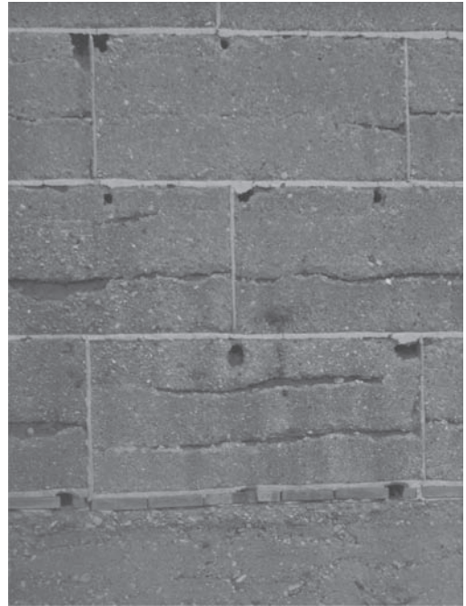
Figure 2. Rammed earth wall with gypsum-reinforced joints in order to protect these weaker points from atmospheric agents (Cristini).
