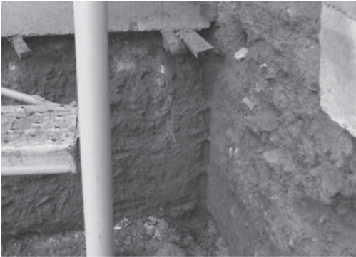
Figure 5. On centre of this photo, it can be seen in a corner of the rammed earth wall, the negative of the five wooden overlapping planks from the original formwork.
