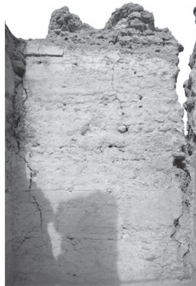
Figure 2. Tower number 2 showing formwork marks.
