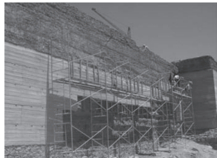
Figure 3. Working zone on southwest wall. Notice the lack of space for scaffolding mount and for machinery work. See the small crane, working from the interior of the wall.
