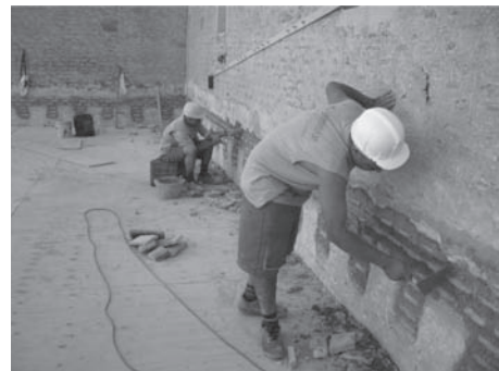
Figure 7. Reintegration of the rammed-earth wall in those areas with hollows of the former supports of the wooden beams.
