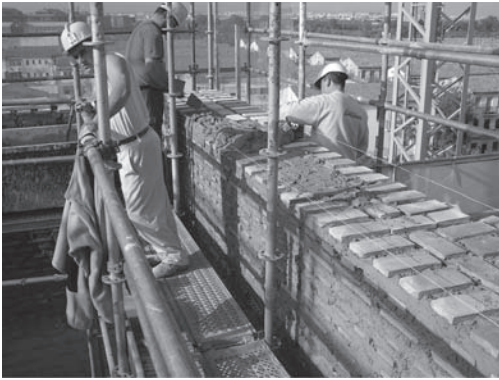
Figure 11. Image of the process of placement of the brick course in the brickwork of the fourth tower during the reconstruction process.
