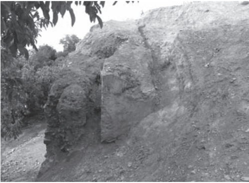
Figure 2. South end of the wall before the intervention, seen from the south.
