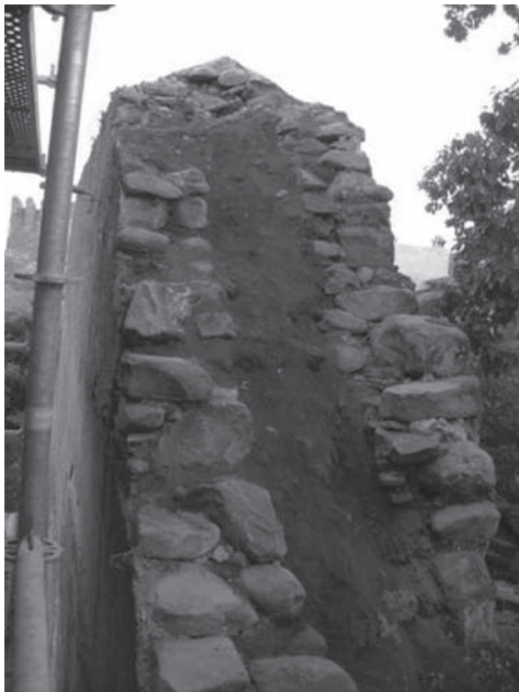
Figure 1. Section of the wall at the rebuilt in 1942 by the Dirección General de Regiones Devastadas.
