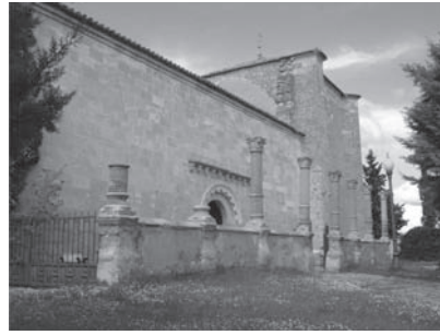
Figure 1. Church of 'San Nicolas de Bari'. State before last intervention. The stone facing from 1965, covering the original rammed-earth wall, is visible. (Pinés & Jové-Architects).
