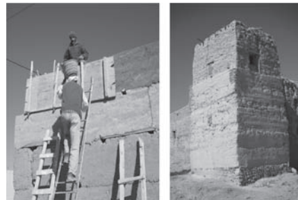
Figure 6. Left: foundations, rammed earth wall and adobe. Right: executing the rammed earth wall.
