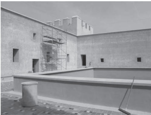
Figure 12. Image from the courtyard during the reintegration and reconstruction works of the fourth tower.
