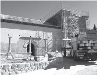
Figure 2. Restoration work. Recuperation of the rammed-earth wall built on top of the remnants of the 13th century wall (Pinés & Jové-Architects).
