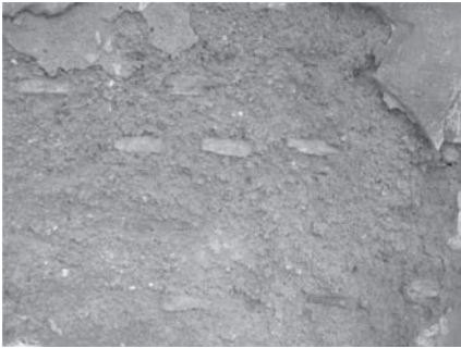
Figure 12. Rammed earth wall with facing made of fired bricks and lime mortar in Koléa. (Alliche. S., 2011).
