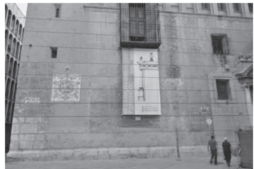
Figure 8. Superimposition of the rammed earth wall courses over a photograph of the southern façade.
