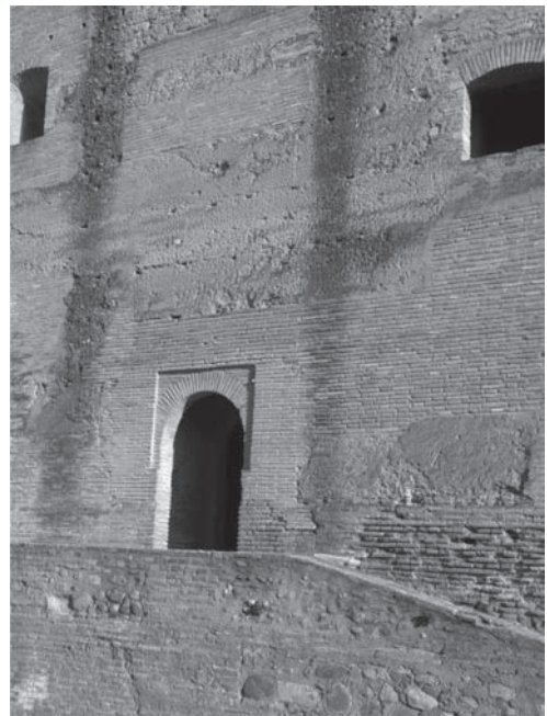
Figure 7. Cavity of the door of the main Tower in the interior with diverse repairs.
