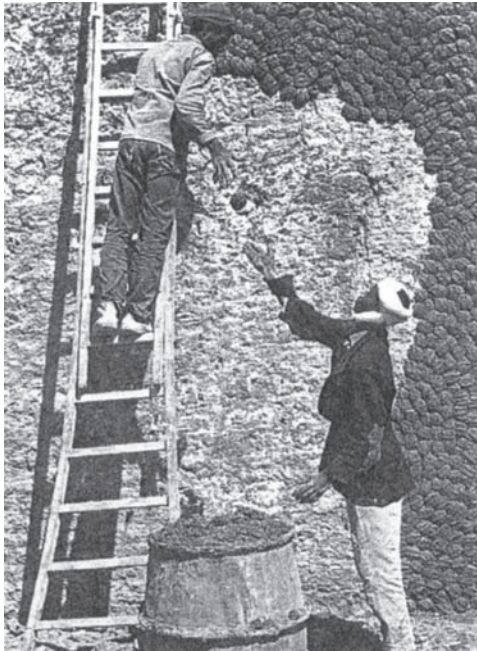
Figure 9. The finish coat. S.Haoui in “For the preservation of the architectures Ksouriennes in raw earth. Example ksar of Timimoun, Algeries”.
