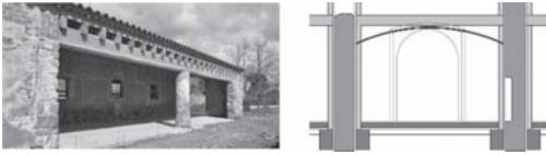
Figure 4. Restoration of Can Falguera. Functional replacement of rammed earth wall. Architect: David Lladó.
