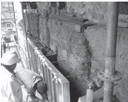
Figure 5. Restoration work on the rammed-earth walls. Church of 'San Nicolas de Bari'. (Pinés & Jové-Architects).
