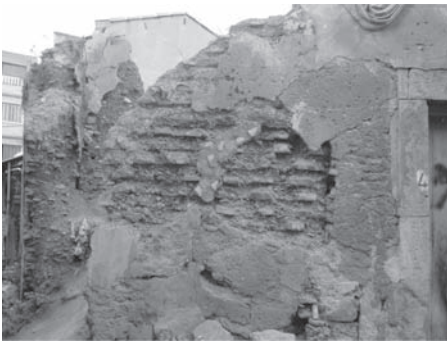
Figure 9. Exterior walls are partially collapsed. (Chennaoui. Y., 2007).
