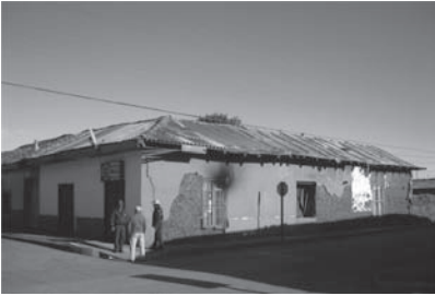
Figure 6. Damages example in Cobquecura (Baglioni E., 2011).
