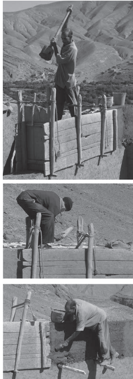
Figure 5. Ramming and finishing a wall section. a. ramming b. hand-ramming c. finishing ( takhbat ).
