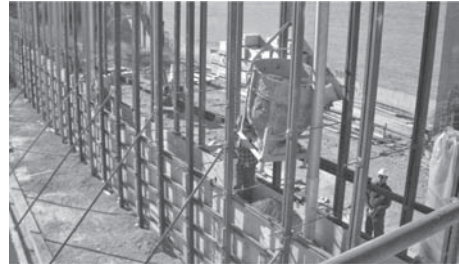
Figure 6. Pouring the earth once placed of the formwork. Autor: Vier arquitectos SLP.
