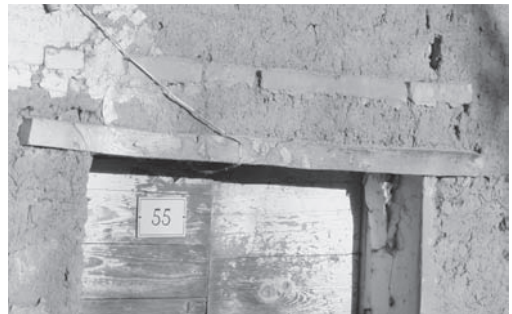
Figure 4. Moscufo, rural building in Contrada Colle di Giogo: horizontal rows of baked bricks.
