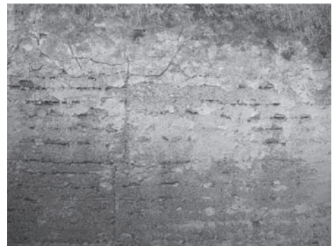
Figure 7. Trace of the formwork side on a wall face with alternating fired brick and lime mortar. (Alliche, S., 2011).
