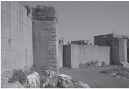
Figure 6. General view of the Niebla city walls after restoration (Huelva, Spain) (Vegas & Mileto).
