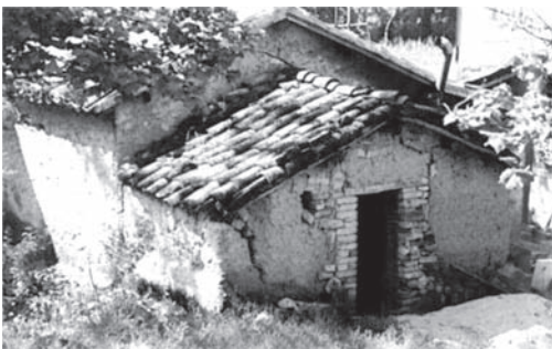
Figure 5. Manoppello, rural building in Locality La Fornace: door reinforced with baked bricks.
