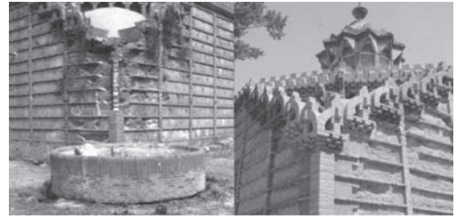
Figures 5-6. Previous and later view of the rammed earth restoration carried out by architect and Professor Joan Bassegoda Nonell, Gaudí Chair director until the year 2000. Pictures: Joan Bassegoda.
