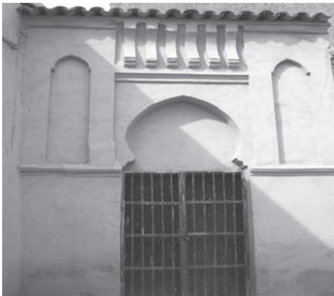
Figure 4. The façade of house with the earthen architecture, Ksar of Tiout (Mebarki 2009).
