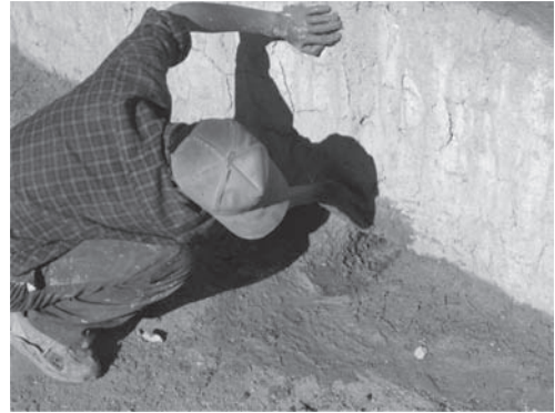
Figure 6. Creation of the improved joint using markallak mixture and finely chopped straw with stone joint cover.
