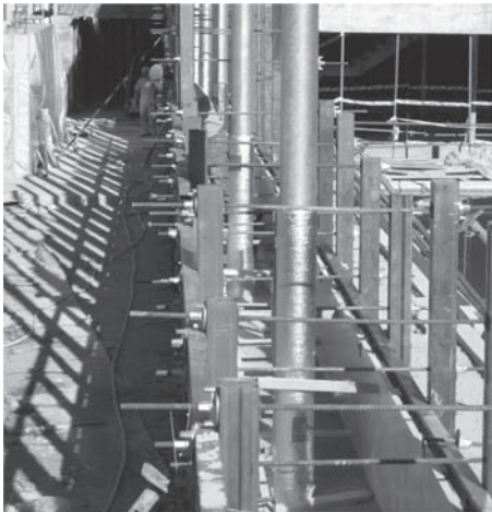
Figure 9. Galvanized steel tube with elastic joint inside the wall. Autor: Vier arquitectos SLP.
