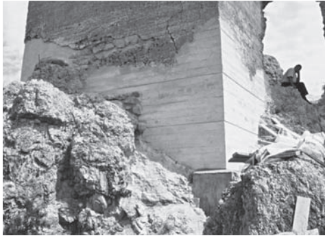
Figure 3. Siyasa. Tower struck by lightning.
