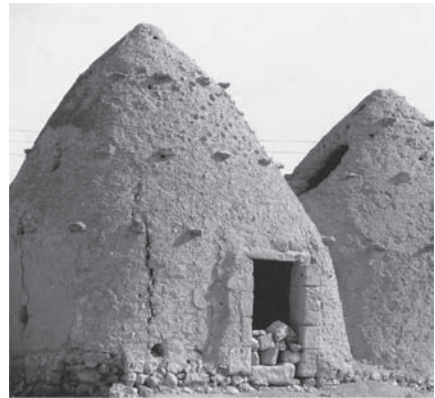
Figure 4. Domes in a poor state of conservation (autor: Dipasquale, L. 2009).
