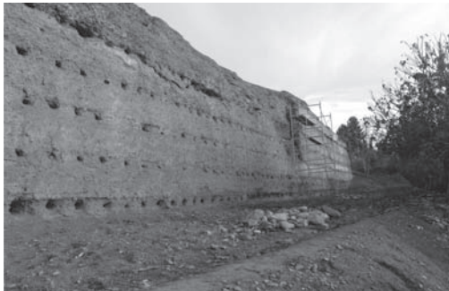
Figure 5. The wall before the intervention. The slope conceals the height of almost two rammed earth sections.
