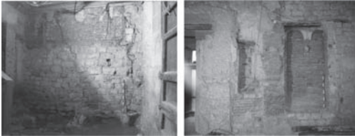
Figure 11. (left) 14th century rammed earth, perpendicular wall to Ripoll facade. Figure 12. Rammed earth from the 14th century, main floor. Facade Hostal En García. Romantic garden. Pictures: ATICS.
