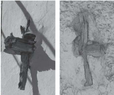
Figure 3. Reeled brace. View from the outside. Cut-out in the axis of the brace. Brace, pin and wedge. Half-lap joint assemble. Brace, pins and iron wedges.
