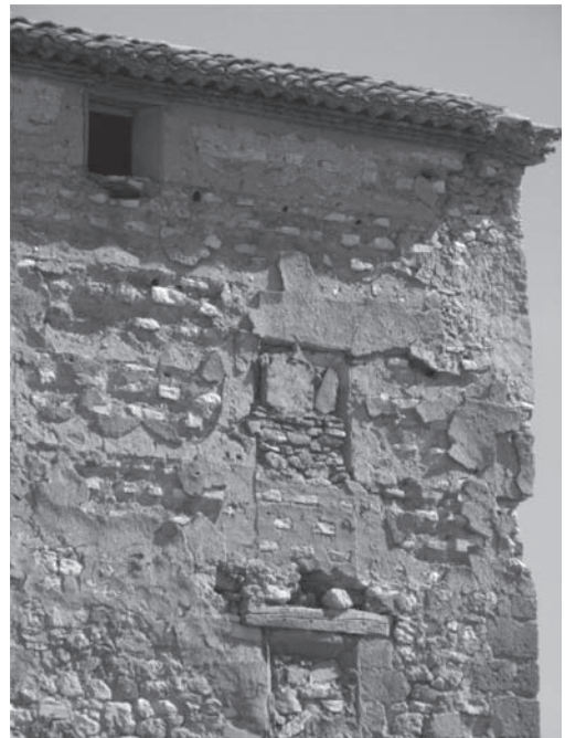
Figure 10. Example of a Valencian rammed earth wall with brenças and rafas damaged by weathering in a gradual process of erosion and loss of material (Vegas & Mileto).
