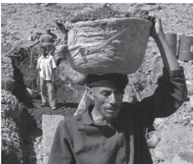
Figure 6. Forefront: Mr. Oukhom hauling the earth in a basket. Bottom: workman in the ditch.
