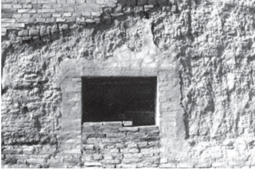
Figure 11. San Omero, building in Locality Case Alte: the original earthen building is increased by a brick raising.
