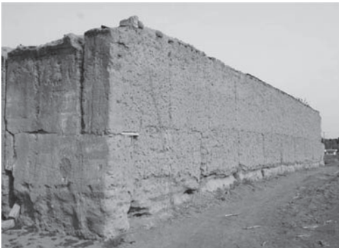
Figure 5. The South façade, to the left of the picture, does not present insects’ boreholes, while the East is crammed with them. Also to be noted is the weathering on the base of the walls by the lack of foundations and plinths.
