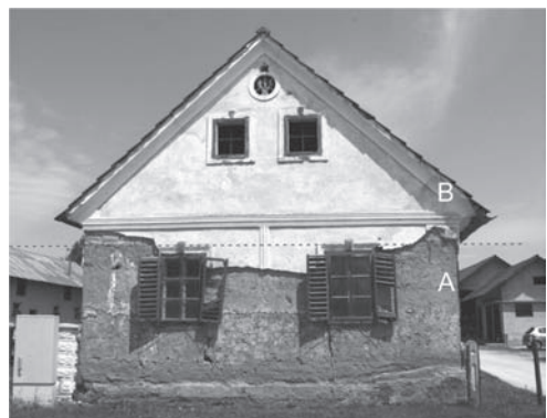
Figure 1. A house in the village of Bukovci: walling construction of rammed earth is exposed. A—wall made of rammed earth; B—gable end wall made of bricks.
