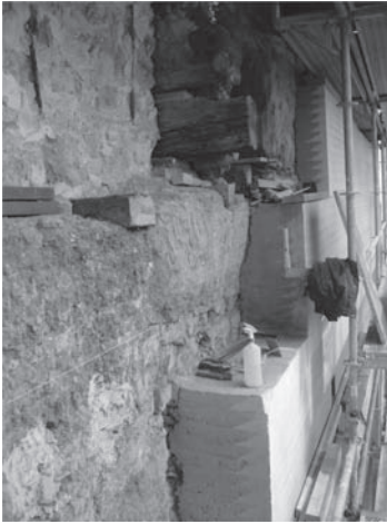
Figure 7. Restoration work on the rammed-earth walls Church of ‘San Nicolás de Bari’. (Pinés & Jové-Architects).
