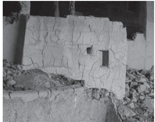
Figure 1. The cracking of the core of the walls suggests that the soil that was used for the construction was excessively moist. Pre-Hispanic houses at El Embudo Caves , Chihuahua, Mexico.
