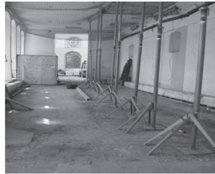
Figure 4. Current situation of the rammed earth floor, northern pavilion and northern oval house, Belvedere Orangerie, September 2011.
