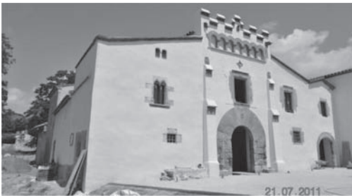
Figure 14. Restoration of Can Falguera. Facade rendered with lime mortar. Architect: David Lladó, DAC Arquitectura.
