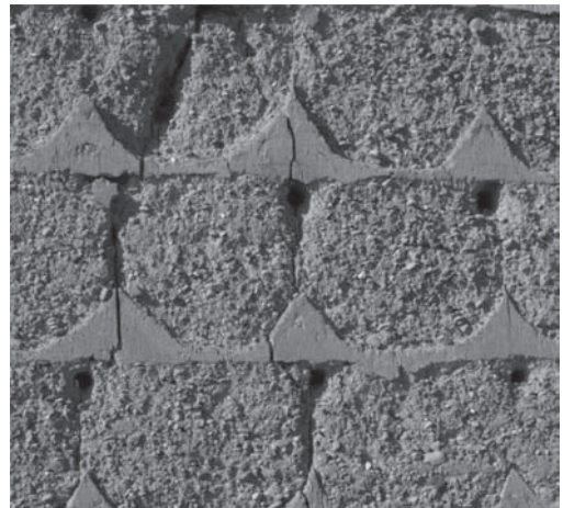
Figure 3. Detail of a rammed earth wall with brencas or undulated gypsum reinforcement (Vegas & Mileto).
