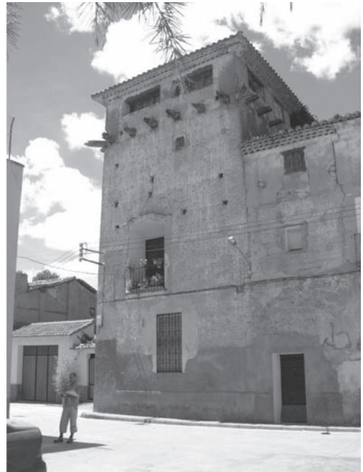
Figure 5. The tower at Torrealta, a typical case of Valencian rammed earth wall bonded in mass and reinforced on the outside with stones, visible on the finished surface (Vegas & Mileto).
