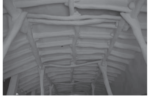
Figure 15. Example of contemporary house in Tucume, Chiclayo Province. A Guarango structure, with daubed earth and straw layers, lately whitewashed. (Cristini & Ruiz Checa).
