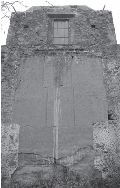
Figura 4. Rammed earth wall with buttress made of volcanic stone and boulders. Chapel of Santa Ana. Calpan, Puebla.
