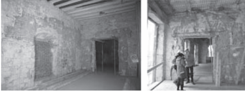
Figure 9. (left) 15th century rammed earth, facade main floor. Figure 10. (right) 16th century rammed earth. Main floor. Perpendicular wall to the romantic garden. Pictures: S. Bestraten–E. Hormías.
