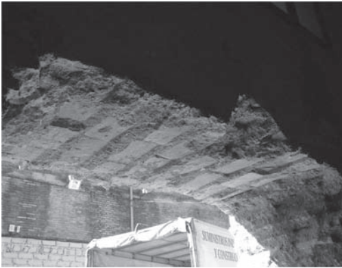
Figure 5. Hollow horizontal section done in the rammed-earth wall of the Alaquàs castle where can be seen the traces of the bricks internal disposition.
