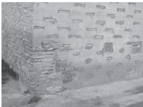
Figure 5. Fake tapia valenciana wall: new wall coated with a rendering into which the bricks are inserted (Alquería de Pinohermoso, Burjassot, near Valencia).
