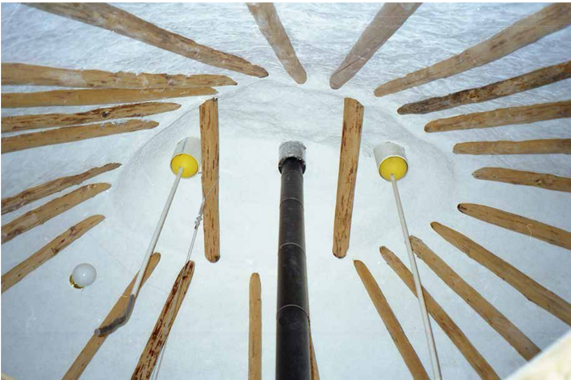
Fig. 11.4: Exhaust ventilation in this large dome was provided by two vents fitted with tetherball closures and long handles to remove or insert them. The central stove pipe was fitted with a zero clearance pipe, similar to that in Figure 11.3.
