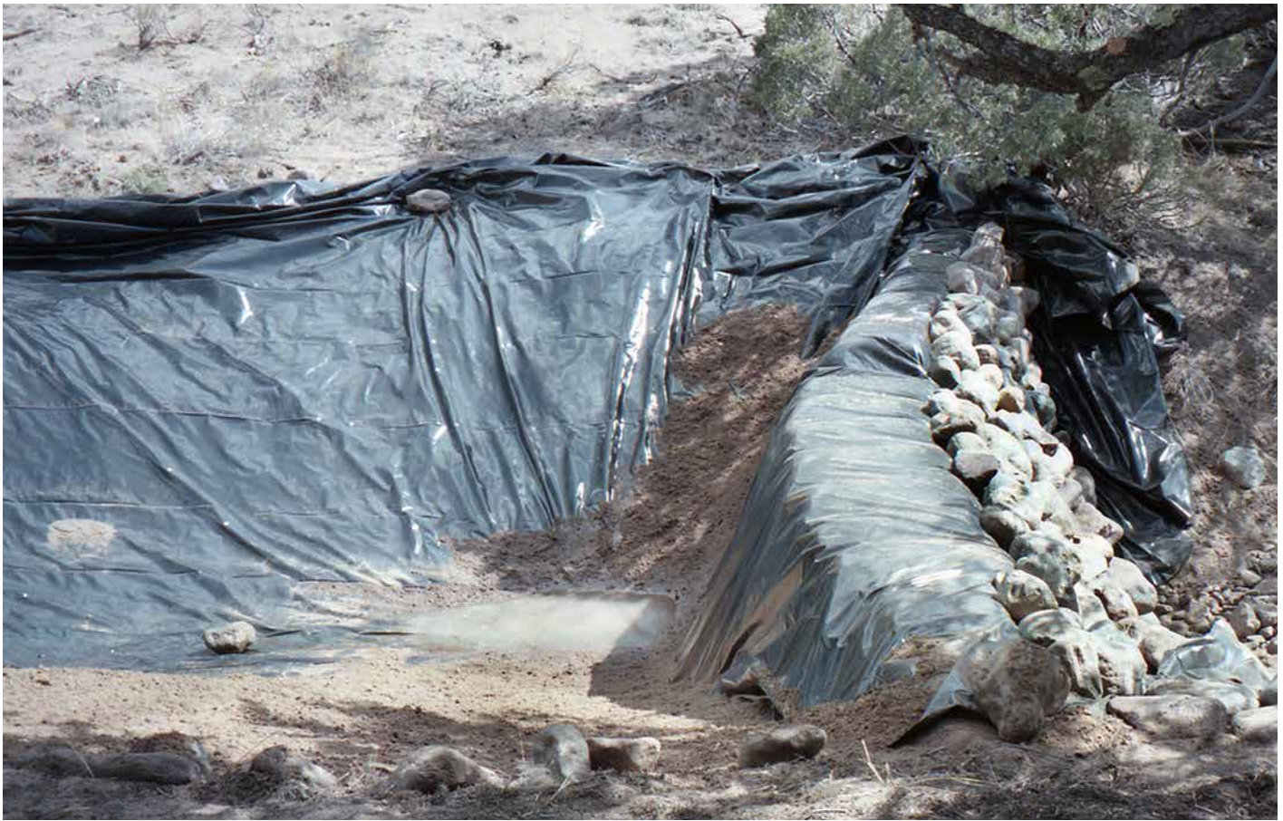
Fig. 16.3: This shows how the earthbag dam was lined with heavy plastic completely over the dam and down the back and then protected with stones on the backside. CREDIT: KELLY HART
