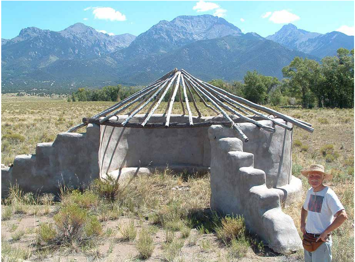
Fig. 4.6: This circular vertical walled structure was built from earthbags filled with unstabilized sand, but it has stood the test of time.
