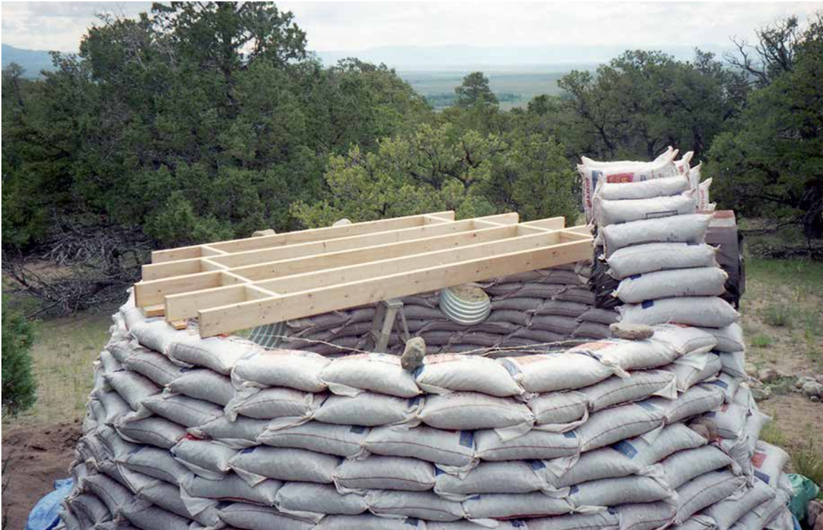
Fig. 8.3: Joists for a partial loft in this small dome were simply placed on the bags and shimmed to bring them level. Earthbags were then inserted in the spaces between them in order to continue building the wall.
