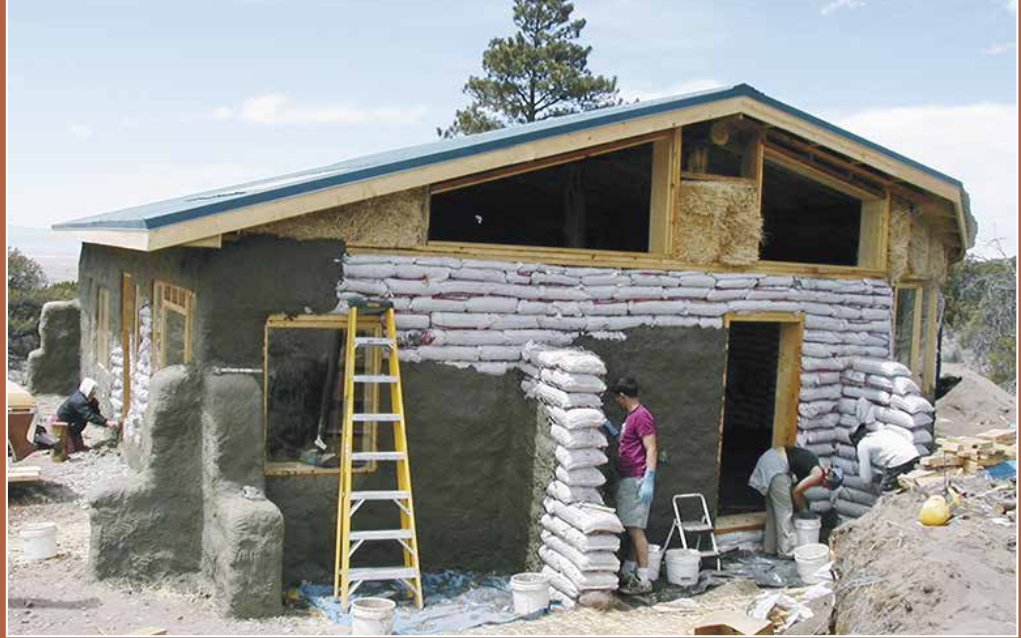
Baraka Burrill's house is under construction in the Colorado mountains; the author assisted with the design. CREDIT: KELLY HART
