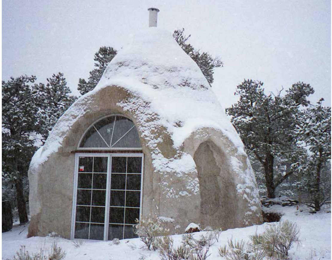
Fig. 14.1: This domed bedroom was completed to this point when construction ceased for the winter. The doorway into the rest of the eventual house is on the right; it was temporarily bagged up and plastered to keep all the walls in good shape until construction resumed.
