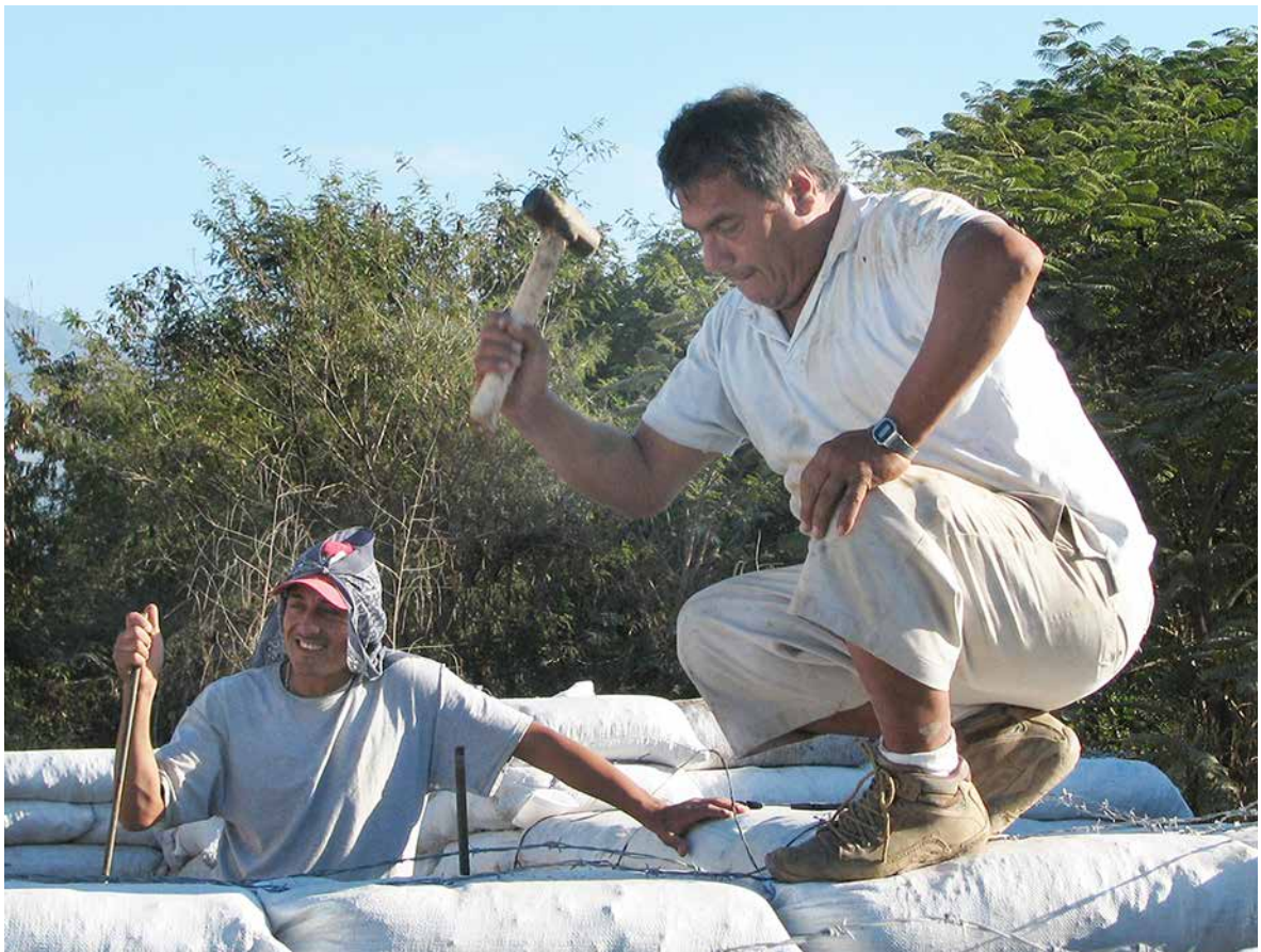
Fig. 7.9: A section of rebar is being pounded into this wall to help reinforce it.
