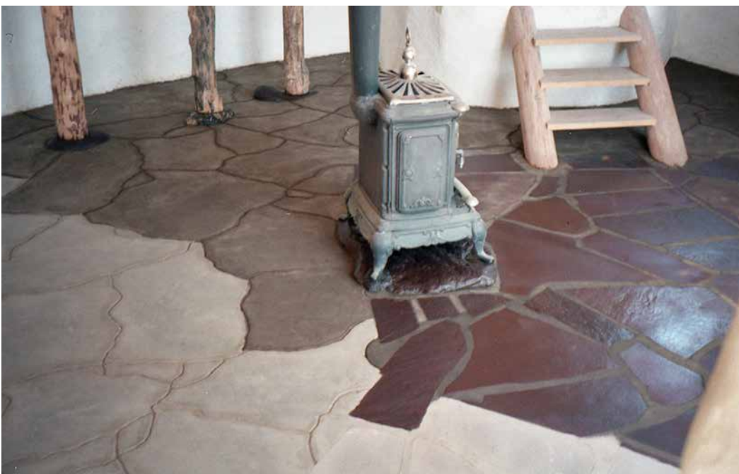
Fig. 10.3: Fresh linseed oil has just been applied to this floor. On the right is flagstone and on the left is adobe that was scored to make it resemble stone. CREDIT: KELLY HART
