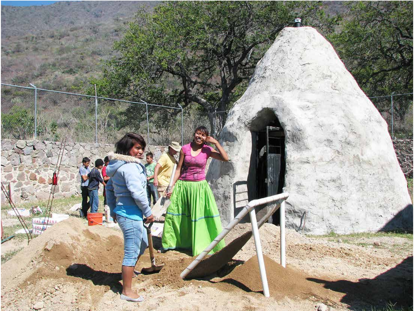
Fig. 3.1: This small earthbag dome under construction in Mexico was plastered on the exterior with cement-based stucco that had a latex additive to make it more waterproof. In addition, it was painted with a couple of coats of water-impermeable roof paint. CREDIT: KELLY HART
