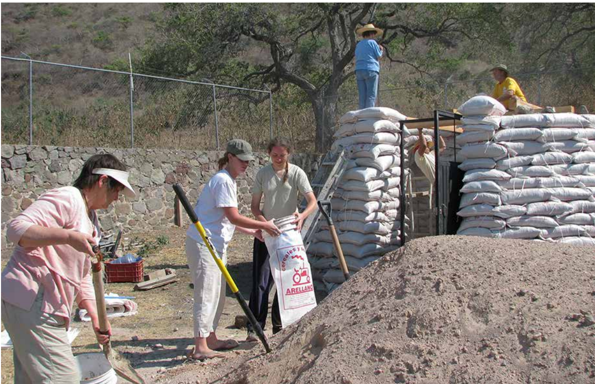
Fig. 7.1: The fill soil for this dome project was brought to the site by dump truck and placed near where the work was being done.
