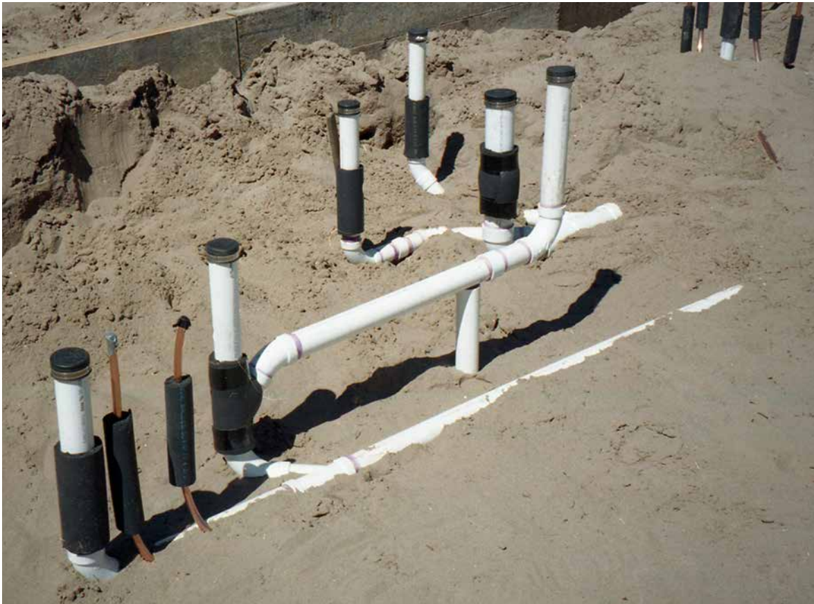
Fig. 10.1: This is an example of how plumbing drains and supply lines might be arranged prior to pouring a concrete slab floor.
