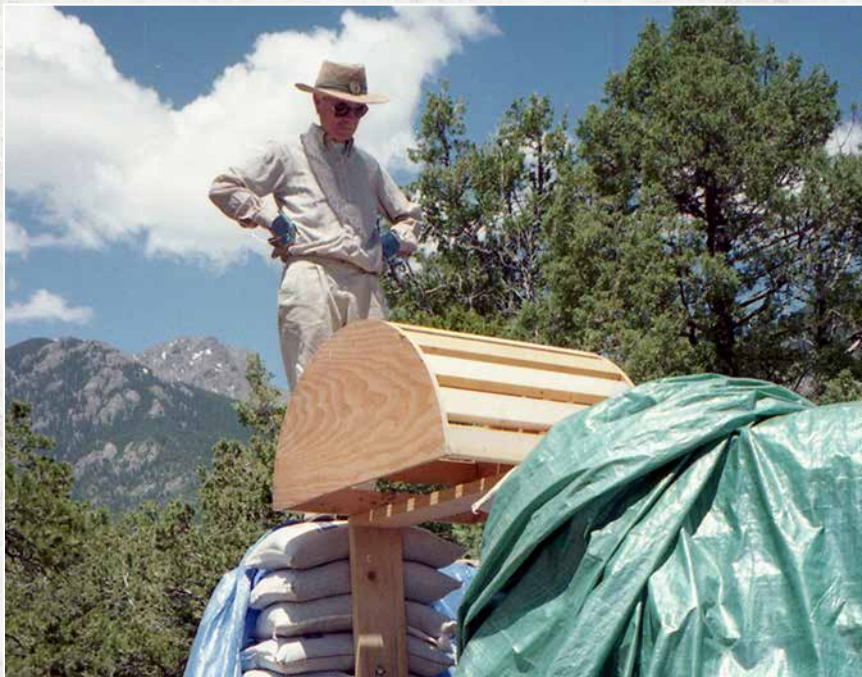
Fig. 5.4: This 3-foot (91 cm) arch form is ready for bags to be placed over it.
