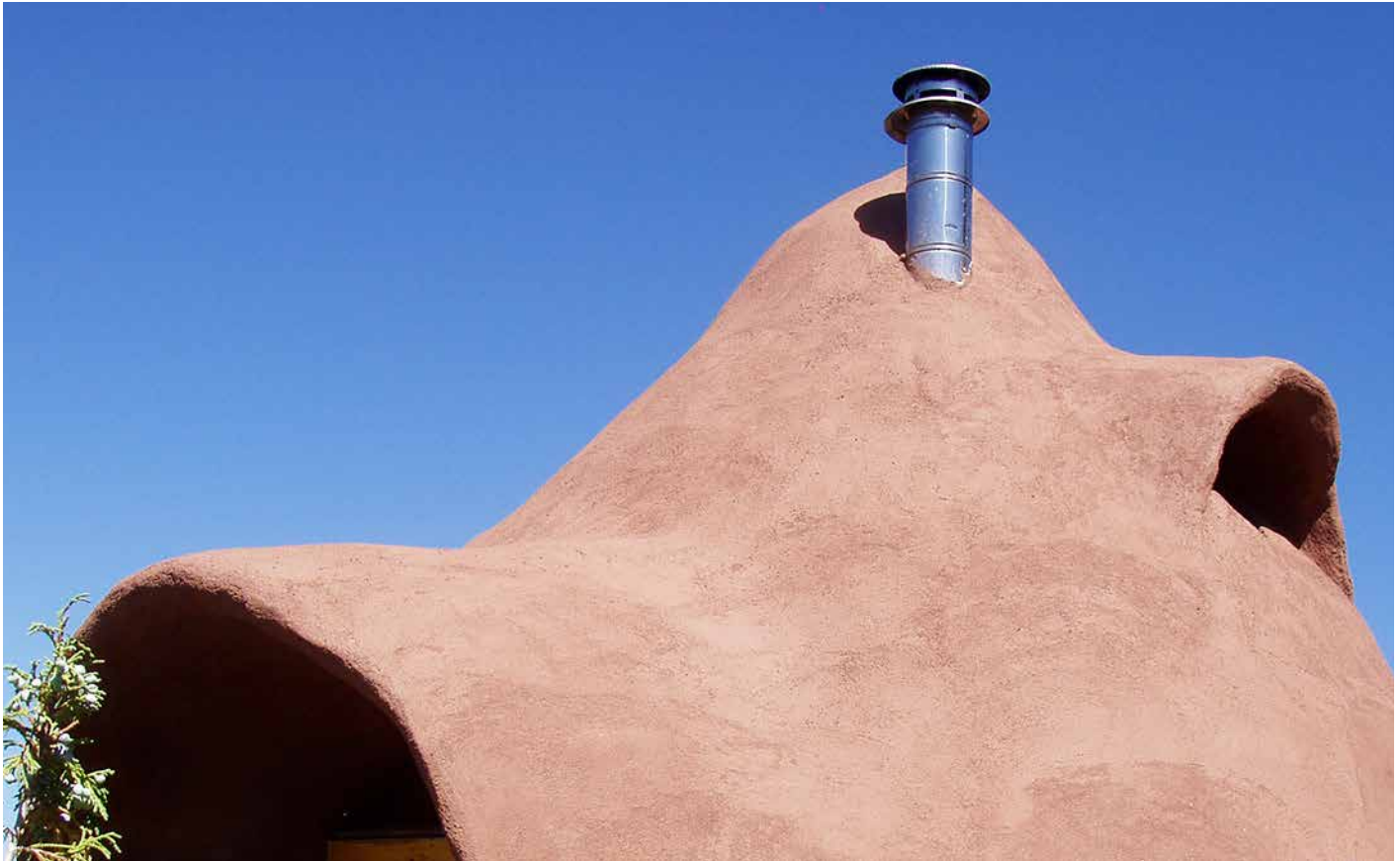
Fig. 11.3: A zero clearance stovepipe was embedded directly into the earthbag roof of this small dome.
