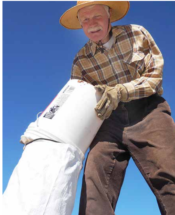
Fig. 5.2: Fill material is being dumped from a bucket into the mouth of the bag being held open by the chute.
