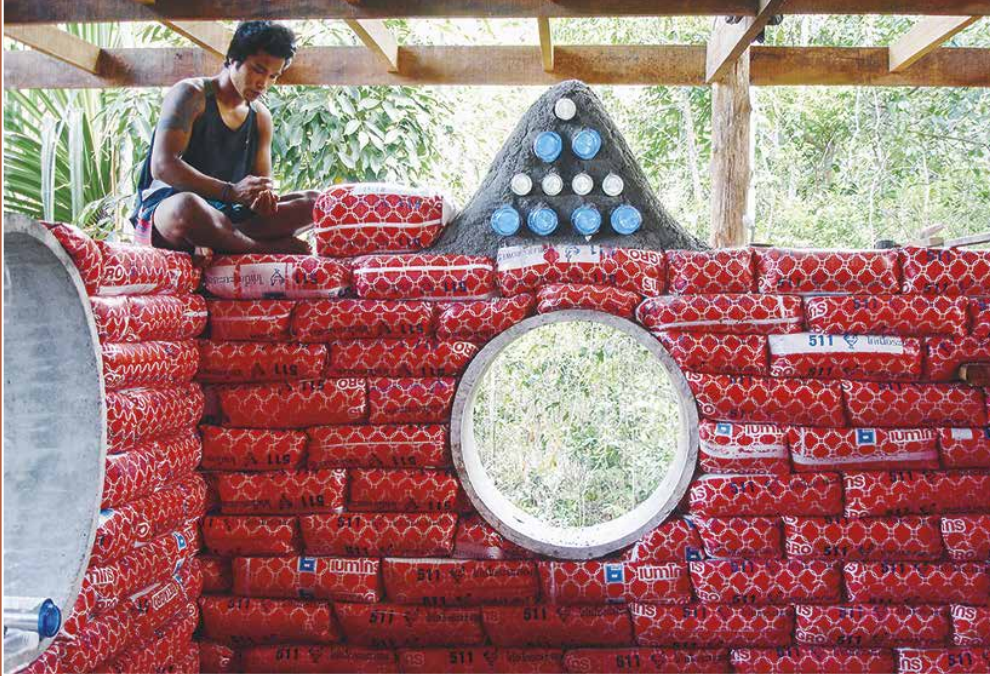
A tool shed and adjacent guest room is under construction at Phangan Earthworks in Thailand.
