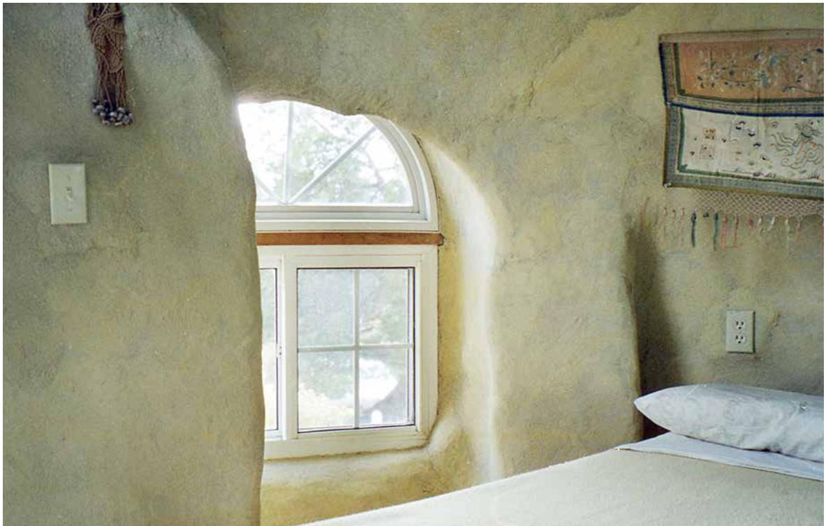
Fig. 11.1: Both a light switch and an electrical outlet are visible in this earthbag bedroom; the wire itself was embedded within the earthbag structure before the plaster was applied.
