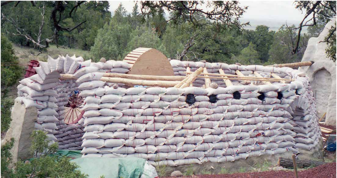
Fig. 7.5: The running bond pattern of this earthbag wall is obvious from the diagonal lines made by the end of each bag. You can also see how the bottoms of the bags are exposed where the wall ends. Also note the arch support: This is the shape that will provide a pointed, Gothic arch. CREDIT: KELLY HART
