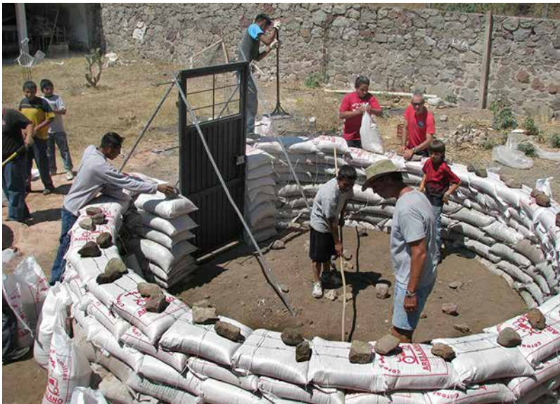
Fig. 4.7: Two strands of barbed wire have been placed along the top layer of this wall; stones temporarily hold the wires in place in readiness for the next course of bags. CREDIT: KELLY HART
