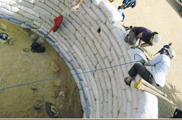
This photo was taken during the construction of the library in Mali. CREDIT: SCOTT HOWARD
