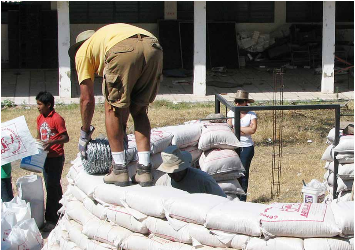
Fig. 7.4: This barbed wire was spooled in such a way that it was possible to unroll it directly on the wall.
