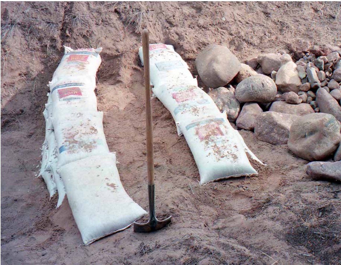
Fig. 16.2: This is what the earthbag dam looked like after the first three courses of bags.
