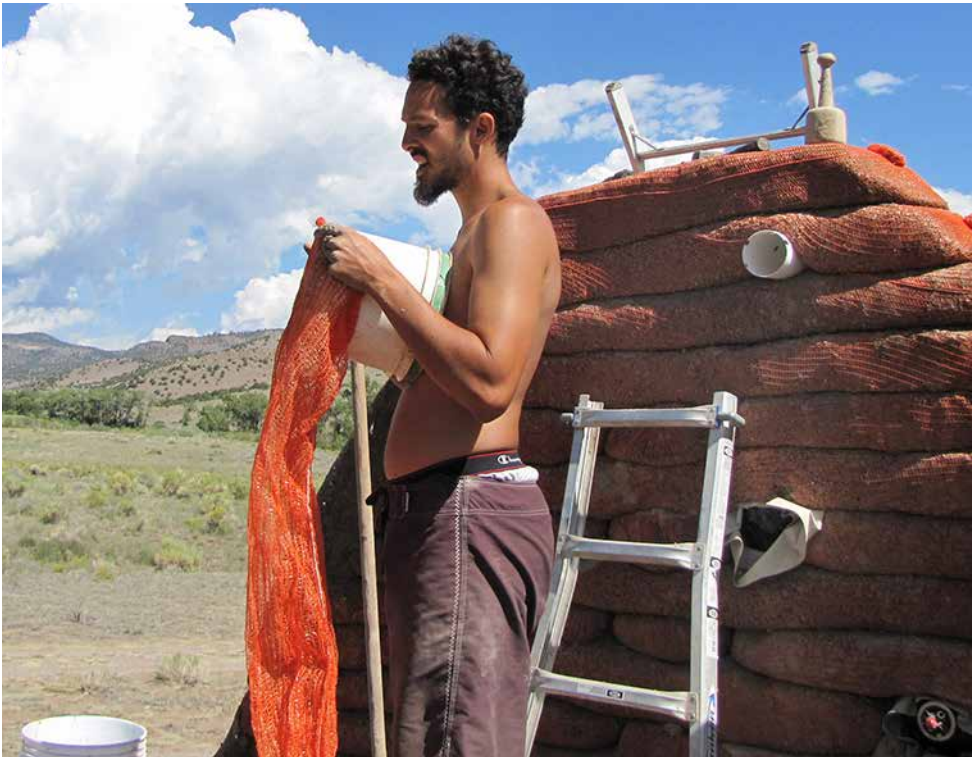
Fig. 7.3: A short section of mesh tubing is being fitted over a chute made by cutting the bottom out of a bucket. The tube is then filled on top of the wall right where it will be laid.
