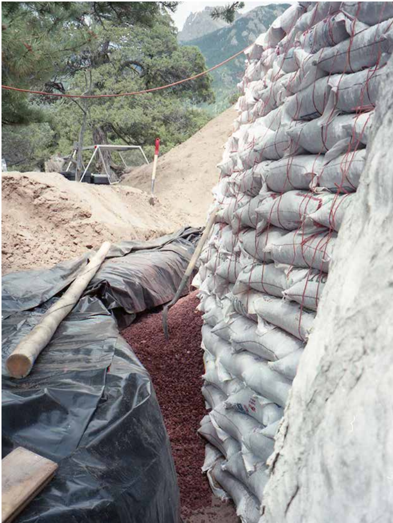
Fig. 6.3: This earthbag wall will be substantially bermed with soil, and scoria is being placed between the wall and the plastic moisture barrier to insulate the wall. The twine that is visible was an experiment in providing a kind of mesh for plaster, a practice that I abandoned when I started using actual mesh material for that purpose. CREDIT: KELLY HART
