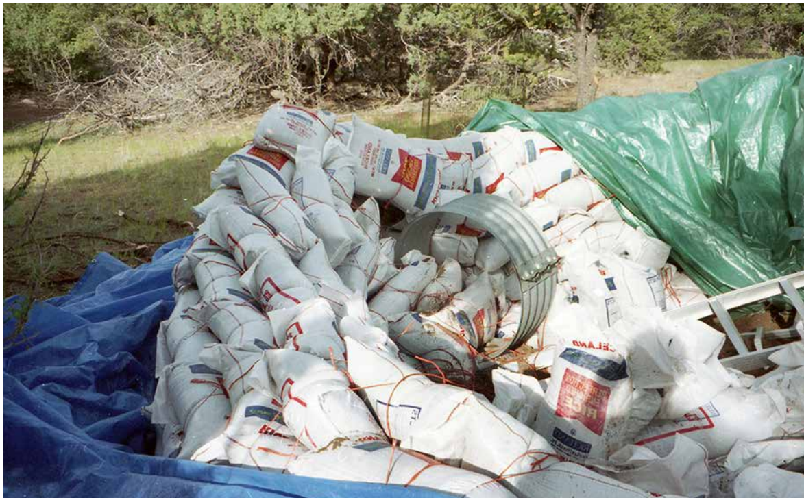
Fig. 4.5: The aftermath of a collapsed partial dome of earthbags filled with unstabilized fine sand.
