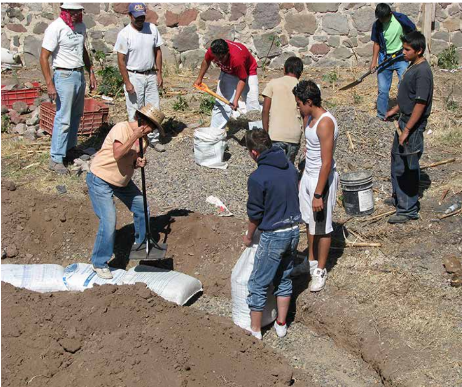
Fig. 6.1: The rubble trench foundation has been prepared with finer gravel on the top, and now bags of gravel are being filled, laid, and tamped into place, right at grade level.
