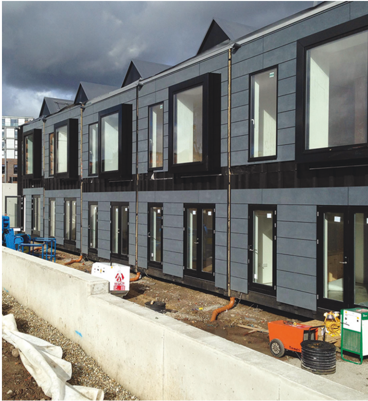
Plate 39: Units assembled in to terrace Multiple volumetric units are located to create the development. Two or three house units can be placed per day.
