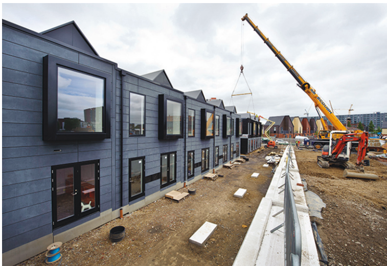
Plate 40: External zipping and completion Connection of external rainwater goods and final trimming take place once the volumetric units are assembled.
