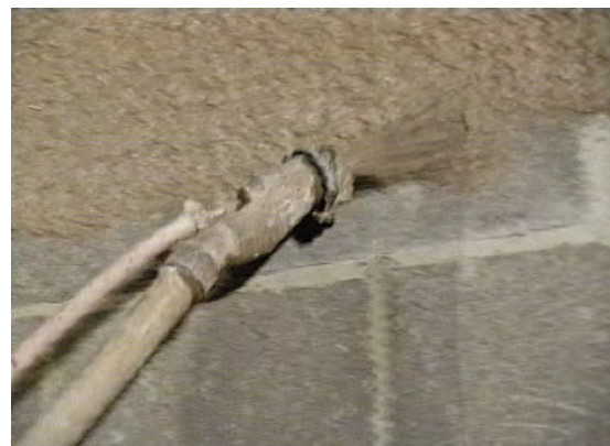
Gypsum plasters are mainly applied by hand. Machine projection is possible, and favoured, for large runs of work.
