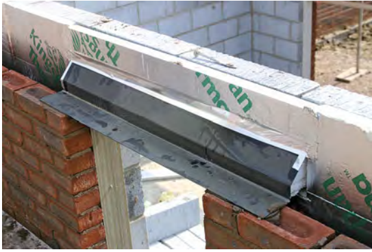
An insulated lintel over a window opening of a modern house. Note the plastic vertical insulated cavity closer in place (below the lintel); see the section on jambs below.
