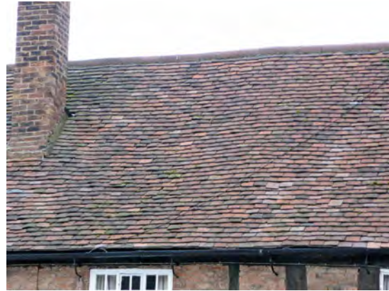
This clay plain tiled roof is of some age. Generally, the tiles are still performing adequately but a number have slipped.
