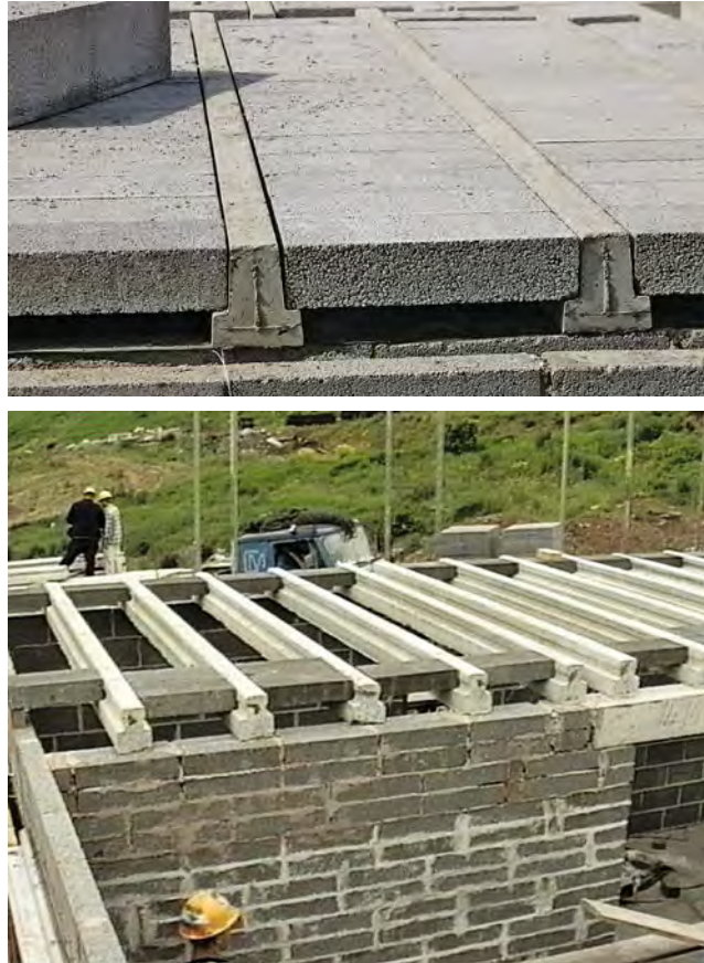
In a beam and block floor the beams should usually have at least 100mm bearing on the internal leaf of cavities and special narrow 'slips' are available to fill the space below the infill blocks.
