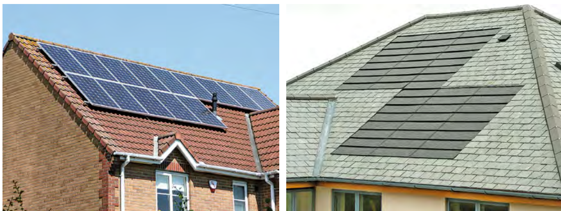
The house on the left, built in the mid-1990s, had a PV system installed in 2011. The panels are fixed to stainless steel rails that run across the roof above the existing roof tiles and are secured to the timber structure beneath. Note the individual cells within each panel. The right-hand bungalow has recently had integrated PV tiles installed at the same time as a new slate roof.
