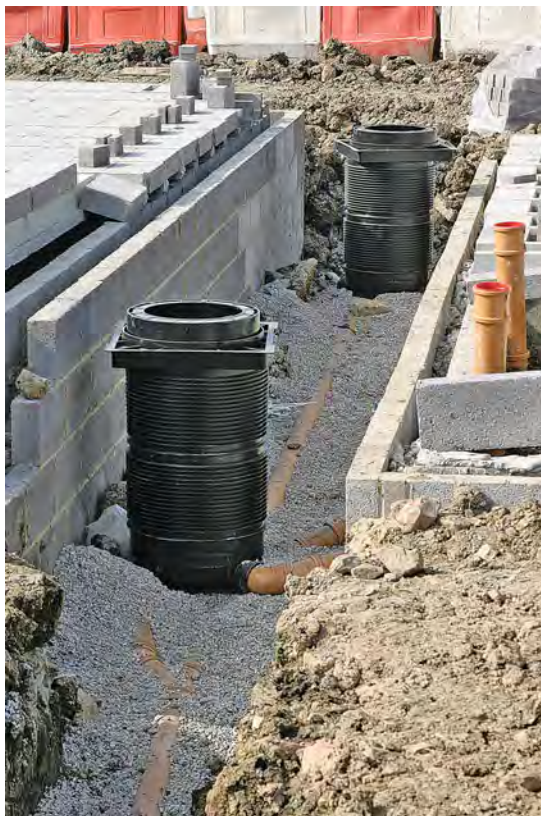
Plastic inspection chambers in position. (right-hand photograph courtesy of Hepworth Clay, Wavin Ltd.)
