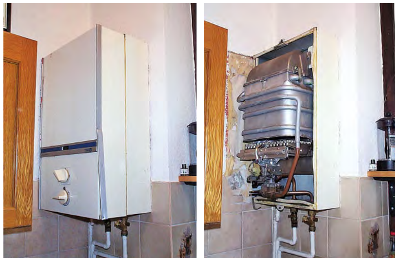
Gas multi-point water heater (right-hand image with cover removed).
