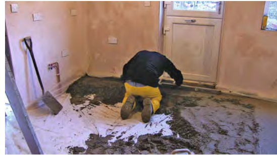
Laying a floor screed is a skilled operation. The cement/sharp sand mix should be laid fairly dry if subsequent shrinkage is to be avoided. It is levelled with a straight edge and then trowelled. It should be smooth enough to take carpets or vinyl tiles.
