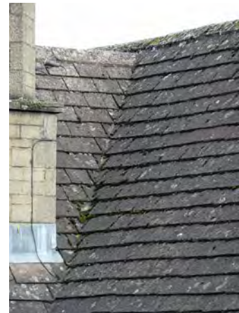
Valley tiles can be seen in this photograph of a concrete slate roof.
