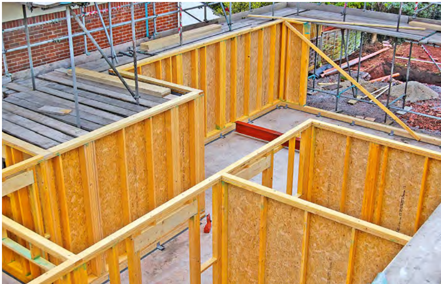
In this platform-framed house, the ground floor panels have been erected and are waiting for the first floor to be installed.
