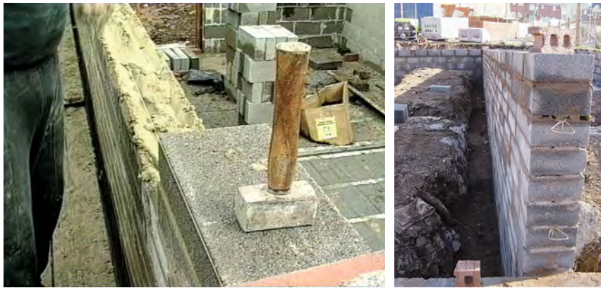
Dense concrete blocks laid flat can also provide a good party wall. They can be bonded in to the internal leaf of the cavity wall or connected by ties. As in the above example, a flexible cavity stop is required in the external cavity.
