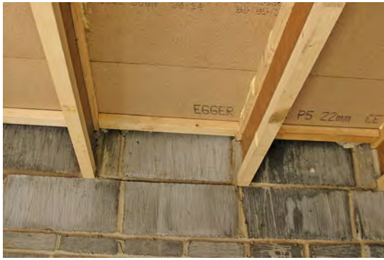
I-joist built into wall and using sealant to prevent air leakage (I-joist above and metal web joist right).
