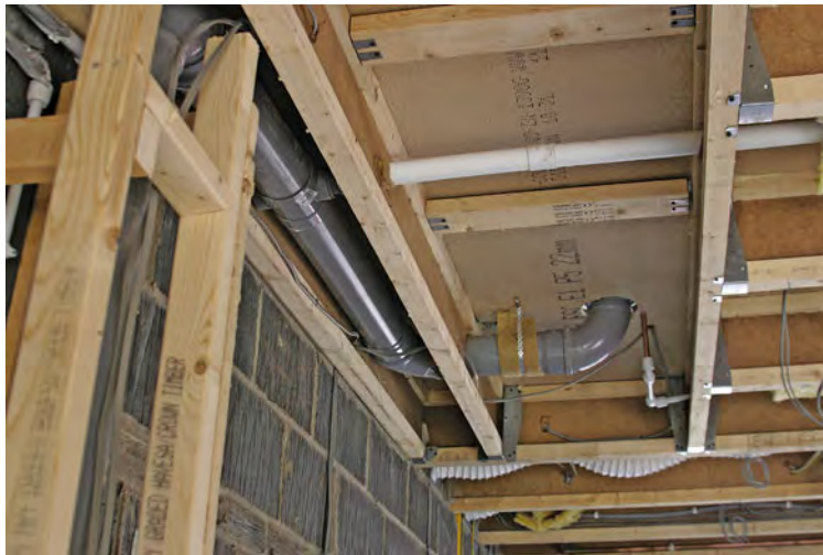
Services running through I-joists.
