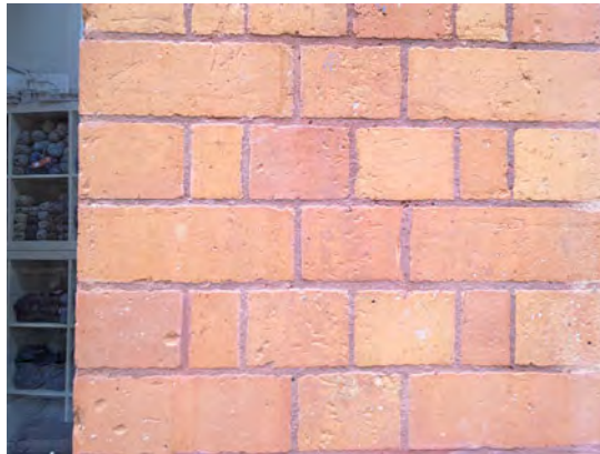
Flemish bond with Queen Closers at a return in a brick wall.
