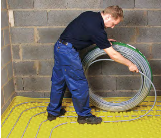
Plastic pipes are laid onto retaining sheet which in turn is laid on top of significant insulation. The pipes will be embedded in a screed, which will be laid once the whole system has been pressure tested.
