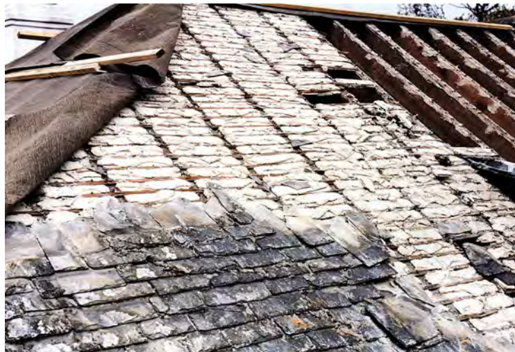
Torching retained moisture, thus encouraging rot attack in the battens. In addition, it was easily dislodged in the event of even slight structural movement of the roof timbers.
