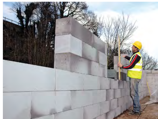
Solid block external wall under construction. Photograph courtesy of H+H UK Ltd.
