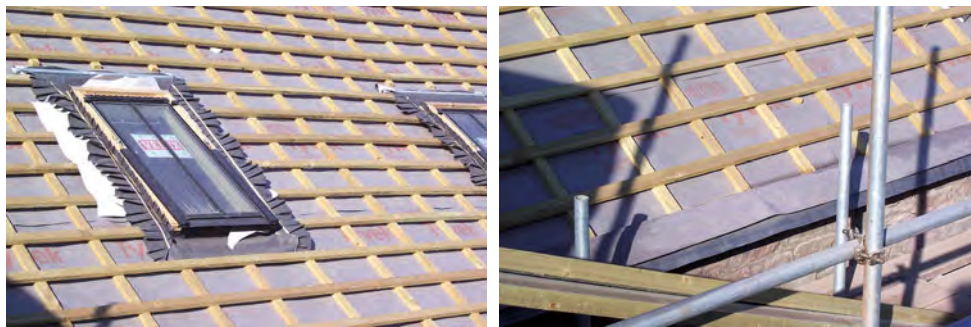
The photographs show a microporous underlay secured with counter-battens laid over each rafter. The counter-battens support the battens and permit airflow beneath the slates or tiles as well as drainage of any moisture beneath the roof cover.
