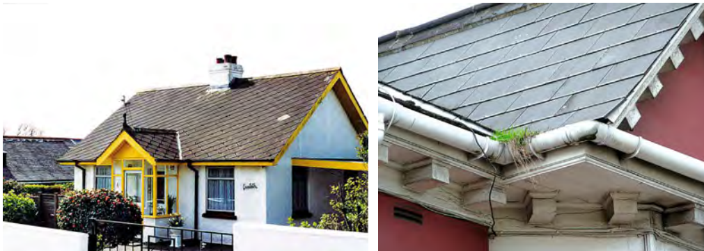
The bungalow in the left-hand photograph was constructed in the 1930s and the roof was covered with diamond pattern asbestos slates. The right-hand photograph shows a roof of modern synthetic slates fixed with nails and rivets. The slates are performing properly, the gutter is not. Note the slate-and-a-half slates above the verge.
