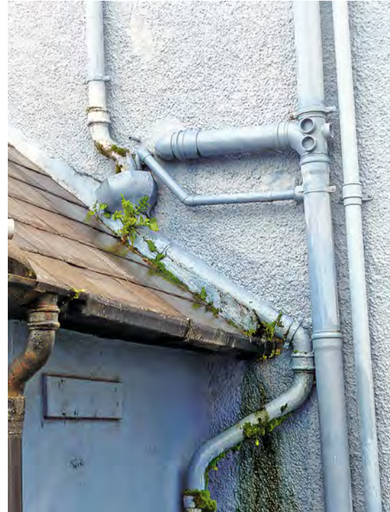
Blockages in this hopper have caused it to overflow.
