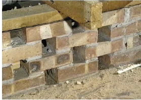
In a honeycombed sleeper wall there are a series of gaps to allow cross-ventilation.
