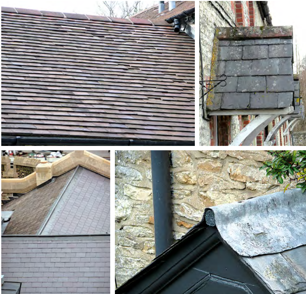
Top left photograph shows a plain tiled roof with clay ridge tiles. The slate covered porch on the top right is finished with clay ridge tiles. Each slate roof on the bottom left has been finished with a lead ridge, which has been dressed over a roll, while the bottom right photograph shows a detail of a lead roll – note: it should have a capped end.
