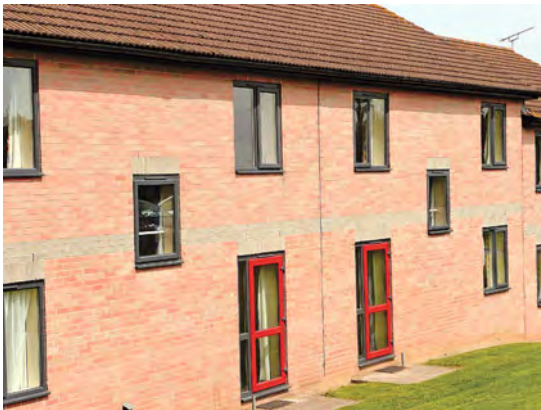
Movement joint (vertical line between two red doors) on a terrace of modern houses.
