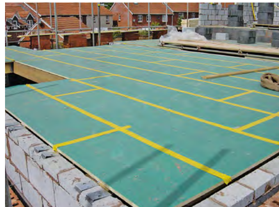
This photograph shows chipboard flooring wrapped in plastic. The chipboard should be a moisture-resistant grade. The plastic covering is temporary and is intended to protect against rain penetration and material spills, etc. during construction.
