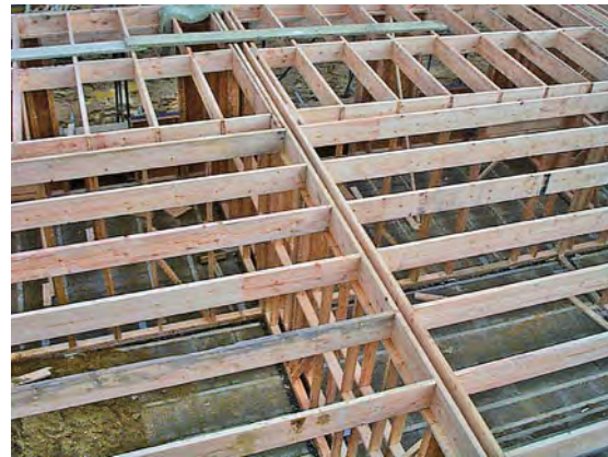
Looking down from above, it should be clear that the floor structure does not cross the party wall. Header joists on either side of the cavity provide support for the upper storey panels and will delay fire or smoke in the cavity of the party wall entering the floor void.
