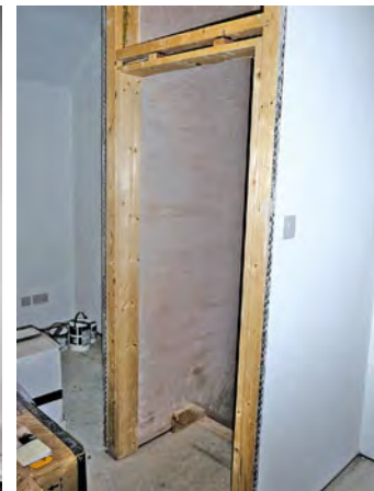
A lining fixed into new studwork partition. The edge of the studs and the gap between these and the lining will be finished in a wide softwood architrave.
