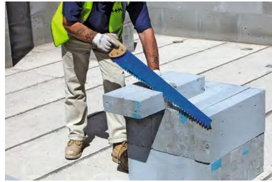
Aerated blocks being cut on site (note that the blocks shown are those used in 'thin joint systems' and are therefore larger than standard aerated blocks). Photograph courtesy of H+H UK Ltd.
