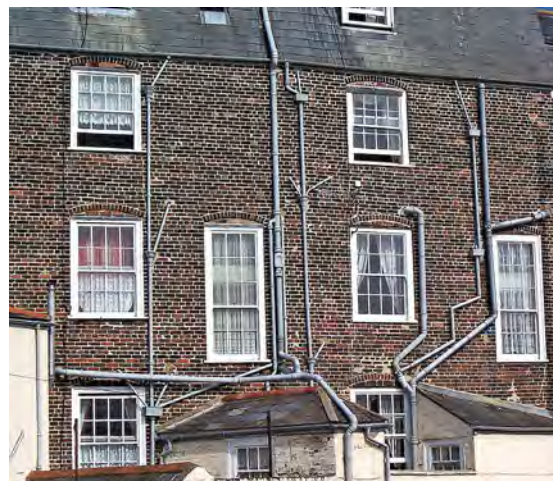
This photograph shows examples of the two-pipe system serving a larger property that has been converted into flats. Over a period of years the system has been adapted and extended, resulting in an unsightly tangle of poorly designed and poorly supported pipes, with associated maintenance problems.
