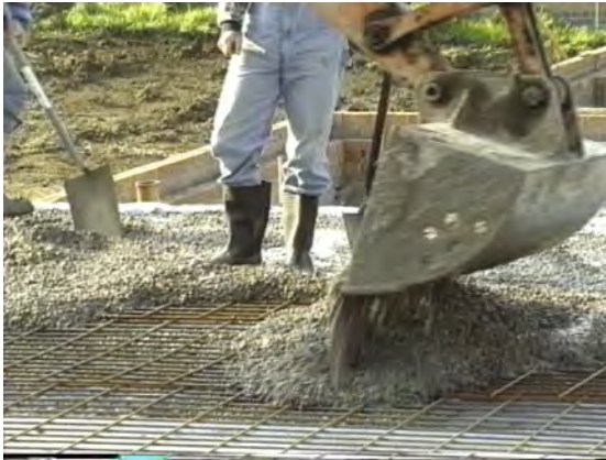
If the ground below the slab contains any localised soil weaknesses, the concrete can be reinforced with a layer of steel mesh.
