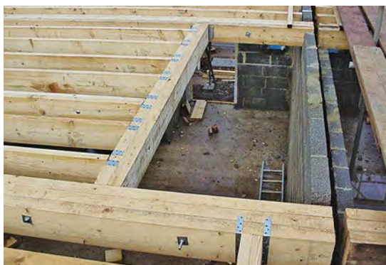
A staircase opening showing trimming, trimmed and trimmer joists (refer to the diagram above).
