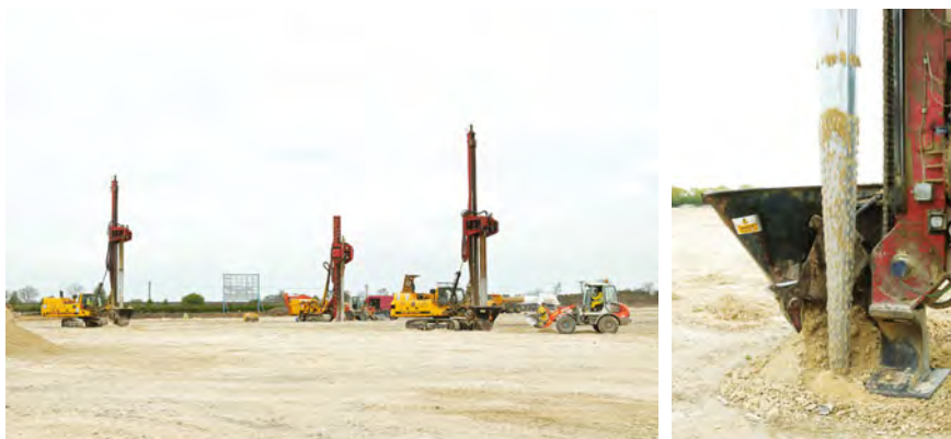
These two photographs show a site receiving vibro-compaction prior to development. Photographs courtesy of Roger Bullivant.
