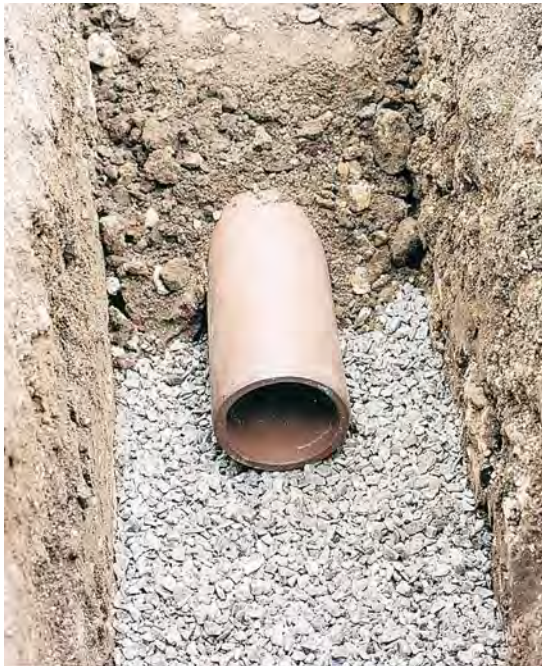
This image shows a drainage pipe laid on a bed of limestone chippings and the backfill. Courtesy of Hepworth Clay, Wavin Ltd.
