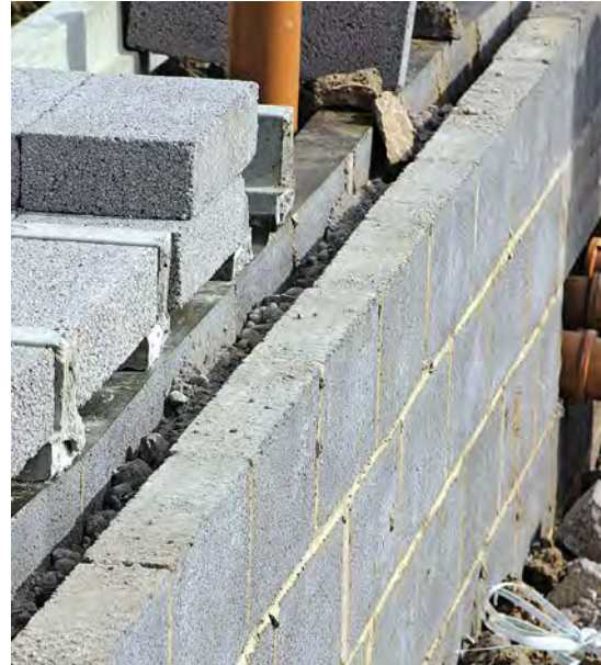
The cavity fill below ground level helps to ensure that the two leaves are not squeezed together by pressure from the ground when the trenches are backfilled.
