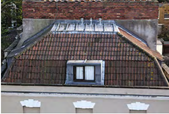
A lead covering to the flat portion of a Georgian mansard roof.
