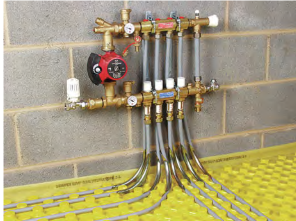
Plastic pipe manifold. This separates and controls the hot flow and cooler return water throughout the installation, connecting back to the heat source's flow and return.
