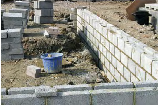
External wall up to the level at which it will receive a suspended concrete ground floor.
