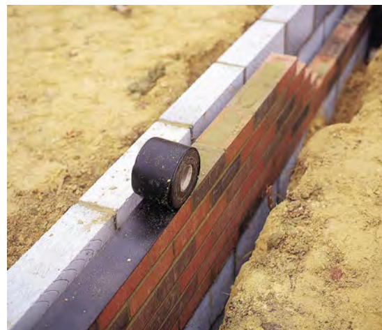
DPC being laid to cavity wall (shown here on brick outer skin but will also be applied to inner skin of blockwork). Photograph courtesy of H+H Ltd.
