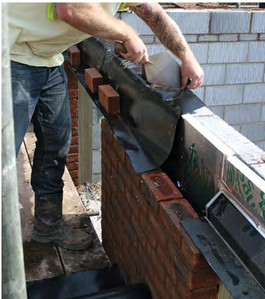
A cavity tray in the process of being formed over a lintel.
