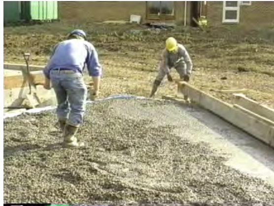
When the slab has been cast it is tamped with a straight edge to level it and remove surplus air and water. Mechanical powered tamps are also available.
