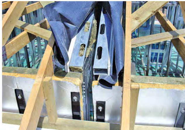
This photograph shows party wall construction (unfinished). You can clearly see the two independent panels. Fire stopping will be required to fill the cavity at the outer edge of the two panels and cavity barriers will be required in the external wall cavity. Typical details are very similar to timber framing.
