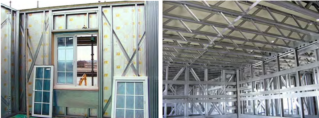
The left-hand photograph shows a braced and framed panel ready for its internal skin to be installed. On the right, the photograph shows part of a terrace of houses. The wall on the right is an internal loadbearing wall. The wall on the left is a separating (party) wall – hence the double panel construction. The diagonal braces help to stiffen the frame and prevent racking. The narrow steel strips fixed to the panels provide fixings for kitchen units, etc.
