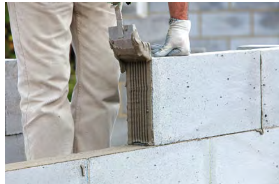
The thin joint is formed using special tools (in this example a 'scoop') to apply the mortar. Photograph courtesy of H+H UK Ltd.
