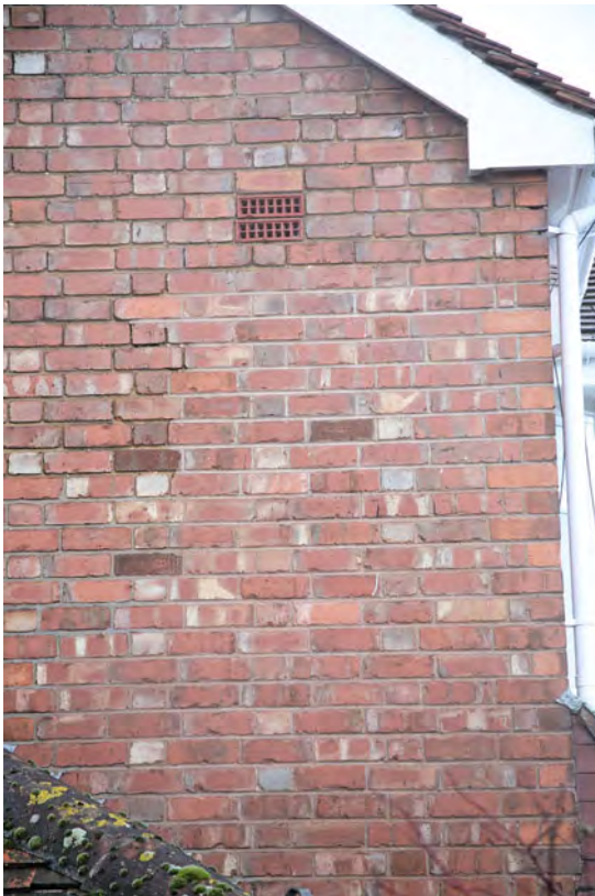
Flemish garden wall bond to a gable wall on an early 1920s house.
