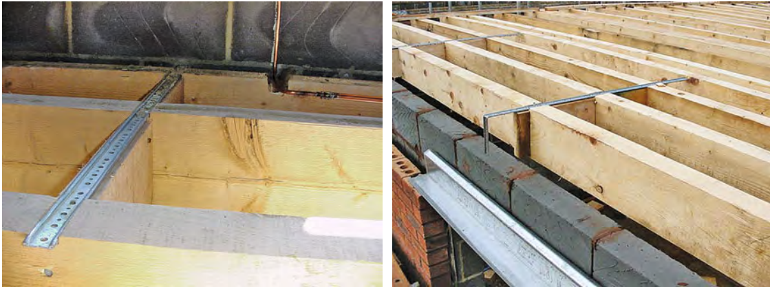
Tying in the external wall to the upper floor where joists run parallel. A galvanised strap extends over three joists with timber blocking below. The joists are notched slightly to ensure that the top of the straps are flush with the top of the joists.
