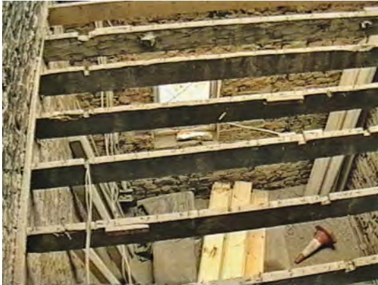
Many early floors are still functioning as originally intended. If problems of rot or insect attack can be avoided, a floor should last almost indefinitely. Some early floors are undersized by modern standards. This problem can be exacerbated by excessive notching, etc. to provide service runs.
