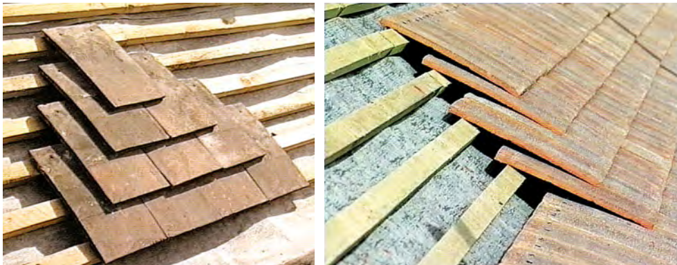
Examples of plain tiling that show the double lap and the head-lap, i.e. the amount by which each tile laps the next but one below, which should be at least 65mm.
