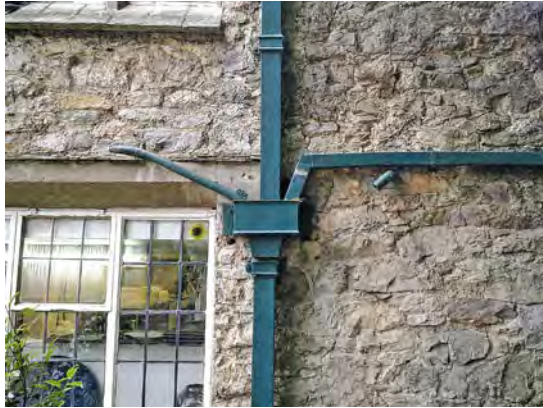
Hopper heads were common on two-pipe systems.
