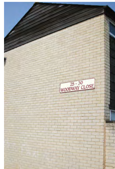
Calcium silicate bricks in a 1960s house.
