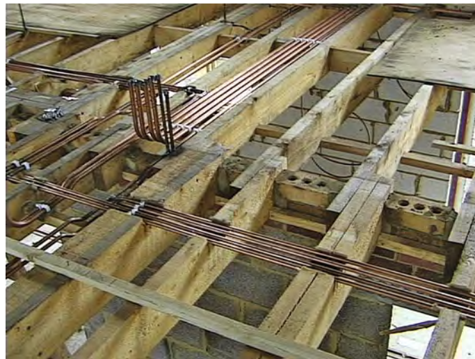
Copper service pipes running through notches in a solid timber upper floor.
