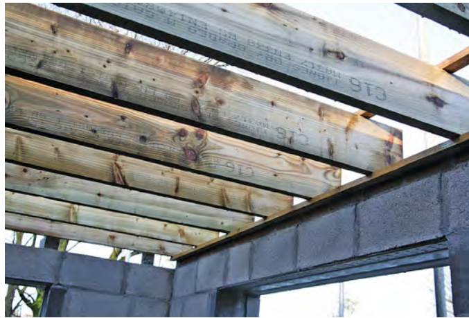
A modern house (2012) using solid ('cut') timber joists to form the first floor.
