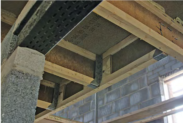
Stair opening formed with an I-joist floor. Note the blocking pieces behind the joist hanger to allow proper fixing of the hanger.
