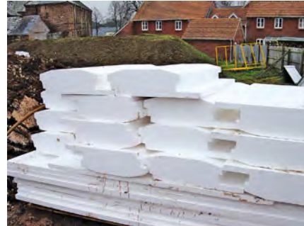
In modern construction, ground bearing floors are becoming quite rare. Pre-cast floors now account for approximately 65 per cent of all new ground floors. The system shown here uses polystyrene blocks which fit in between the beams (and extend below it to prevent cold bridging). An in-situ concrete topping completes the floor. This can be screeded or power floated.
