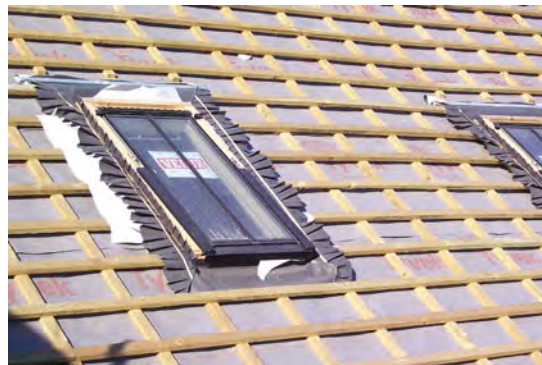
A composite roof window – known by its trade name 'Velux' – being installed in a new pitched roof.
