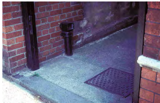
Vent to an interceptor trap in adjacent manhole.
