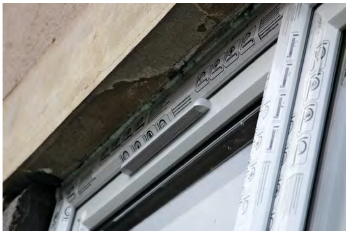
Although there are other means, background ventilation is often provided by the incorporation of controllable 'trickle ventilators' within the structure of a window. The photograph shows a trickle ventilator in a newly installed window (hence the protective wrapping).
