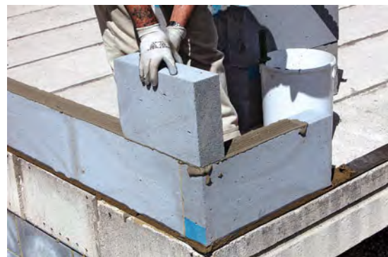
The two images above show the first course of a thin joint block being laid on a mortar of traditional thickness in order to ensure a level base for subsequent courses. Photographs courtesy of H+H UK Ltd.
