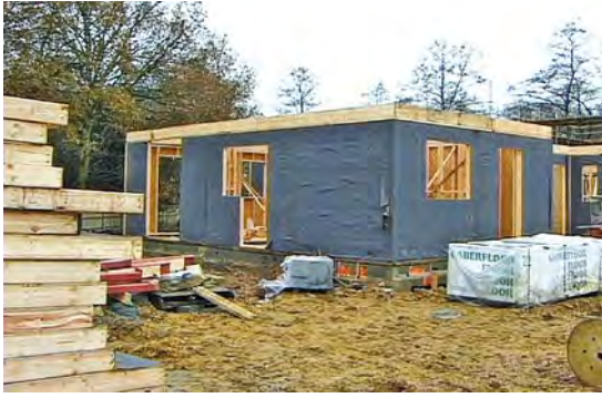
When all the ground floor panels are in place, the next stage is to build the 'platform' ready for the top storey panels. The panels are factory-fitted with a waterproof, but vapour-permeable, membrane.
