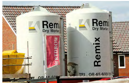
Dry mix mortar silos on site.
