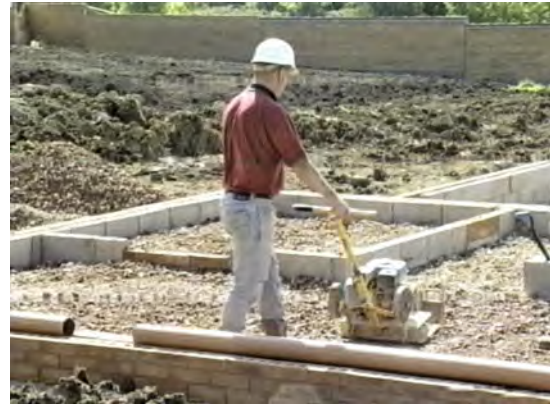
The hardcore is compacted by a vibrating plate or roller. The top of the hardcore is kept below the substructure blockwork so that the slab can be cast inside the walls.
