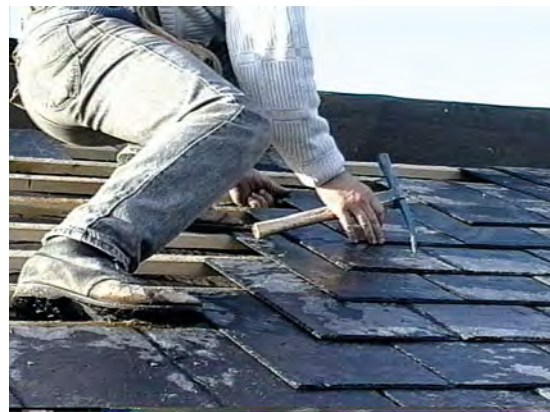
A slate roof being laid – note how the slate is being centre nailed. Slate is normally fixed by nailing. The nail holes can be pre-drilled at the quarry or formed on site using a special hammer called a zax.
