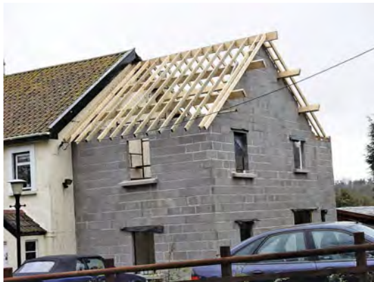
This is a modern purlin roof. This roof is slightly unusual in that there are two purlins on each slope (one on each slope is more common). The purlins support the rafters which, in turn, support the roof battens and tiles. The purlins are built into the gable wall and the party wall for support.
