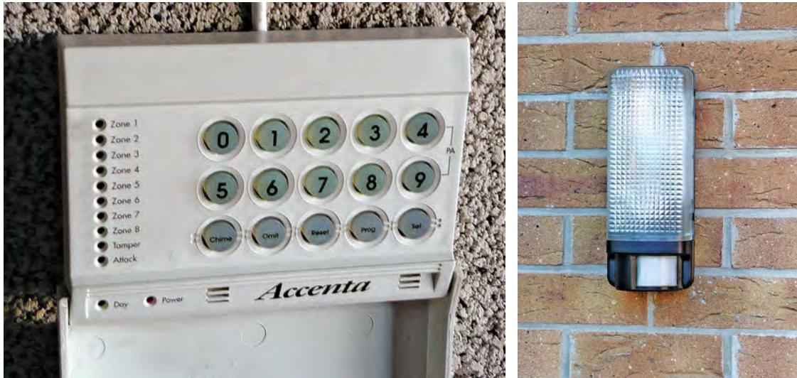
The programmable control unit, showing a number of zones on the left, is linked to the external alarm box shown previously. The external security light has an in-built PIR detector at the bottom.
