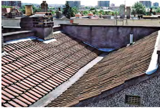
A butterfly roof above a Victorian terraced house showing how each slope drains into a valley gutter. The original lead valley gutter has failed and has been temporarily lined with felt. You can just make out the steps to the original gutter. Note: the clay double Roman tiles have been 'stretched' (i.e. have an extended gauge) to save cost – this is not good practice.
