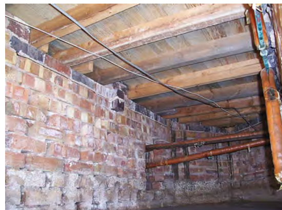
The floor was built in about 1960. The sleeper wall is roughly honeycombed and, although there is no wall-plate beneath the joists, there is a course of dense engineering bricks acting as a DPC.
