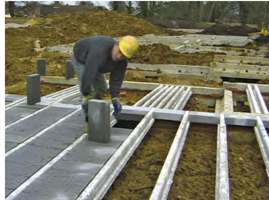
The pre-stressed floor beams sit inside the ground beams (see Chapter 3). Concrete blocks, in this case aerated blocks, are then placed between the floor beams. When all the blocks are in position, any small gaps are filled with grout.
