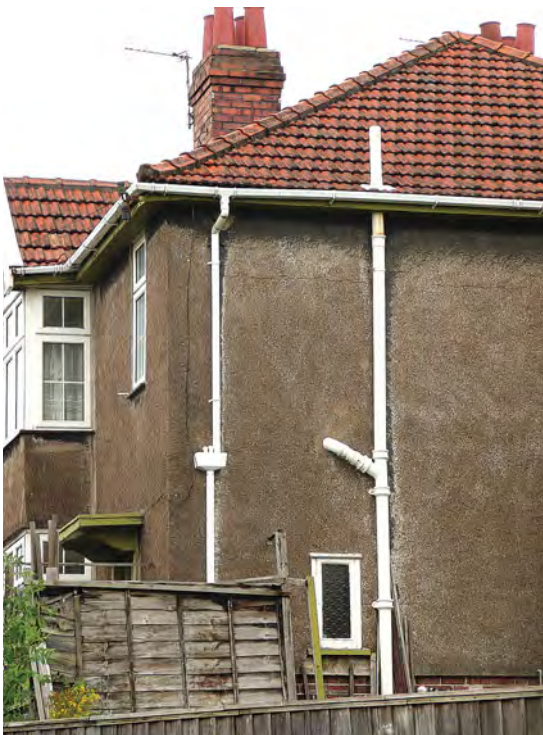
The photograph shows a house dating from the 1930s served by a two-pipe system. One of the pipes carries the soil from the toilet and the other carries the waste from the bath and basin. On many properties the waste pipe also carried rainwater from the roof (as shown here).
