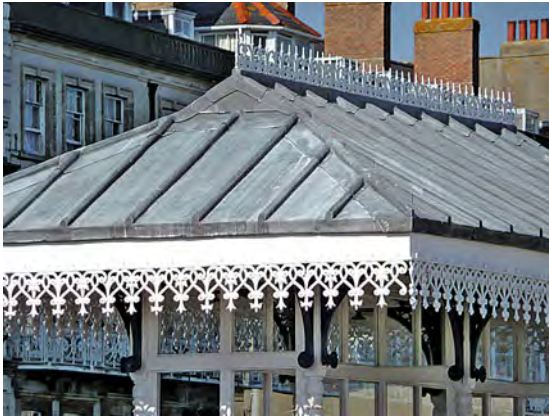
This sea-front shelter in Weymouth has recently been re-roofed in leadwork. Note the individual lead sheets dressed over the rolls and the hip detail.
