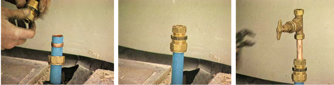
The photographs above show the compression fitting where the incoming main (polythene) is joined to a copper rising main. The stop tap allows the supply to be isolated for maintenance purposes. A drain cock will be fitted just above the stop tap to enable the rising main to be drained.
