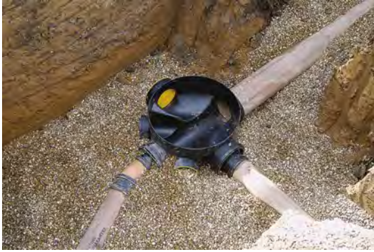
The base of an inspection chamber with pipes connected and trench partially backfilled. Courtesy of Hepworth Clay, Wavin Ltd.
