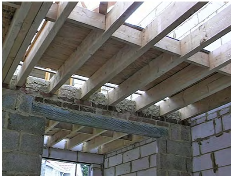
An opening in a modern internal loadbearing wall. The wall is made from dense blocks (unlike the internal leaf of the cavity wall on the right which is lightweight block). Upper floor joists are built into the top of the wall and are supported over the opening by a steel lintel. Note: the right-hand side of the lintel should be supported by a full block not a cut one.
