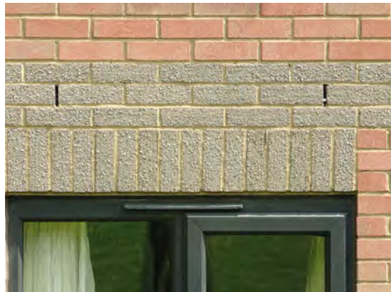
Sometimes (as here) the cavity tray is located a few courses above the opening.
