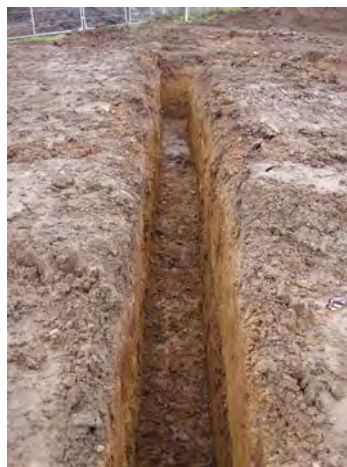
This trench in a shrinkable clay sub-soil has been excavated to a depth of at least 1,200mm to avoid the effects of seasonal change.
