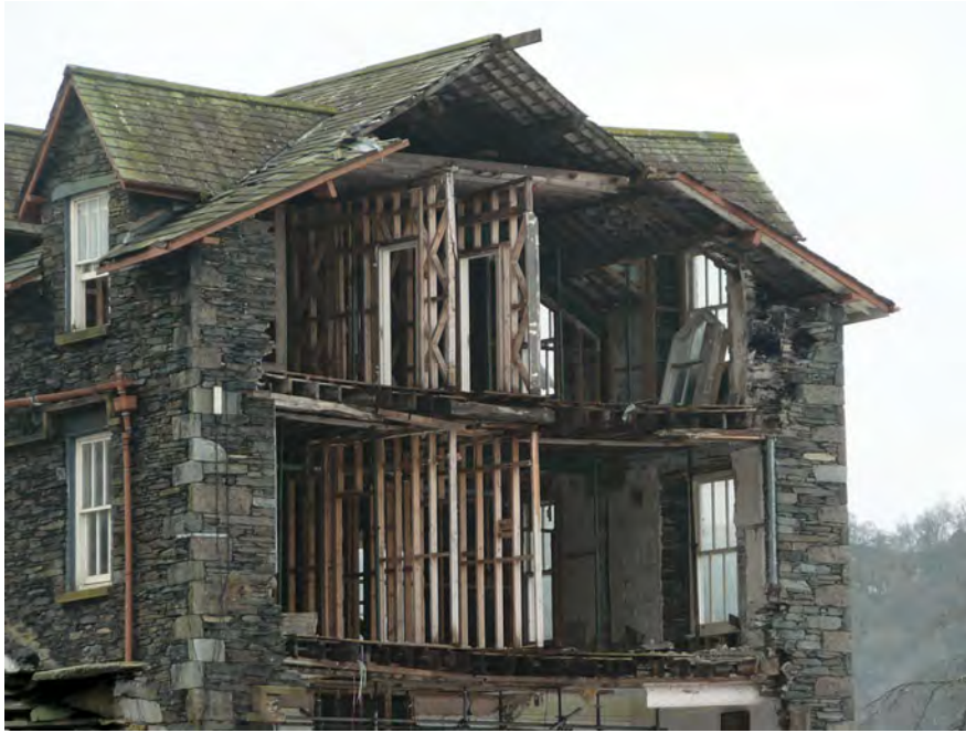
The timber stud partition on the upper floor has diagonal bracing (on the left-hand side) so it was meant to be loadbearing. The lower partition was non-loadbearing. However, because there is no supporting partition on the lowest floor, both upper floors are sagging as the design did not properly take account of the load from the partitions themselves plus the roof.
