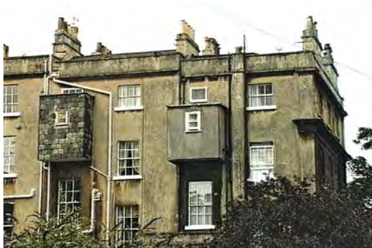
The cantilevered back-additions shown on the left are early water closets. They are Victorian additions to Georgian houses in Bath and are typical examples of how such houses were 'modernised'.
