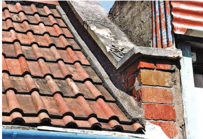
A clay double Roman tiled roof on an older building with a mortar flashing to an abutment with a parapet wall.
