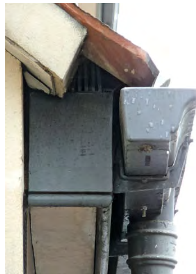
The grey fascia board and the white soffit board can be clearly seen in the photograph. Note how far the tile overhangs the fascia to discharge into the gutter.
