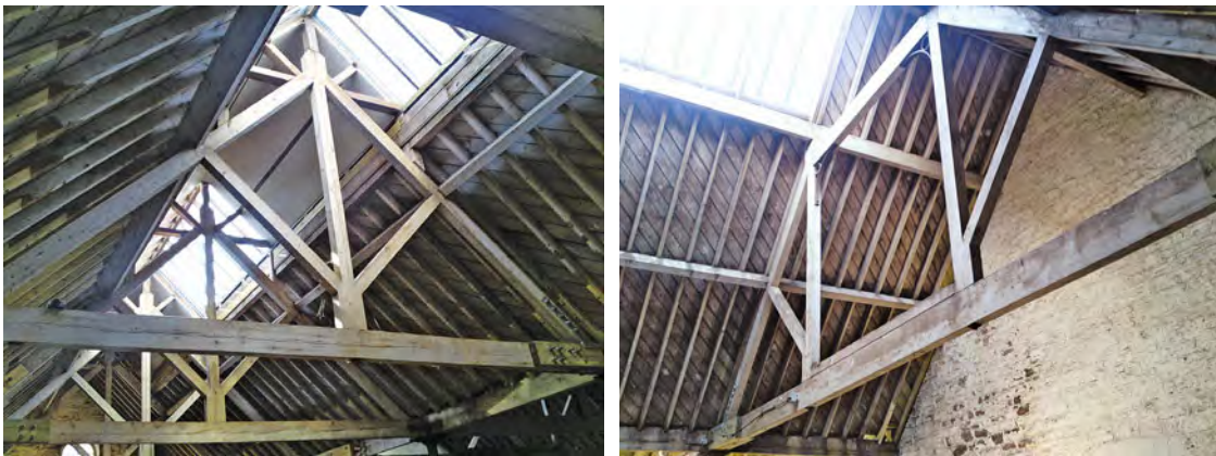
The left-hand image shows a king post truss. They provide support for the purlins without the need for internal loadbearing walls. This enables the floor space below to remain open plan. The photograph on the right shows a queen post truss. In some forms of construction these are so big that accommodation, i.e. attic space, can be formed within them.
