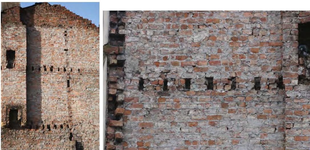
The photographs above are of the party wall remaining after the demolition of a Victorian house. The 'sockets' where the first and second floor joists were built into the party wall are clearly visible. The close-up view shows the empty sockets, but also note the stretcher and header bricks of the front external wall, which are clearly visible to the left-hand side of the image.
