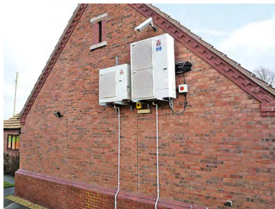
Air handling units located on a gable end.
