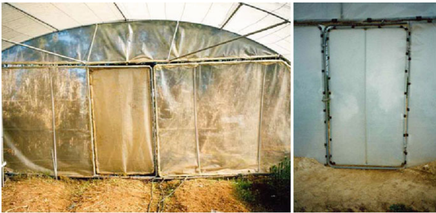
Fig. 8.28 Leaky doors where insects can penetrate and heat energy will be lost at night
