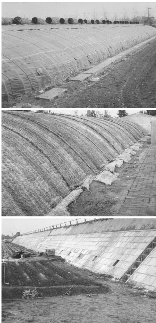
Fig. 5.56 Greenhouse in China. A round-arched structure is leaned against a north wall, and will be covered by straw mats at night
