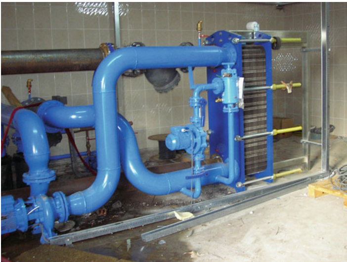
Fig. 12.17 Heat exchanger for geothermal water in Turkey
