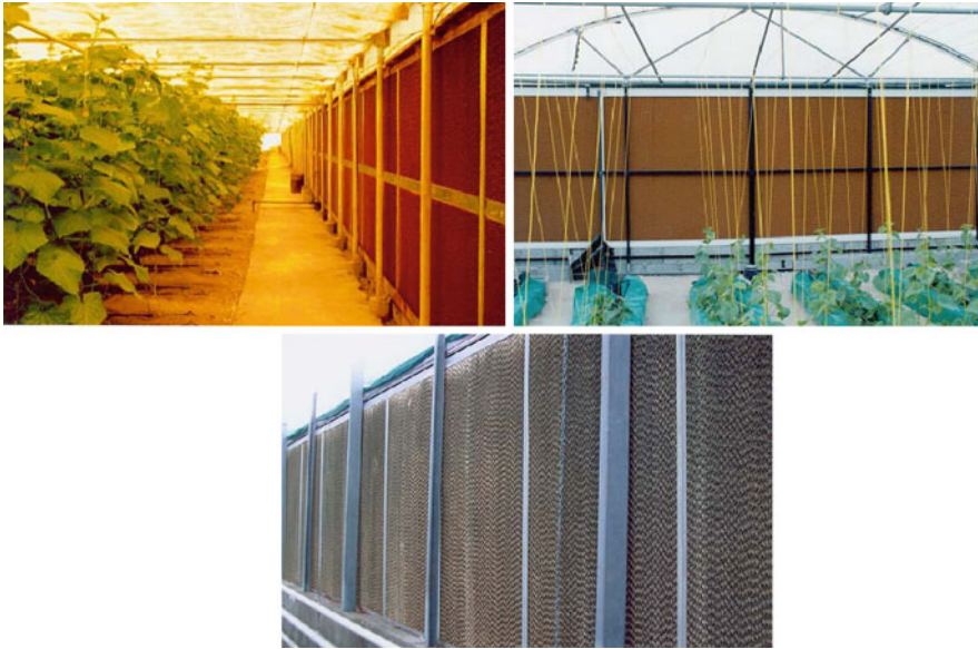
Fig. 11.6 Well-installed, operated, and maintained corrugated cellulose pads
