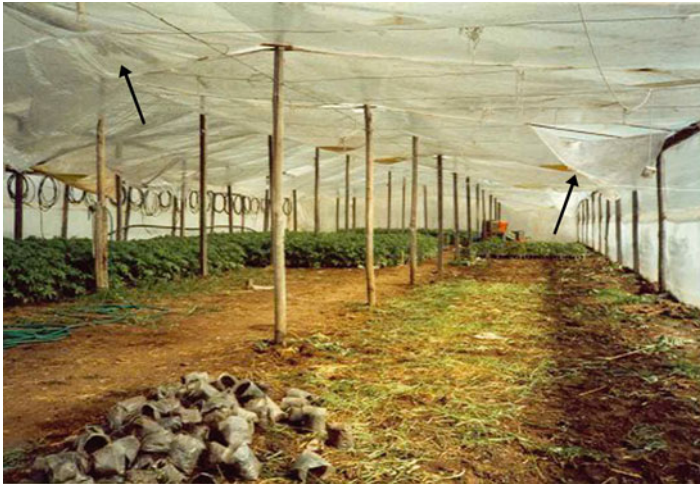
Fig. 5.71 Water pockets in the plastic film of flat roof
