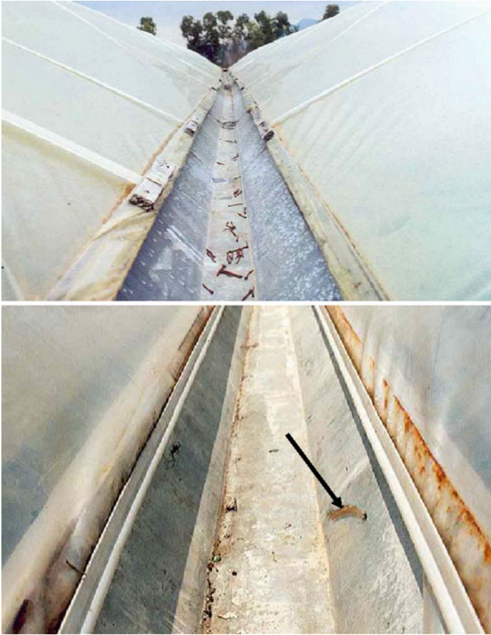
Fig. 8.29 Forgotten nails and screws cause rusting-through of the gutter. One corroded hole is closed by a wooden stopper
