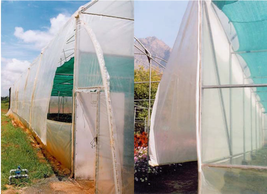
Fig. 9.7 The roll-up vents are moving and fluttering at the side wall due to wind forces, causing leakage and danger of destruction. The roll-up vents are not stretched close enough to the construction by ropes or steel rods
