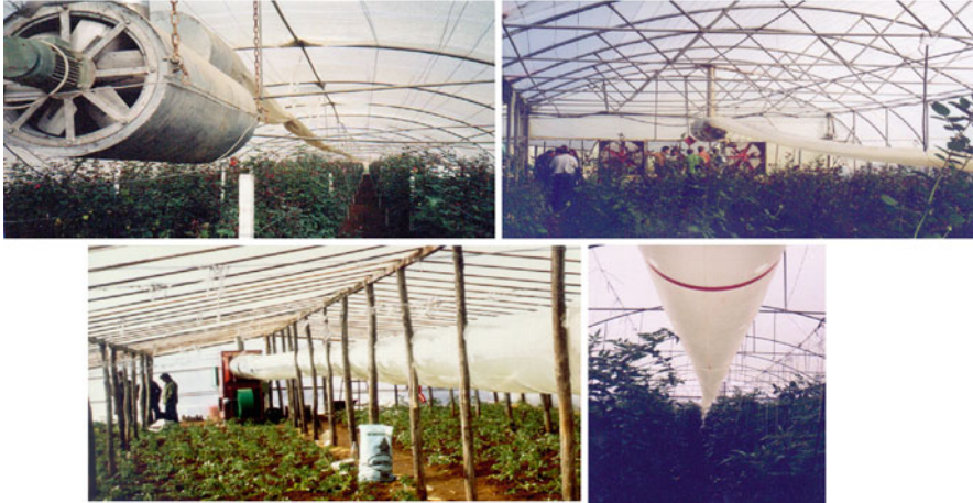
Fig. 12.7 The plastic tubes are installed too high above ground and plant level
