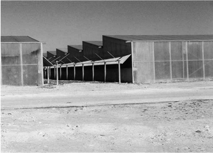
Fig. 5.63 Shed roof structure covered with corrugated polyester sheets. Those sheets are not recommendable anymore, because the light transmittance decreases within a short time and the sheets are relatively expensive.
