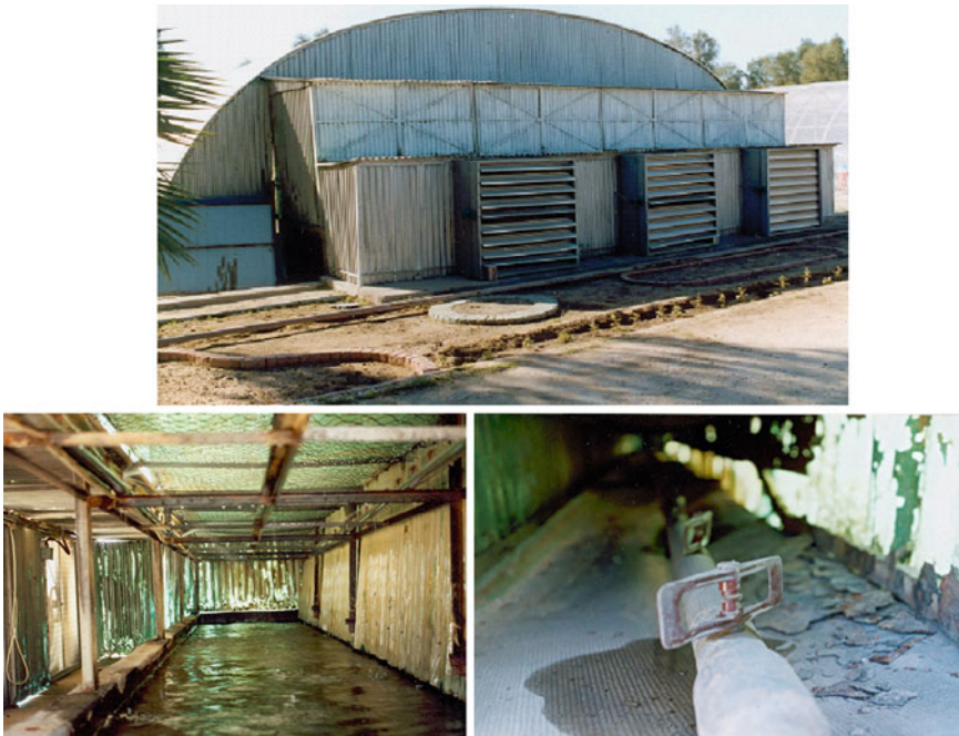
Fig. 11.36 Positive spray cooler in Kuwait 2002 (type A in Fig. 11.35), with inside view above water basin and nozzles
