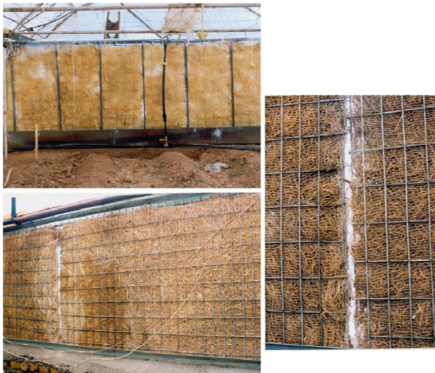
Fig. 11.15 Leaks in pad systems should be avoided. Shrinking of natural material has to be avoided by continuous refilling
