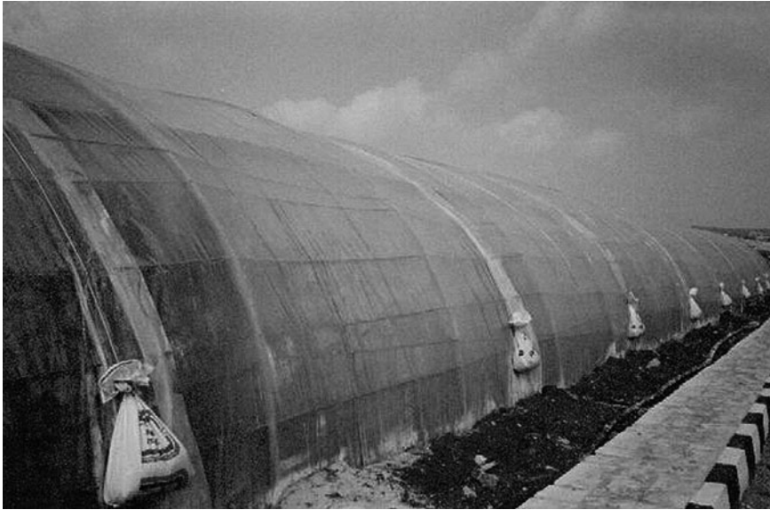
Fig. 5.8 Greenhouses without foundations are secured against uplift forces by sand sacks (Jordan). Point foundations are preferable
