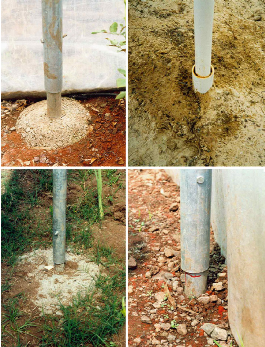
Fig. 8.2 Some well-designed concrete foundations. The vertical columns should be inserted on or in a pipe which is part of the concrete foundation block. The columns should be fixed by screws or bolts and not welded
