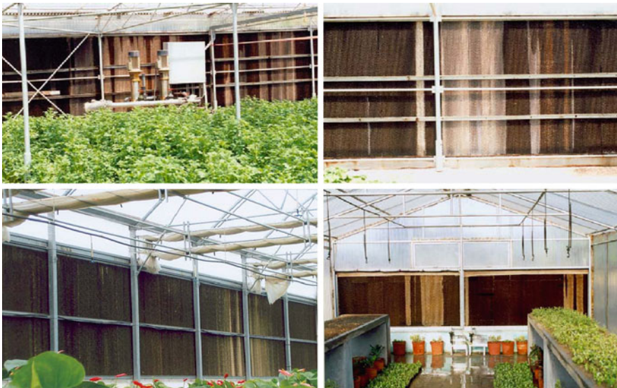
Fig. 11.22 Partly dried out pads reduce the cooling efficiency
