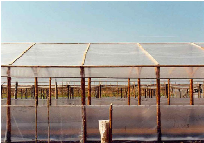
Fig. 8.14 Nailing the plastic film onto the structure is time-consuming and not recommendable
