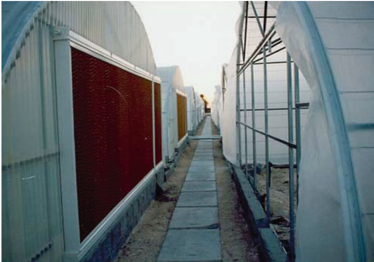
Fig. 11.20 The pad is installed nearby the pad outlet of the next greenhouse, so that the warm and humid air directly enters the next greenhouse and reduces the cooling efficiency remarkably
