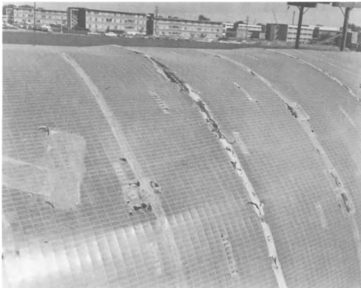
Fig.3-37. Degradation of a 6 mil vinyl film after 20 months service on a Colorado State University quonset structure
