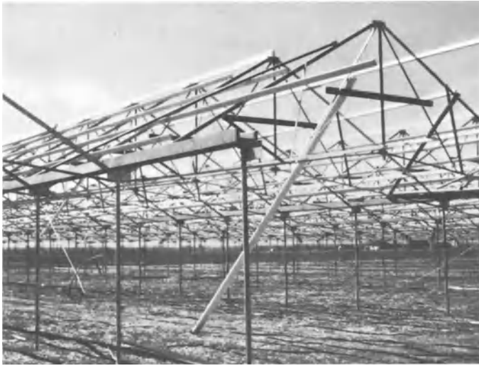
Fig.1-8. Example of galvanized steel superstructure to be covered with fiberglass. Wooden gutters are supported on galvanized pipe posts
