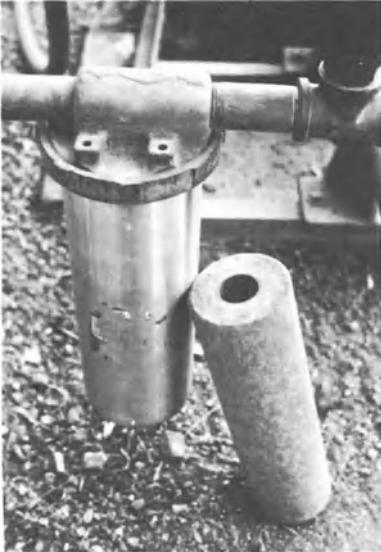
Fig. 5-14. Filtering system for high pressure mist system. Filter capable of removing particles down to 150\ \mu diameter. All mist systems should be protected, and require water with few salts
