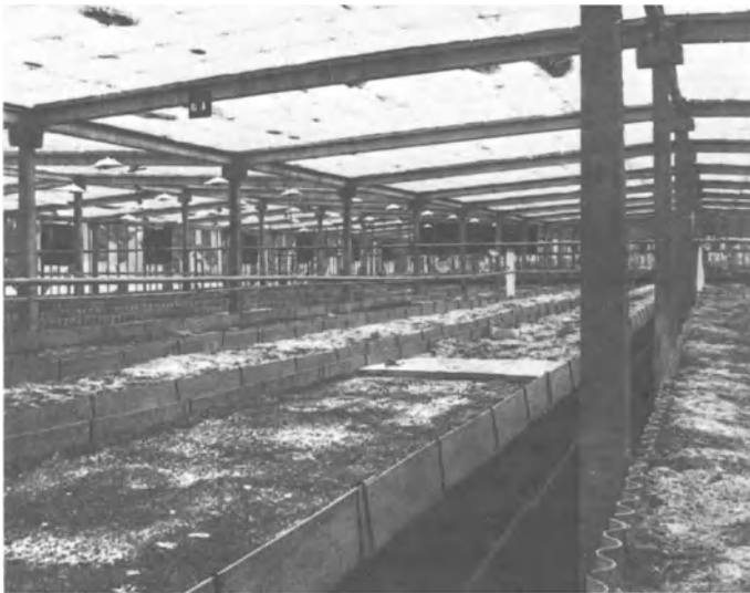
Fig.1-7. Example of concrete superstructure with thin layer polyethylene for roof, sandwiched between layers of wire mesh, in a geographical location where wood is scarce and steel costly. Flat roof indicates that snow loads are nonexistent, and rainfall slight
