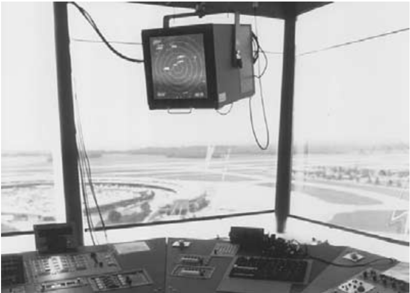
Fig. 20-3. The enhanced D-BRITE radar in the tower displays the same data as those on the Approach Control TRACON scopes.
