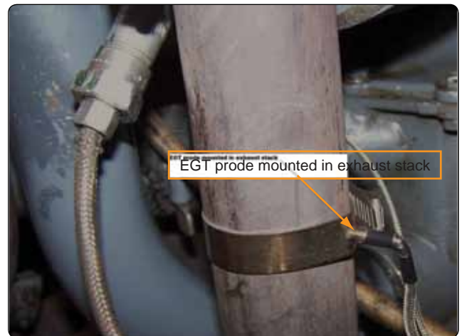
Figure 6-60. EGT probe in exhaust stack.
