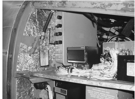
Figure 7.8 Fuses located in a panel
