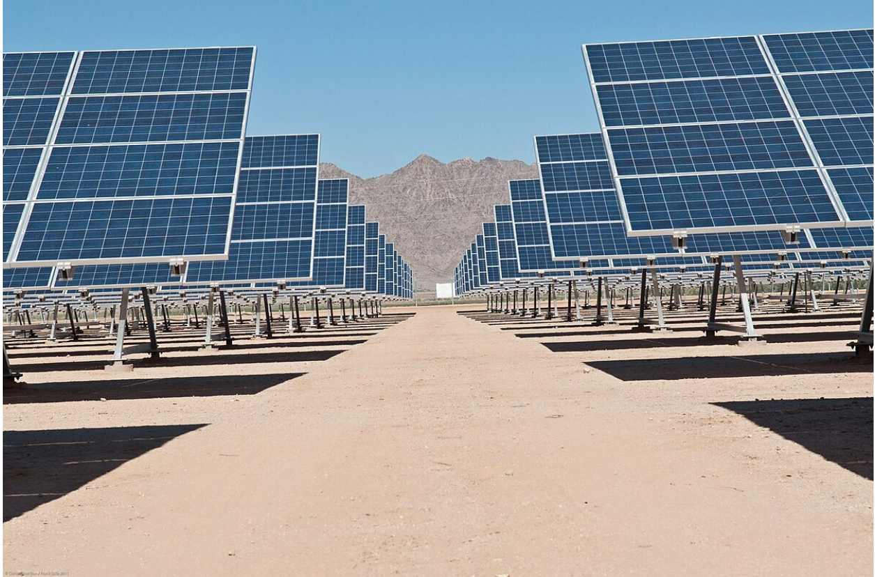
4. Solar Panels Plant System. Source: RPC Communication Unit, CC BY-SA 4.0 < https://creativecommons.org/licenses/by-sa/4.0/ >, via Wikimedia Commons: https://commons.wikimedia.org/wiki/File:Rpc_solar_plant_system.jpg
