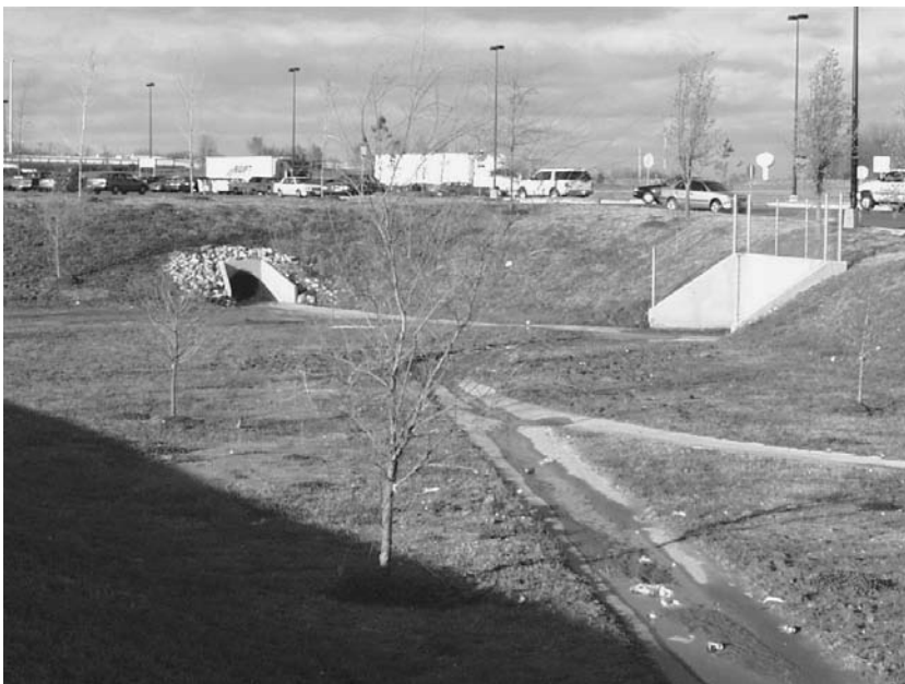
FIGURE 13-19 Extended detention pond picture.
