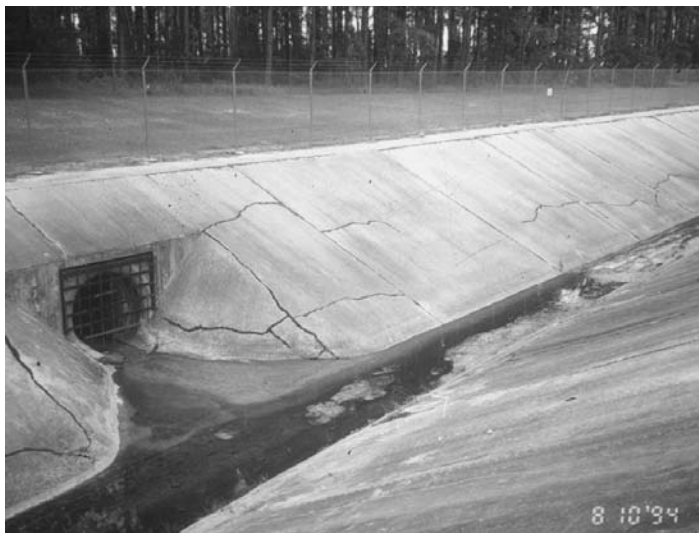
FIGURE 15-15 Dye test results showing illicit connection.
