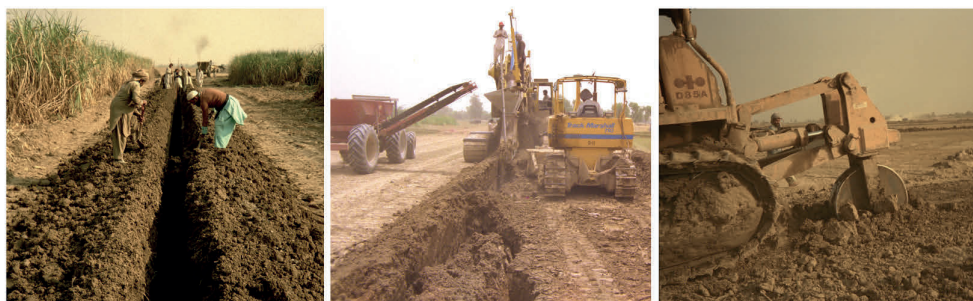
Figure 8.21 Manual blinding, trench back fill with bulldozer to prevent pipe uplift, and method 3a of Figure 8.22 (photographs W.F. Vlotman)
