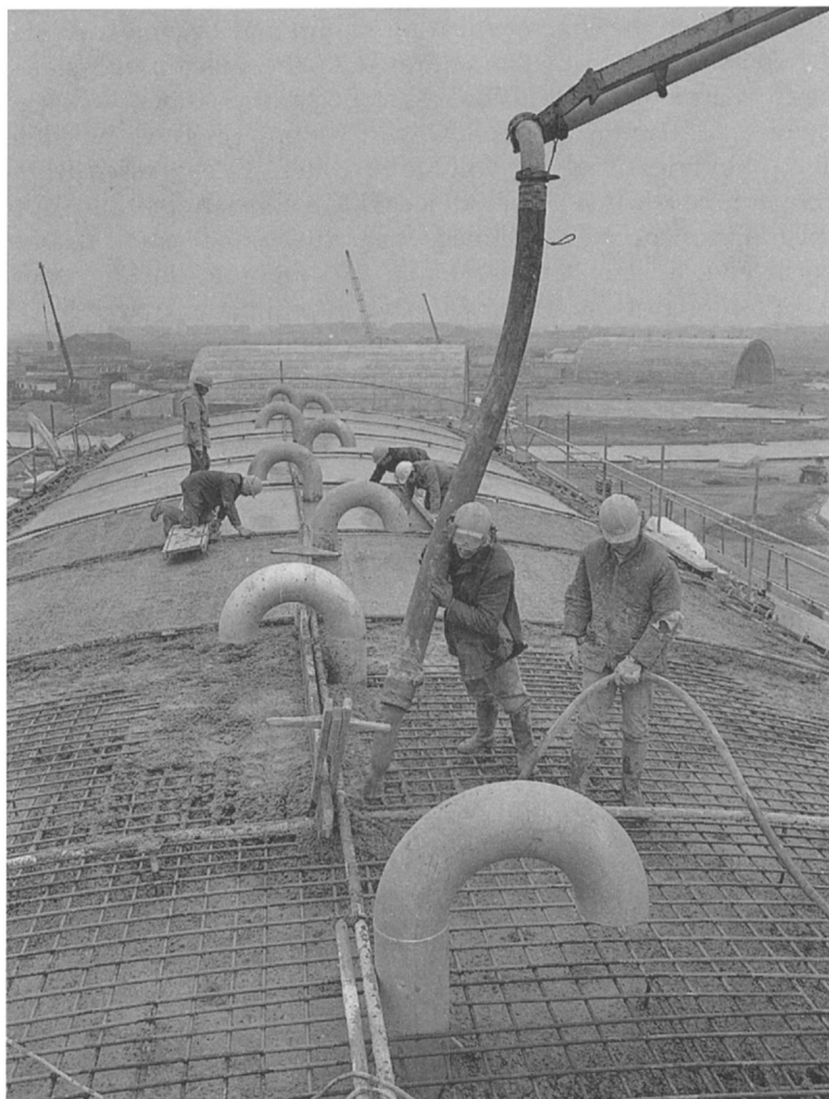
Figure 12.1 Placing concrete by pumping and compaction by use of an internal vibrator. (Photo courtesy of the British Cement Association)
