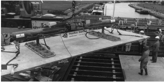
Fig. 7.46 Erecting a UHPC panel (45 mm thick) for the Kaag Bridge in The Netherlands (2003)
