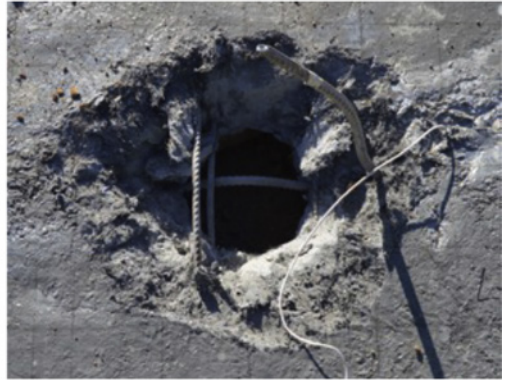
Bottom surface spall diameter 480 mm
