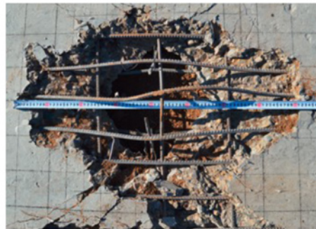
Bottom surface spall diameter 820 mm
