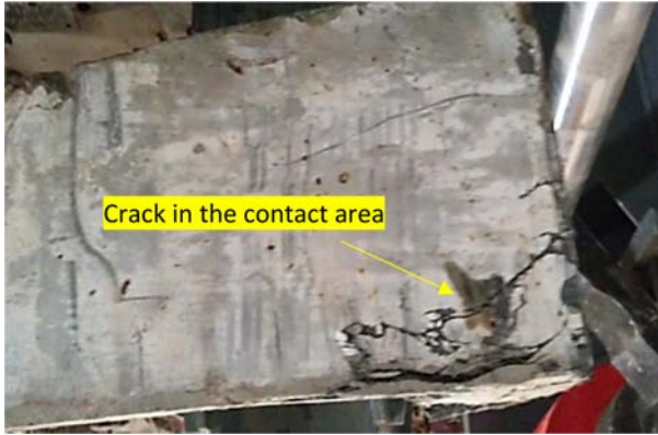
Figure 4.19 Boundary cracks on U2A.
