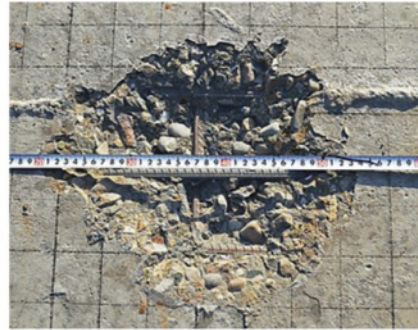
Bottom surface spall area diameter 330 mm
